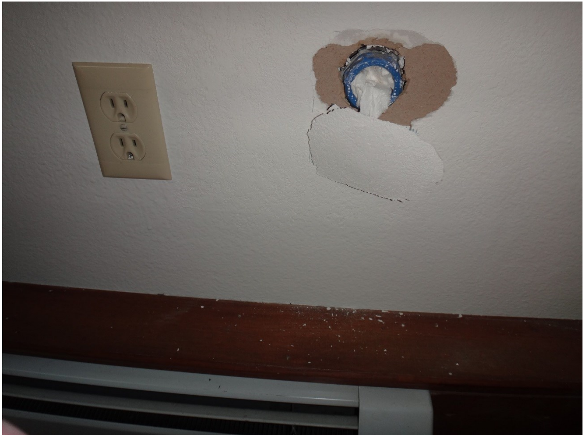
Living Room Damage
