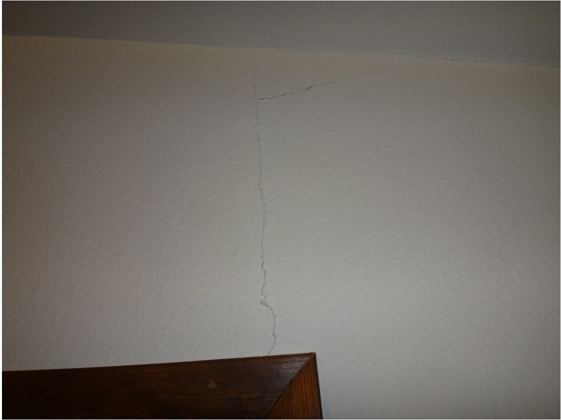
Master Bathroom Crack
