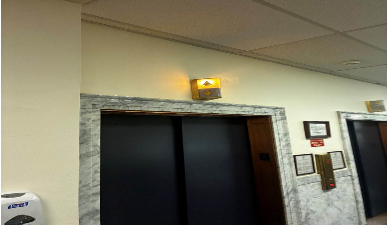
Hallway Car Direction Lanterns (Floors 1-5, up white)
