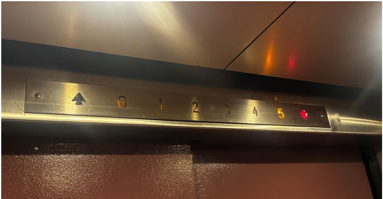
Elevator Car Interior Position Indicators
