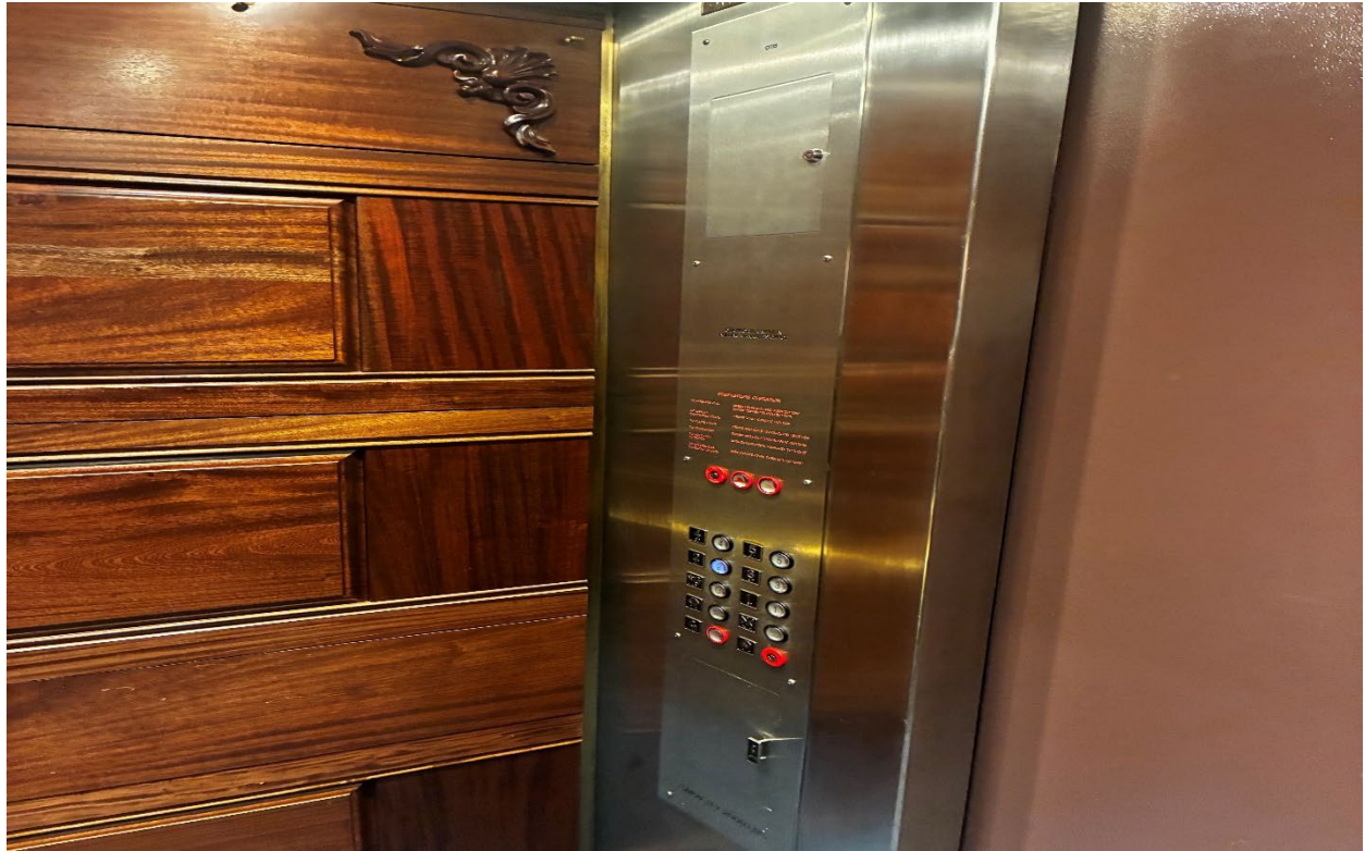
Elevator Car Operating Panel
