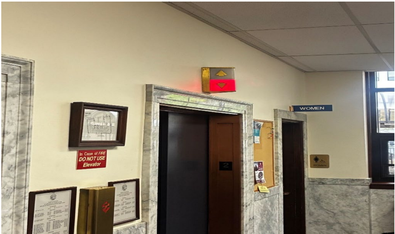
Hallway Car Direction Lanterns (Floors 1-5, down red)
