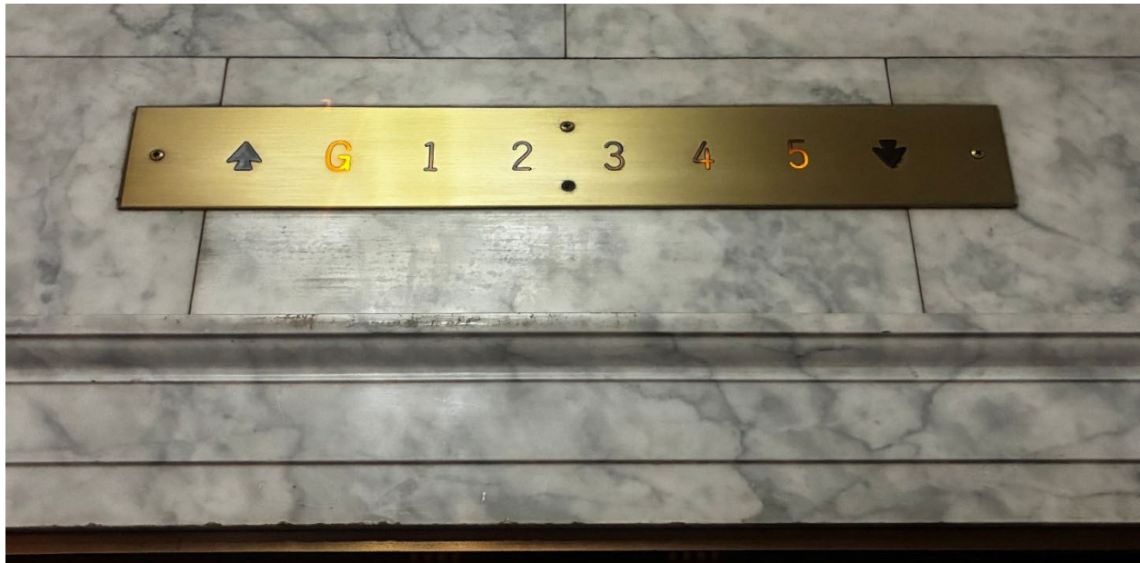
Ground Floor Lobby Position Indicators (Ground Floor Only)
