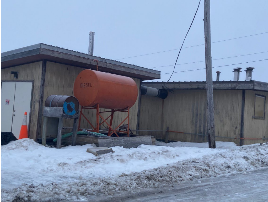
Figure 5 Old Village Fuel Tank
