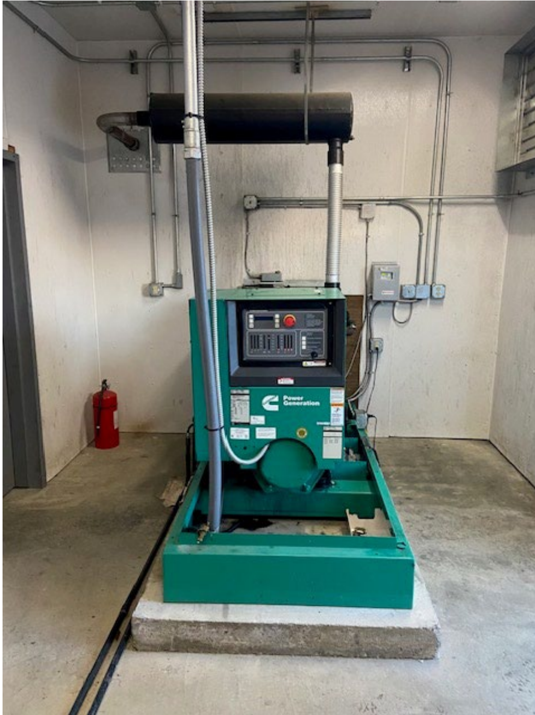
Figure 3 Manokotak Heights Existing Generator
