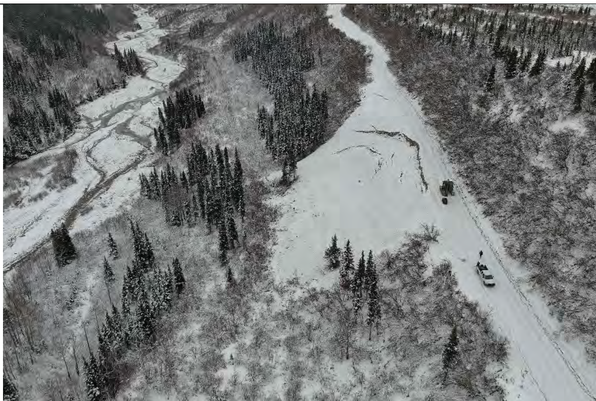
Photo 1. Unstable Slope – Aerial View Southeast
