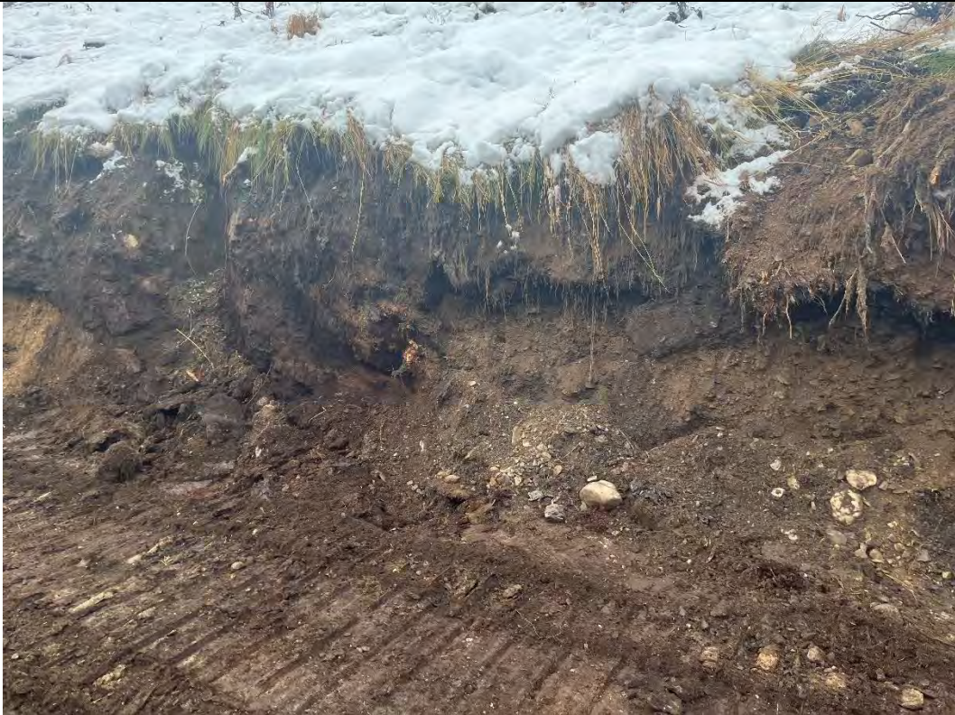
Photo 16. Slope Investigation – Photo #2 of Toe Material Exposed Upslope of Test Boring 2
