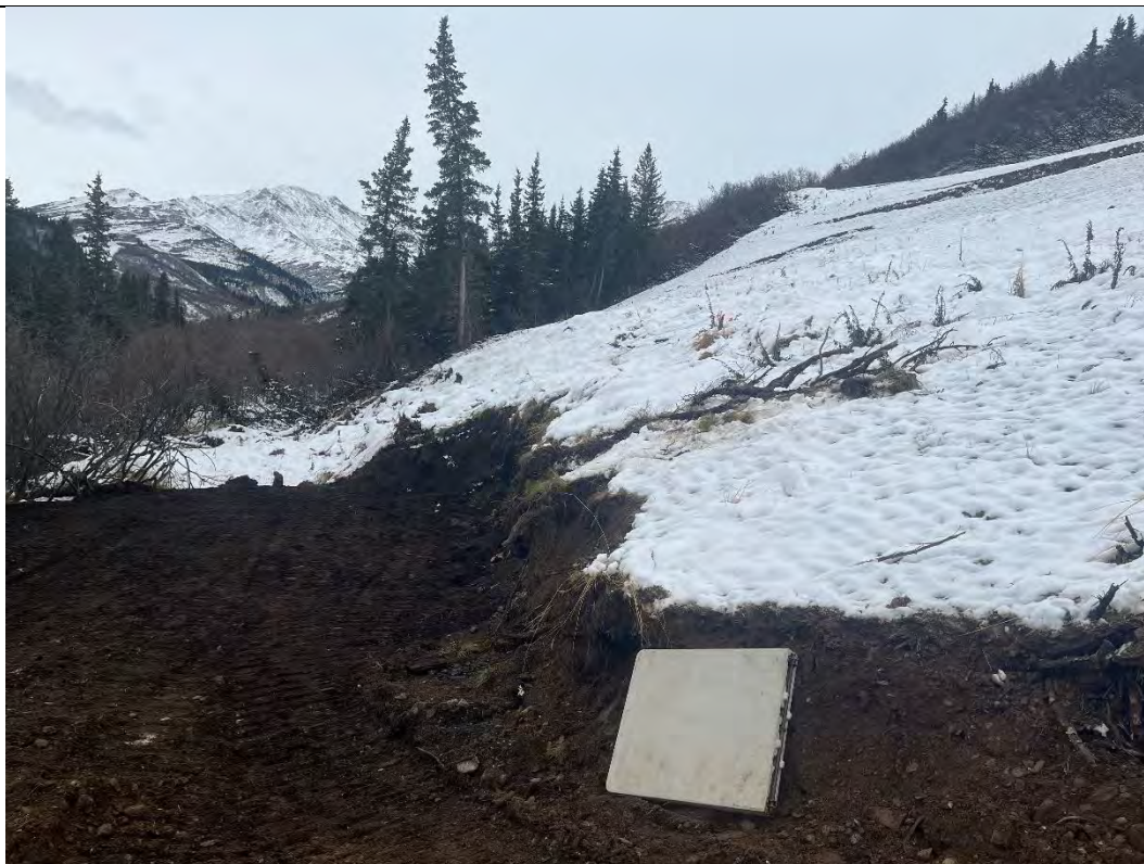
Photo 14. Slope Investigation – View Southeast at Toe of Fill and Leaning Trees
