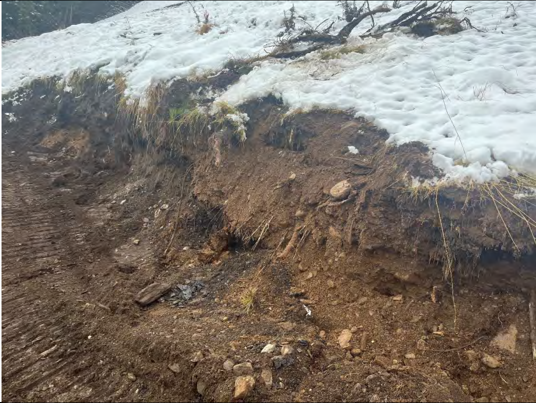
Photo 15. Slope Investigation – Photo #1 of Toe Material Exposed Upslope of Test Boring 2
