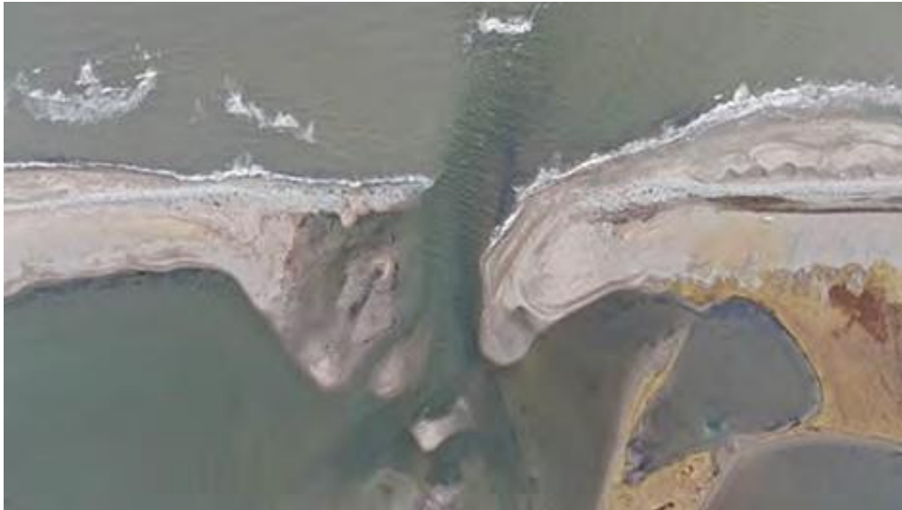
Figure 11. Oceanic breach of highway in Nome
