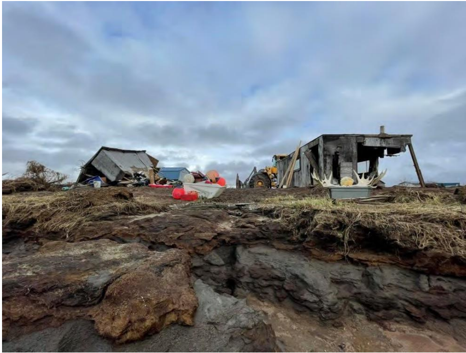
Figure 13. Fish Camp in Nome Sustains Damages
