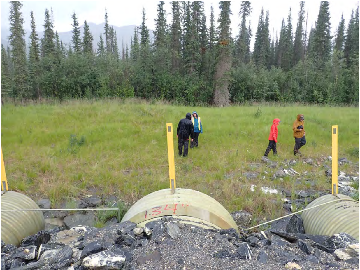
Figure 7. Looking upstream from MP 214.7 structure – existing berm is preventing flow into crossing. Historic channel appears to have migrated north, likely due to this berm.
