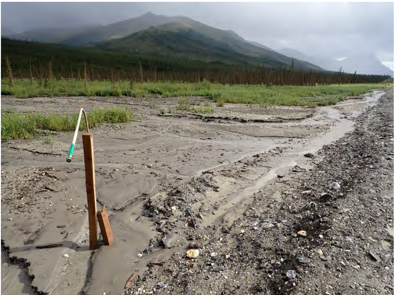
Figure 4. Sediment deposition on east shoulder of Dalton Highway results in clogged culverts and road overflow.
