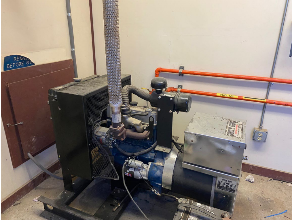
Figure 6 Old Village Existing Generator
