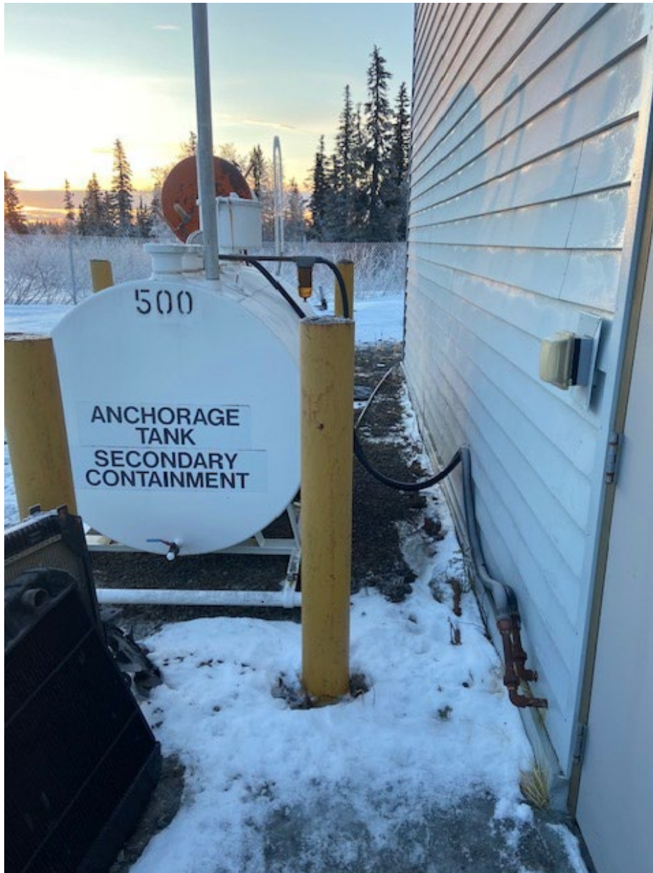
Figure 2 Manokotak Heights Fuel Tank
