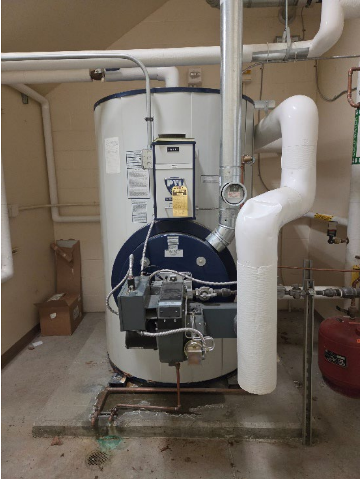
Figure 2. Existing Water Heater
