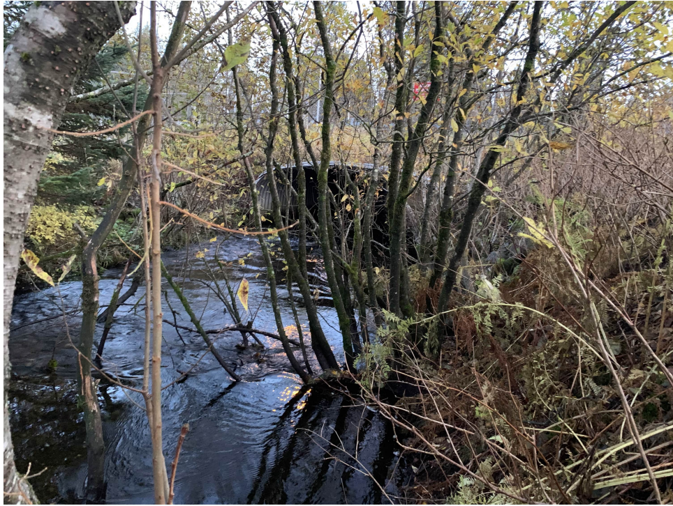
Photo 13: Yakutat Airport stream culvert under DOT property near proposed waterline crossing, facing east.
