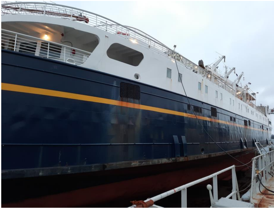
Figure 4 Corroded louvers on port side
