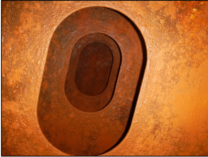
Photo 14: No. 3 Center Line DB Ballast
