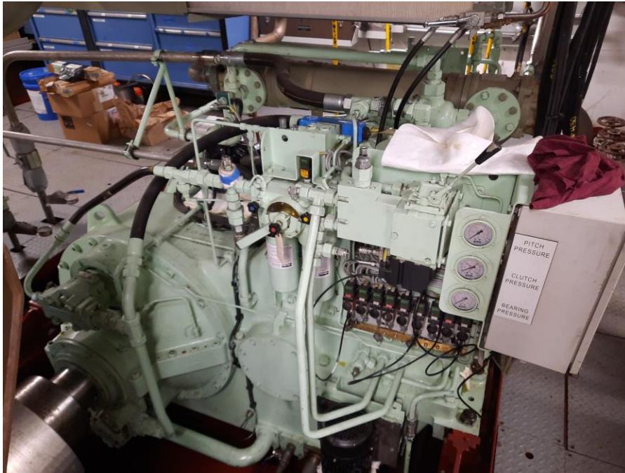
Figure 40 Starboard reduction gear
