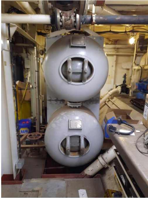
Figure 33 Corroded inspection hatch covers
