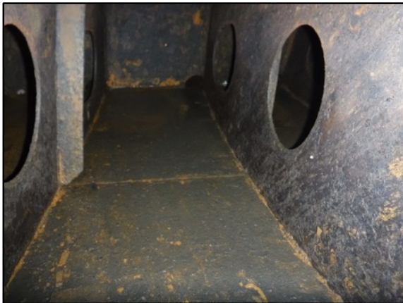
Photo 20: No. 4 Port Wing Ballast
