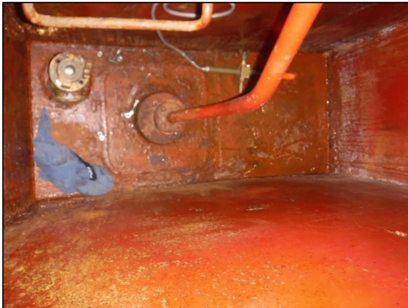
Photo 23: Existing Coating System in No. 4 Transducer Void
