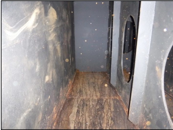
Photo 29: Minor Corrosion on Welds on Deck of No. 5 Double Bottom
