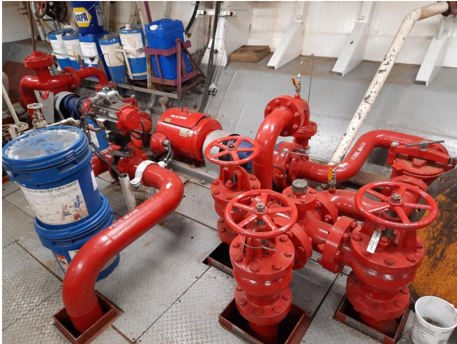
Figure 36 Firemain piping and #2 fire pump located in Main Engine Room
