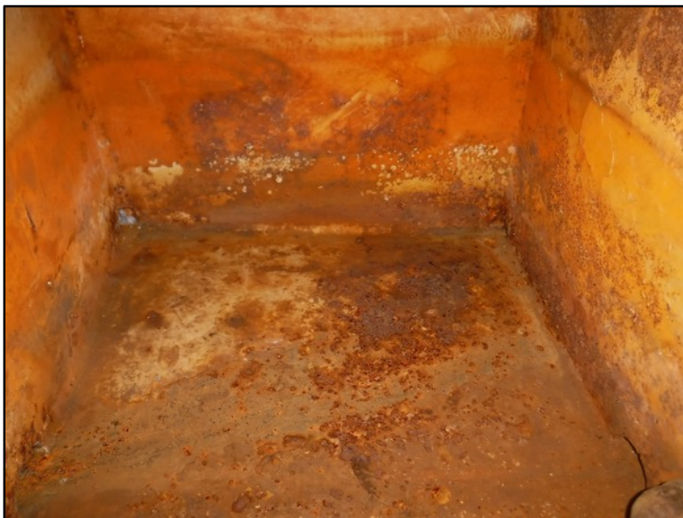
Photo 45: Corrosion on Deck of Cross Flood
