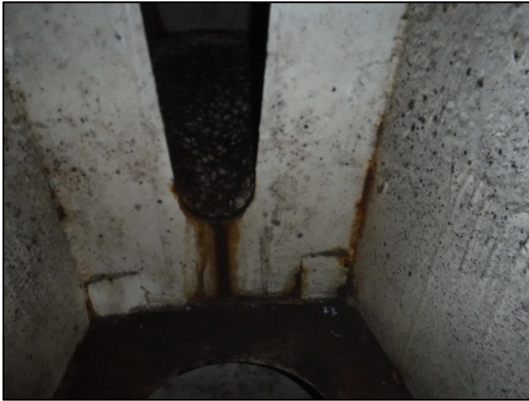
Photo 2: Minor Corrosion on Skip Welds & Sharp Edges in Lower Forward Section
