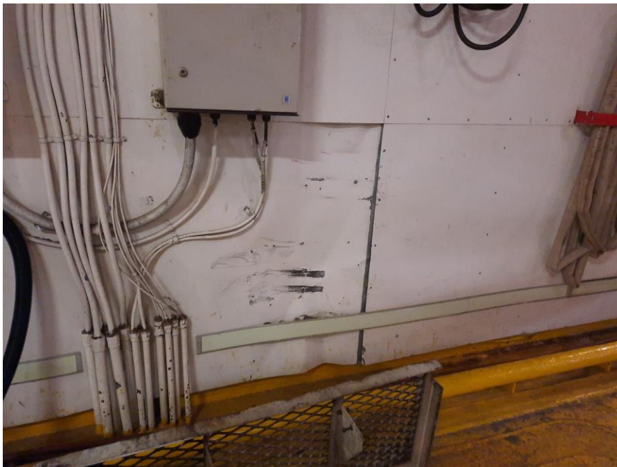
Figure 10 Dented insulation on center island
