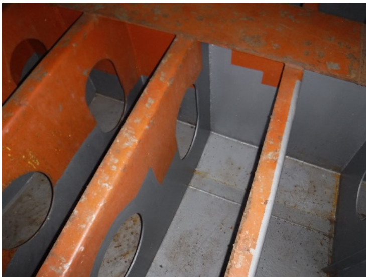
Photo 43: No. 10 Center Line Void
