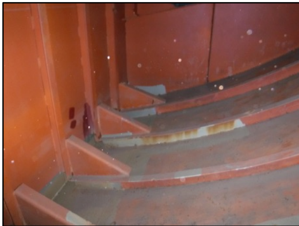
Photo 38: No. 10 Port Void
