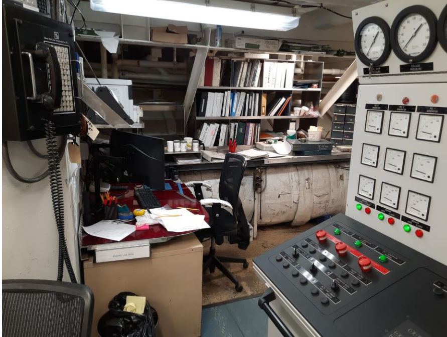
Figure 27 EOS with adjacent Engine Room ventilation supply ducting
