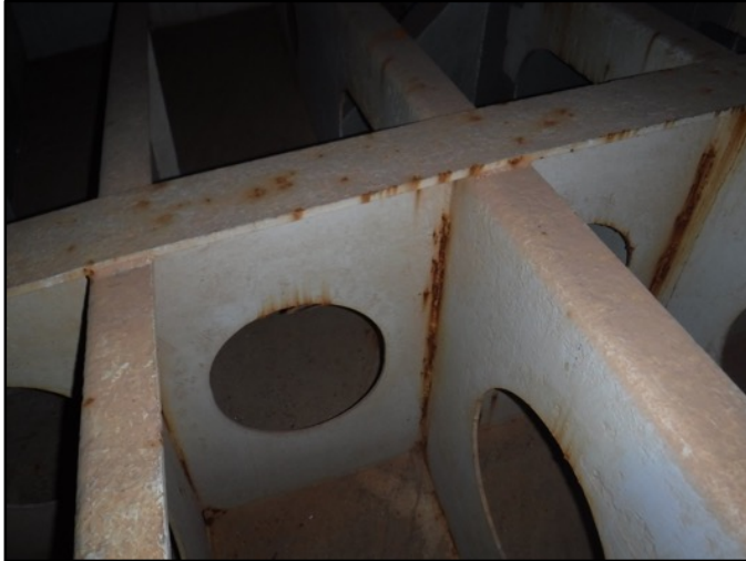
Photo 54: Minor Corrosion on Welds in Lower Section
