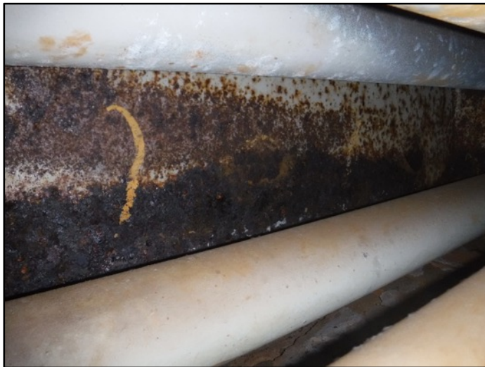
Photo 18: Corrosion on Sides of Pipe Alley
