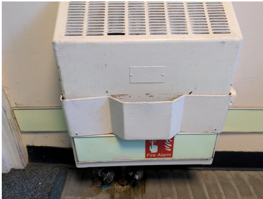
Figure 14 Corrosion around radiator deck penetration in aft Boat Deck Foyer
