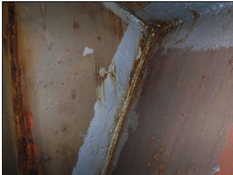
Photo 7: Minor Corrosion on Welds in Upper Section
