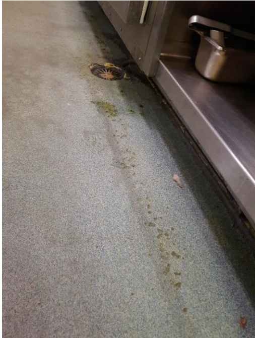
Figure 23 Worn and flaking deck covering in Galley
