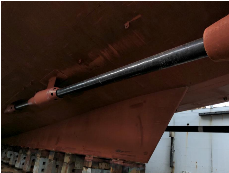
Figure 42 Port propeller shaft
