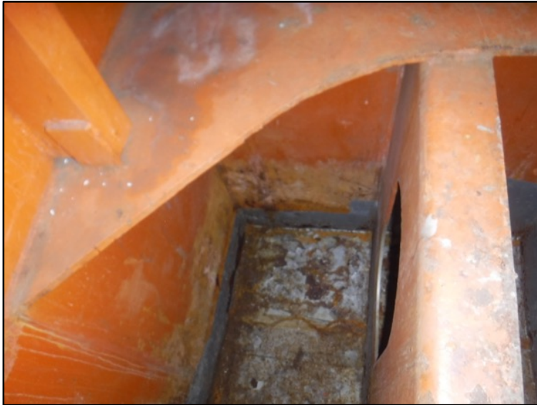
Photo 44: Coating Delamination Spots & Corrosion on Deck in Middle Section
