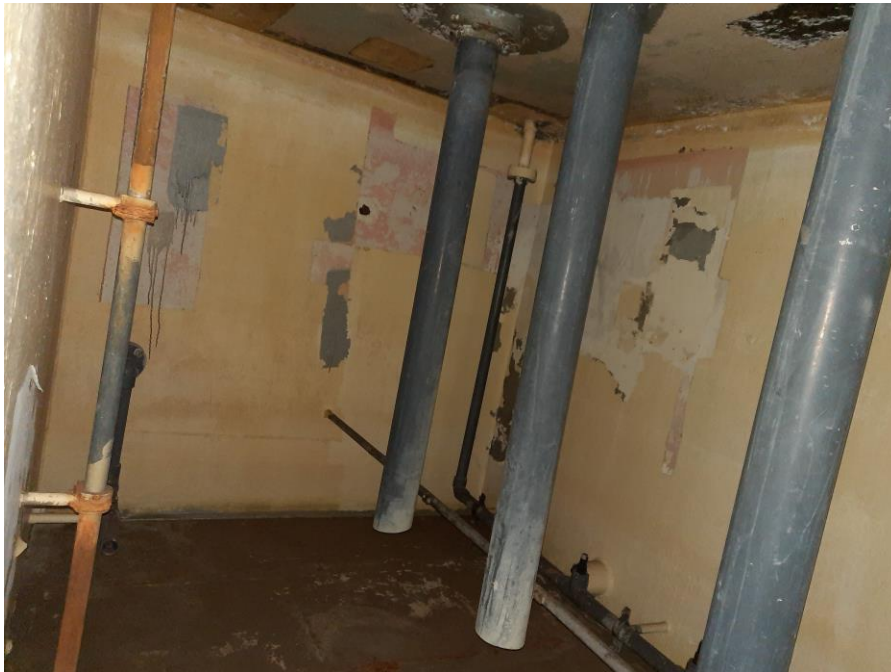
Figure 45 V2 tank suction lines
