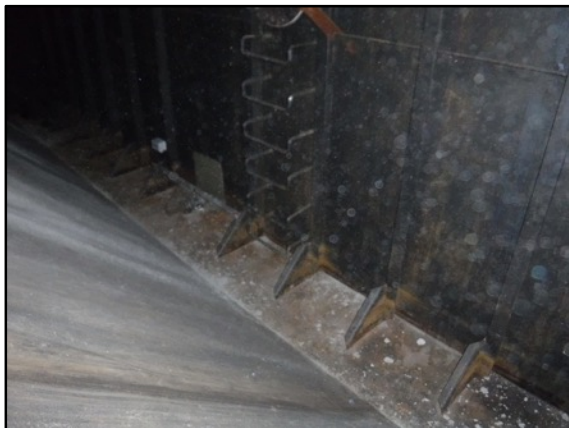
Photo 24: No. 5 Port Void
