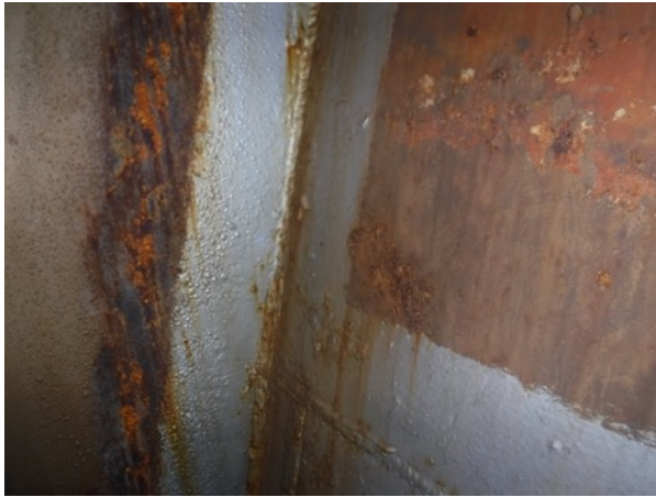
Photo 5: Corrosion on Forward Bulkhead
