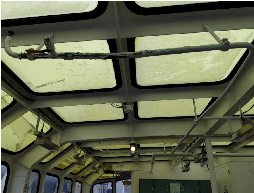
Figure 35 Damaged coatings and corrosion on piping in Solarium overhead
