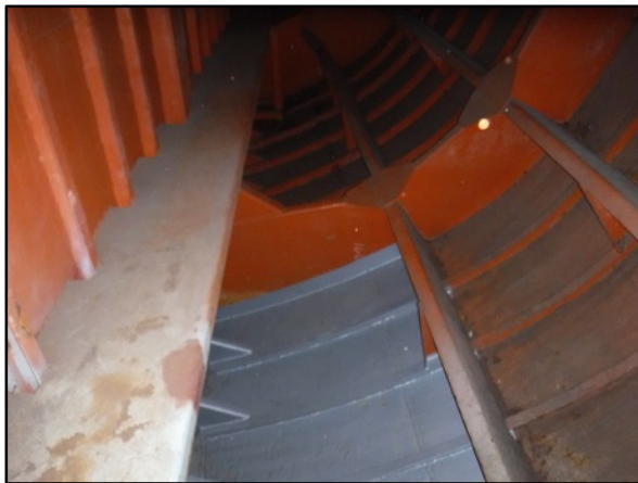
Photo 46: No. 11 Port Void
