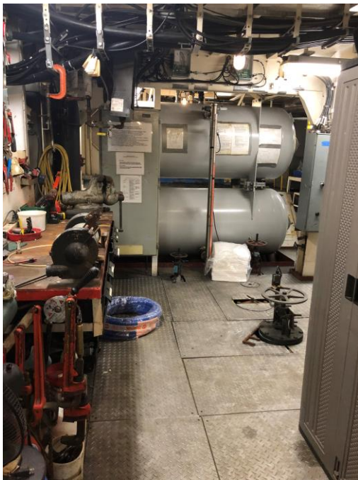
Figure 34 Accommodation sprinkler system pressure tanks
