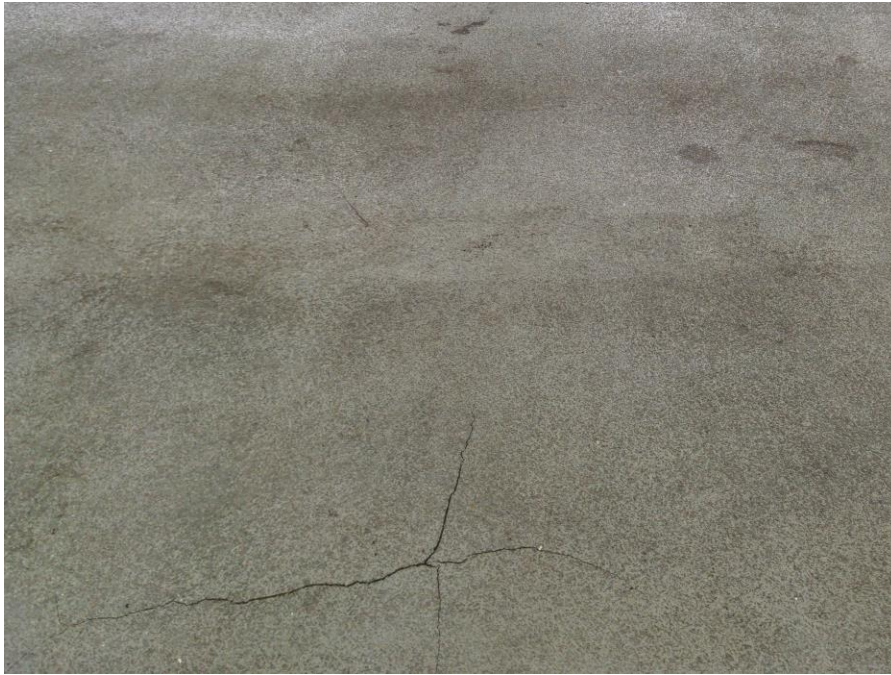
Figure 18 Cracks in Solarium deck covering
