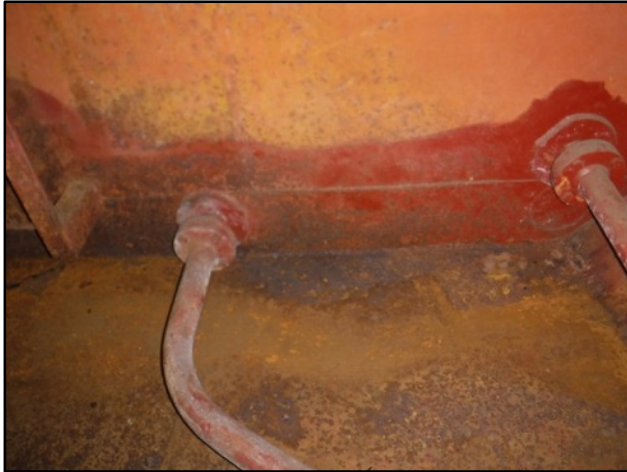
Photo 10: Corrosion on Deck near Forward Bulkhead
