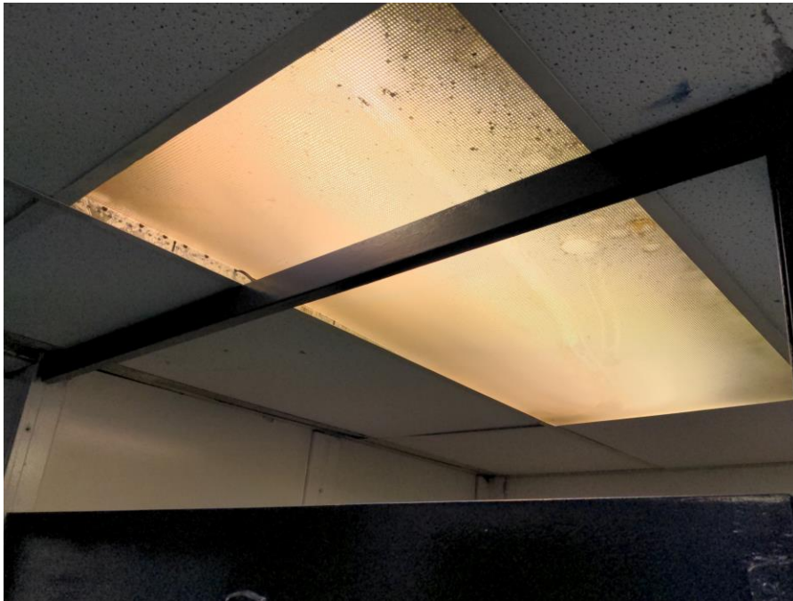
Figure 17 Aged overhead and lighting diffuser in Boat Deck forward Women's Head
