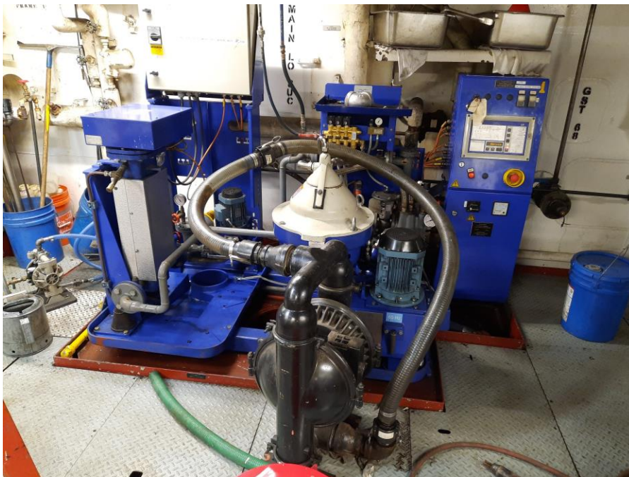
Figure 48 Lube oil purifier
