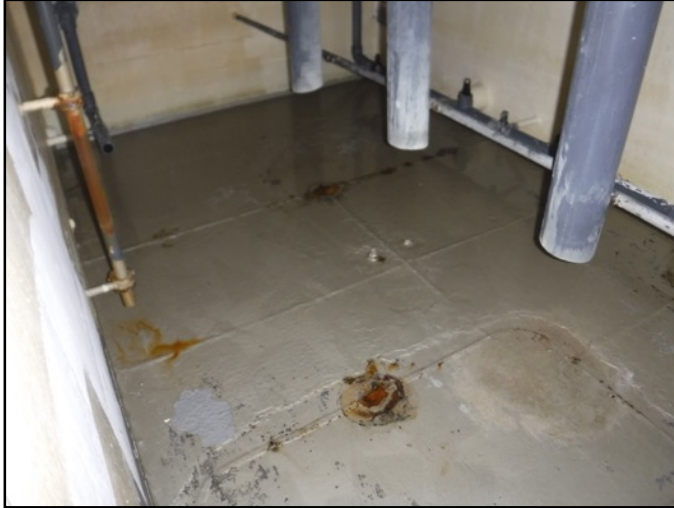
Photo 31: Delamination Spots on Deck of V-2 Sewage Tank
