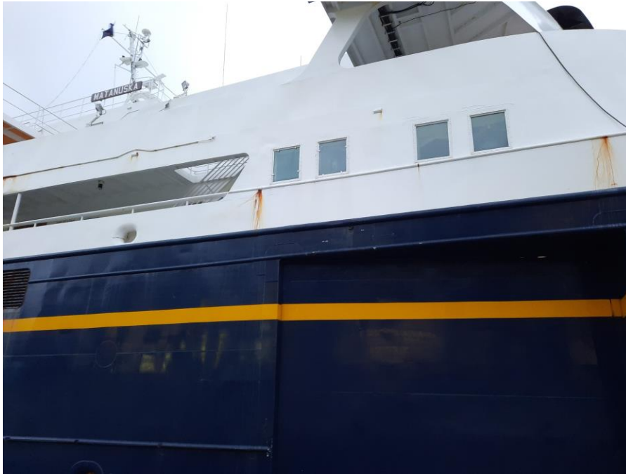
Figure 7 Rust bleeds on superstructure
