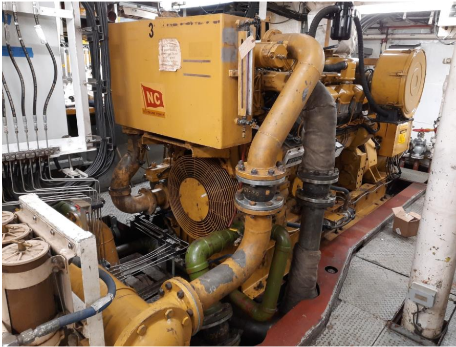
Figure 38 Ship service diesel generator
