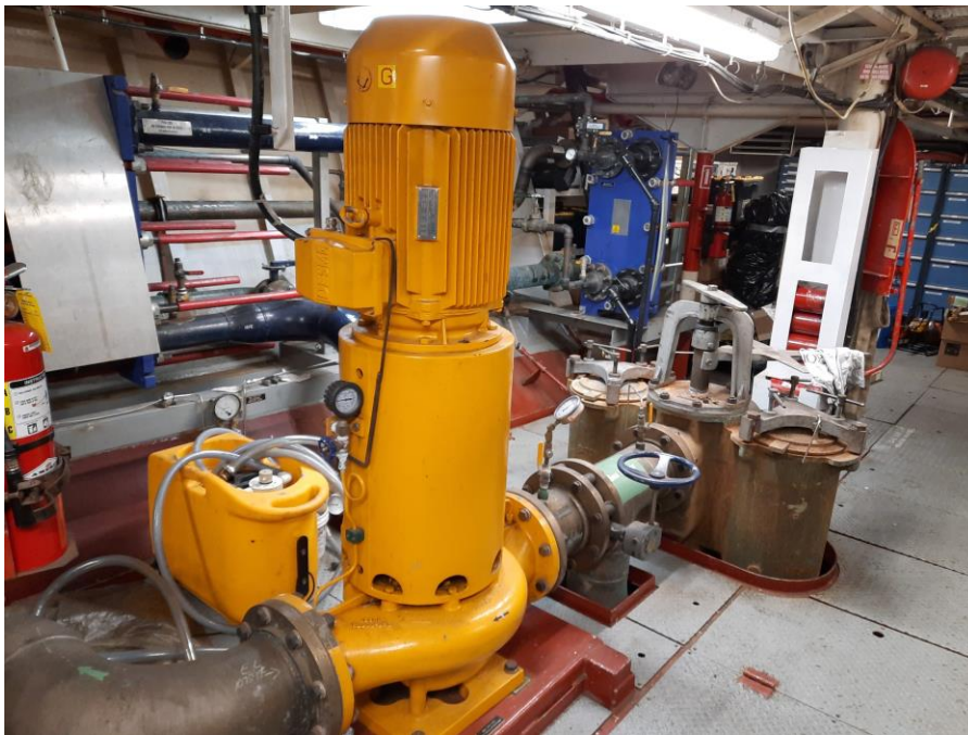
Figure 47 Seawater pump and piping
