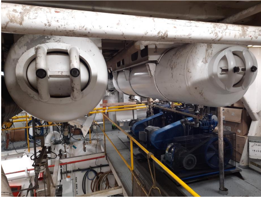
Figure 49 Compressed air receiver tanks
