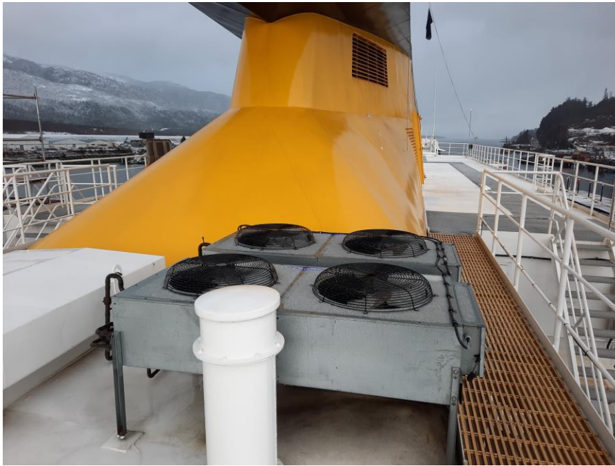
Figure 32 Exhaust stack seen from aft
