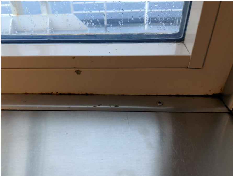
Figure 15 Corrosion on bottom edge of window in Boat Deck passageway
