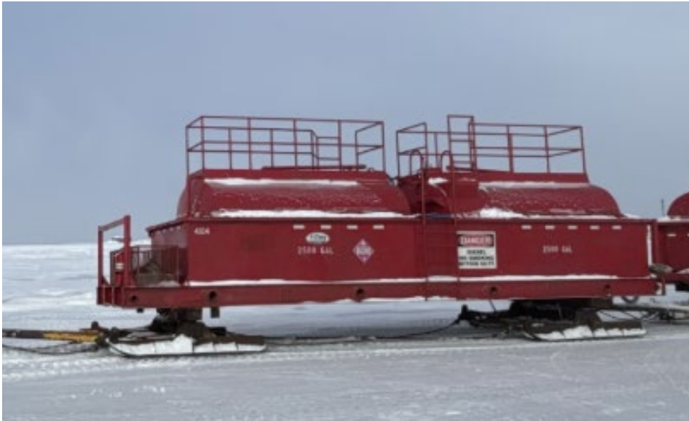
Figure 12: Mobile diesel fuel storage sleigh with two 2,500-gallon double walled tanks.
