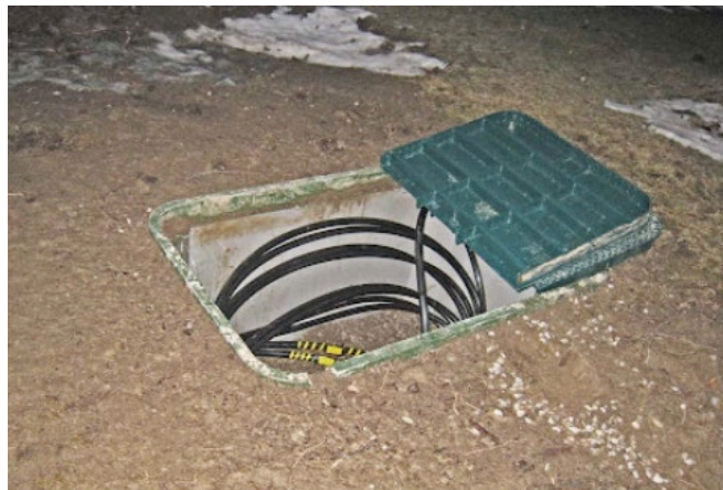
Figure 25: Cable Vault with extra FOC cable
