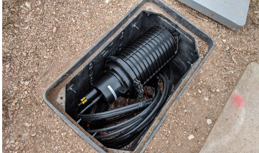
Figure 24: Handhole with FOC and splice case
