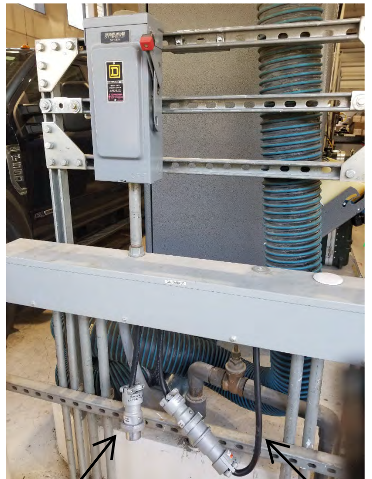
Old Compressor/Pressure Washer Layout, Note 2 Separate Hook Ups
