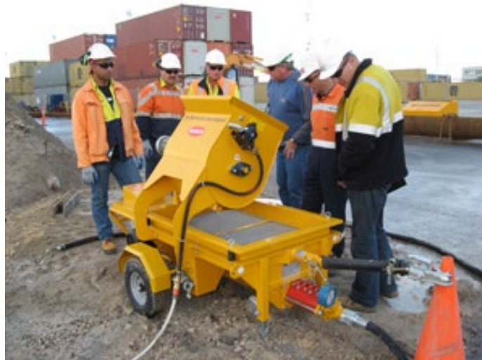
Figure 15-1 Grout Mixing Equipment
