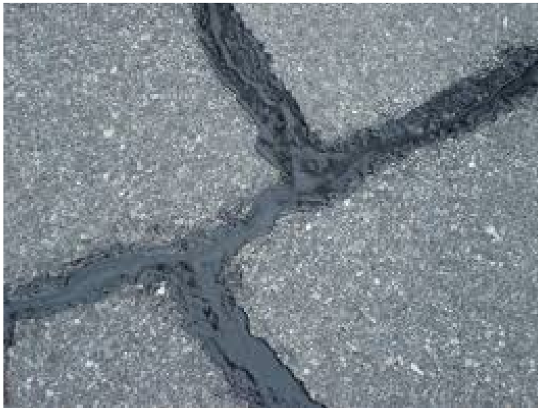
Figure 9-12 Crack After Sealing
