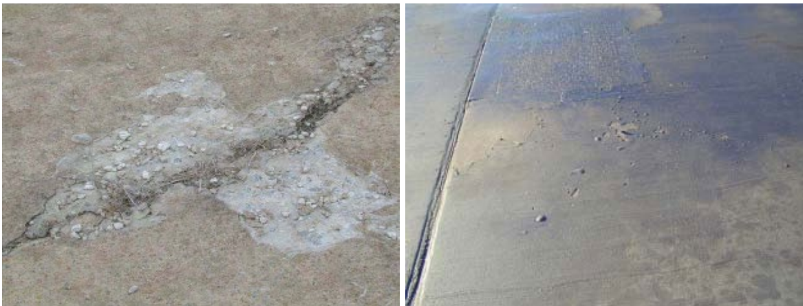
Spalling and Scaling
