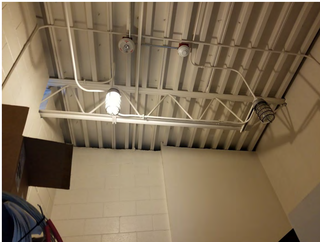
Storage Room Interior Lighting Photo
