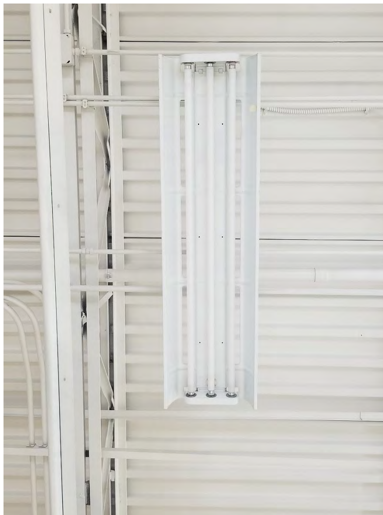
North Bay Interior Lighting Fixture Photo
