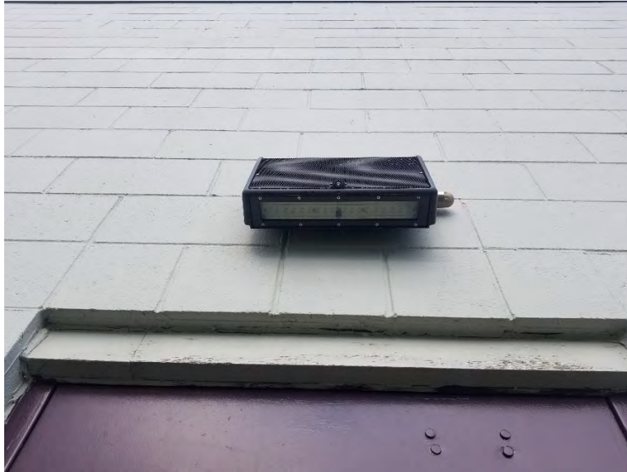
Exterior Lighting Fixture #3 Photo
