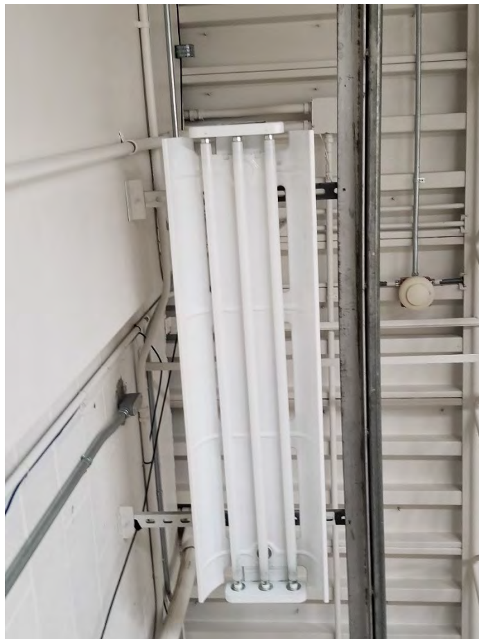
South Bay Interior Lighting Fixture Photo
