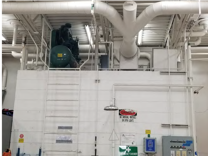
North Bay Single Light Fixtures Photo (Above Mech Room By Compressor)
