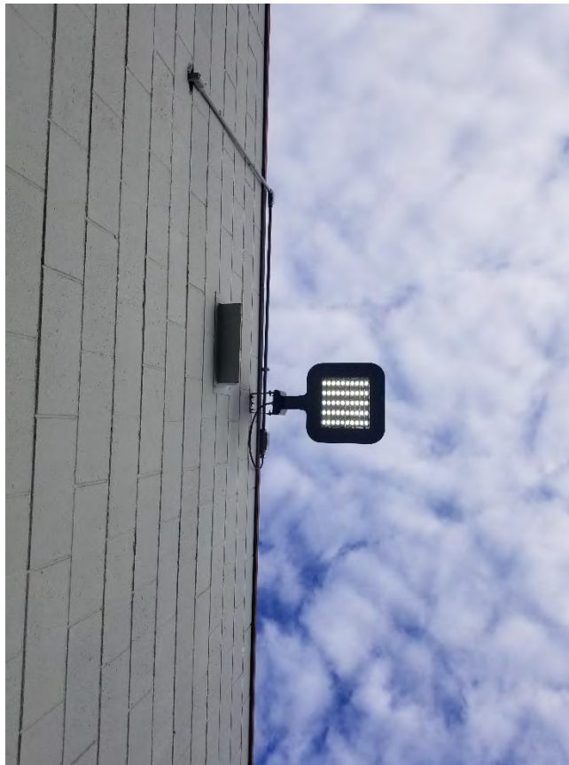
Exterior Lighting Fixture #2 Photo
