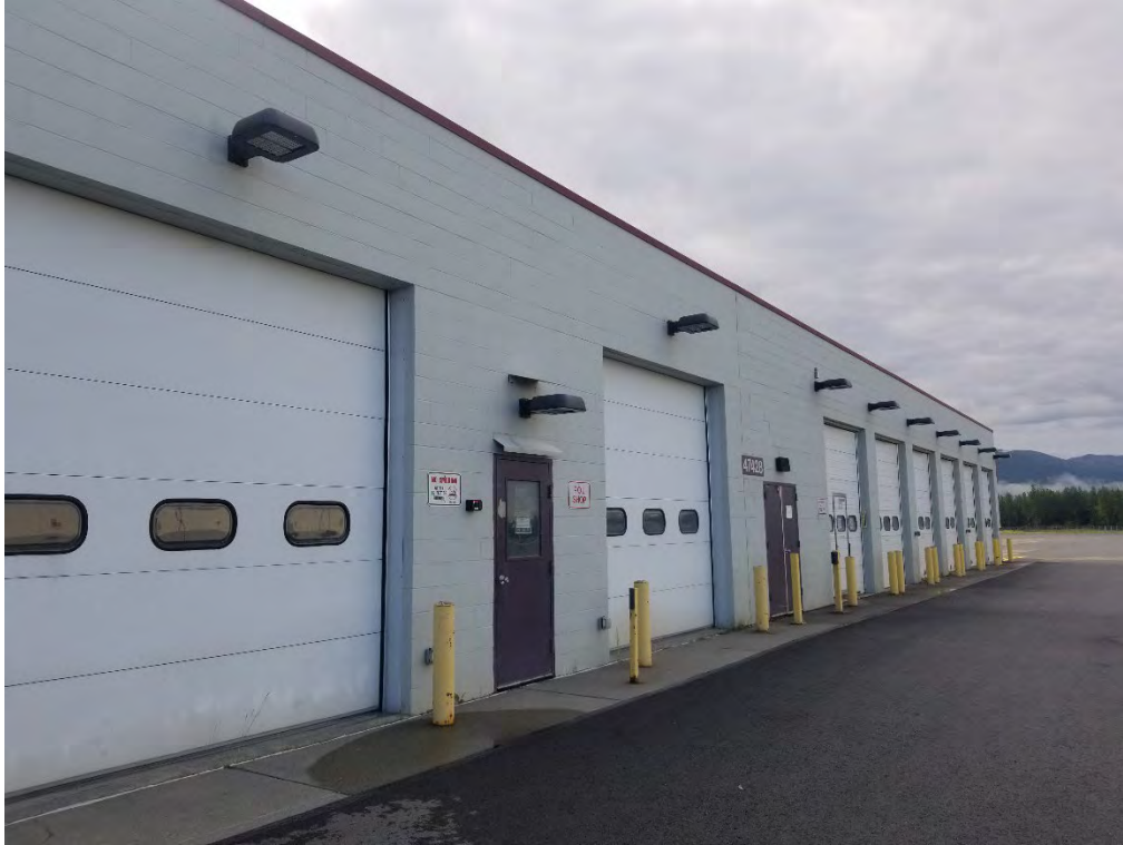
Exterior Lighting Photo (West Side)
