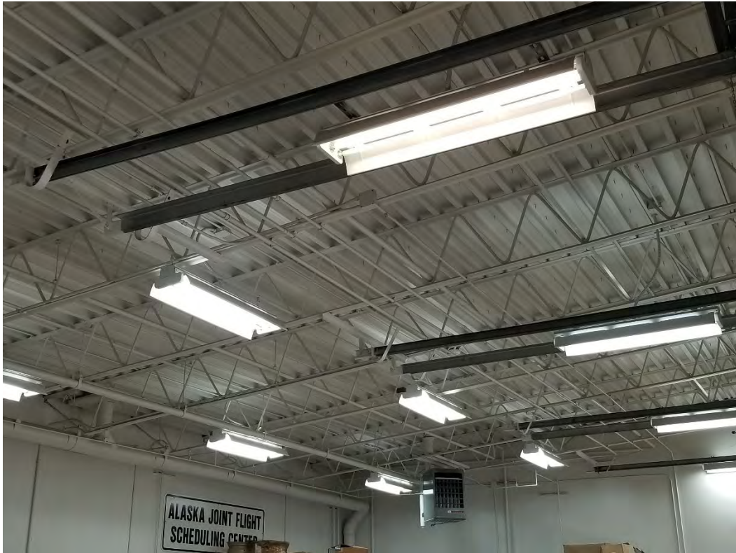
South Bay Interior Lighting Photo
