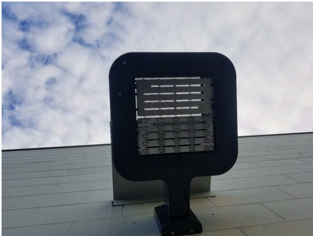
Exterior Lighting Fixture #1 Photo
