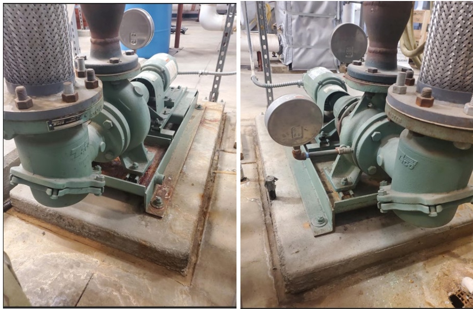
Figure 5 & 6. Rear View, Boiler Water Circulating Pumps on Slab Bolted Down
