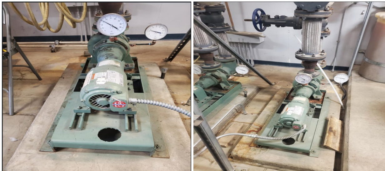
Figure 1 & 2. Pumps Front View, Motor, Gauges, and Electrical Components
