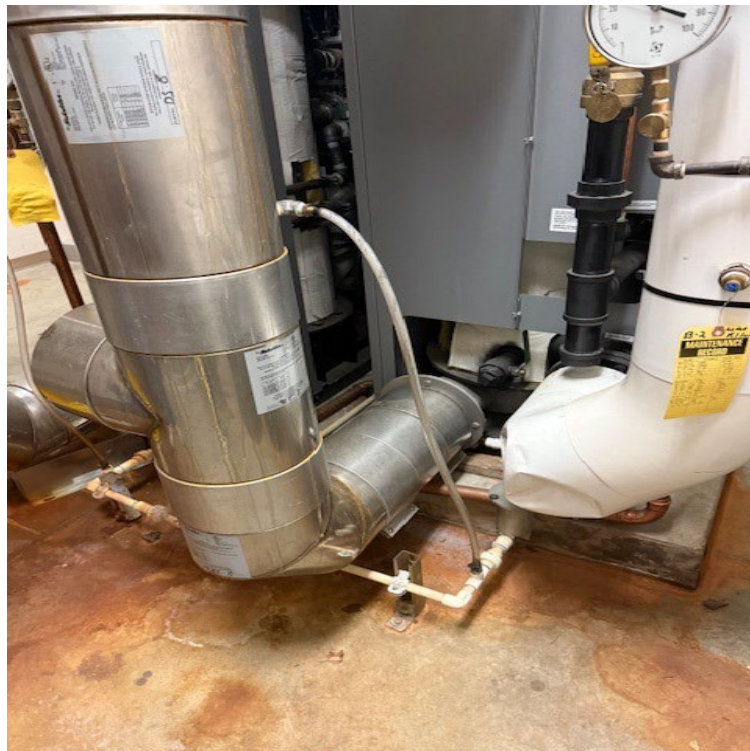
Figure 2. Vent's flange connection to boiler
