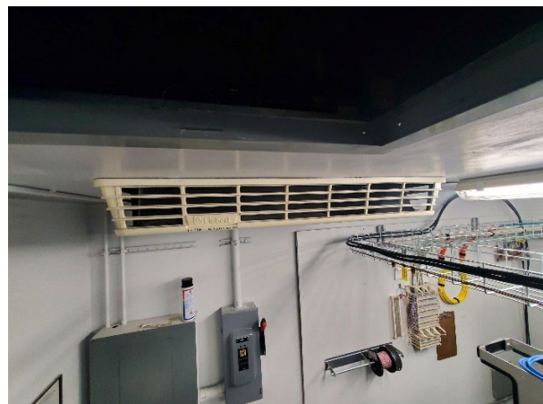
Figure 2. A/C Unit Below Ceiling Tile
