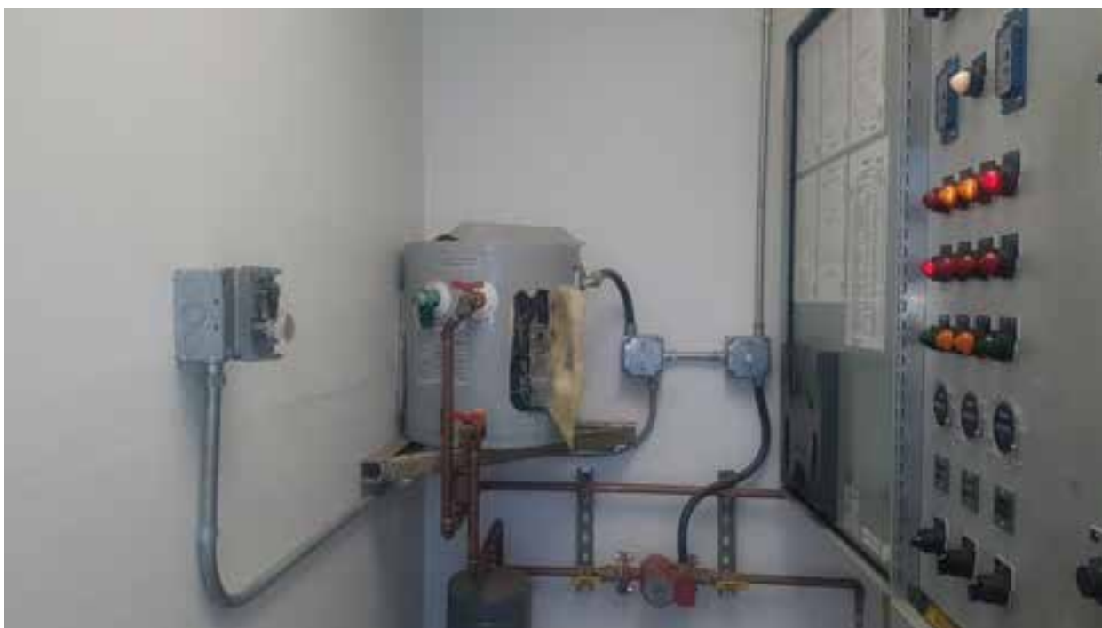
Figure 42- Covenant lift station - Broken water/glycol heater for slab, control panel on right
