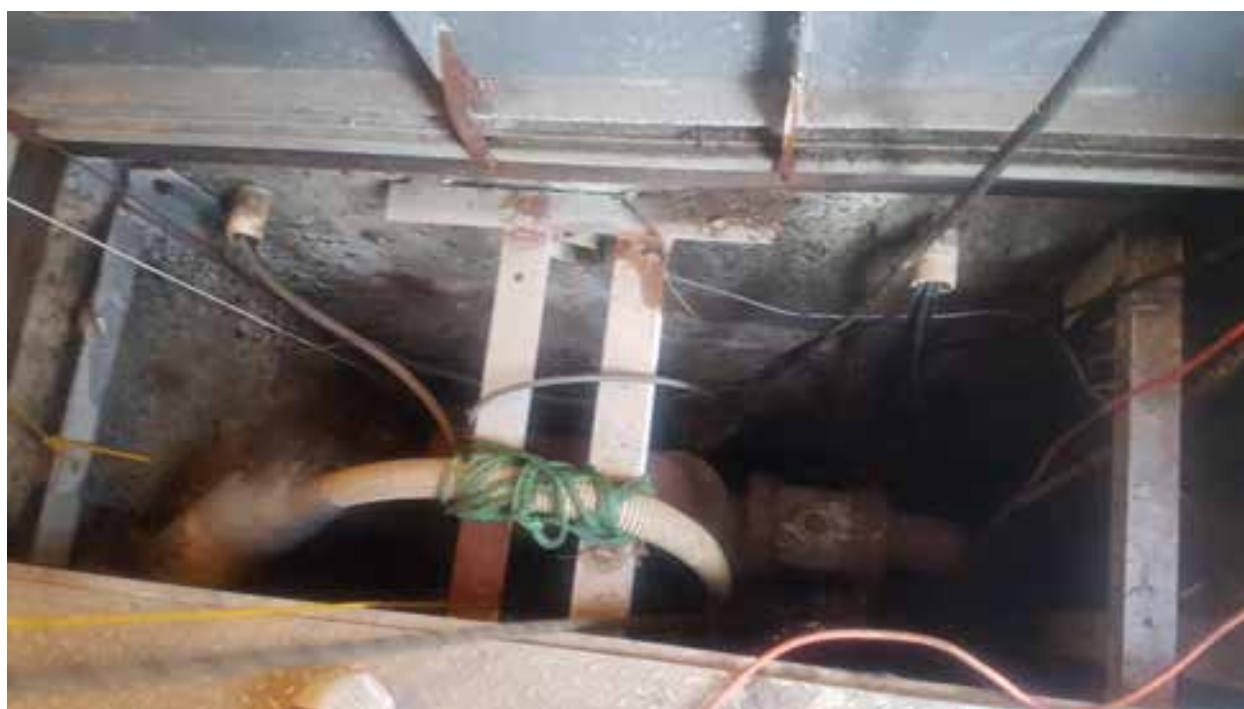
Figure 28 - FAA Lift station - Temporary 110v pump and hose connection with temp 110v float switches.
