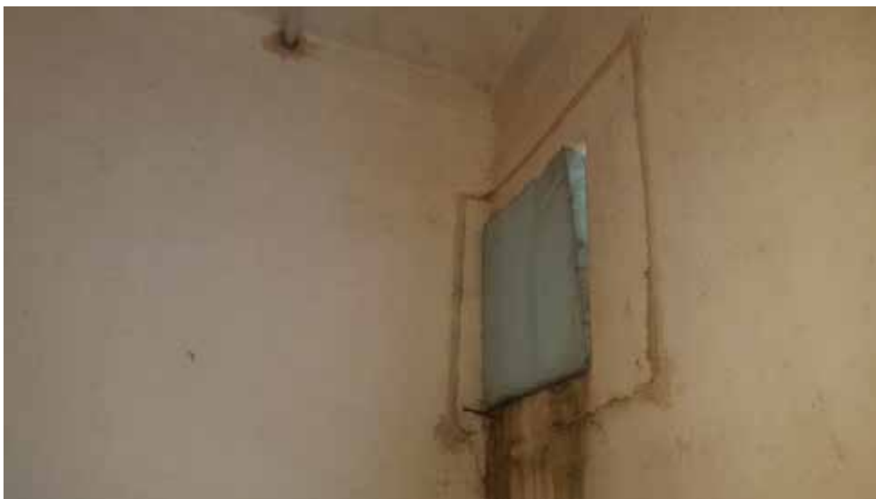
Figure 3140 - Covenant Lift Station - Interior "Passive" ventilation
