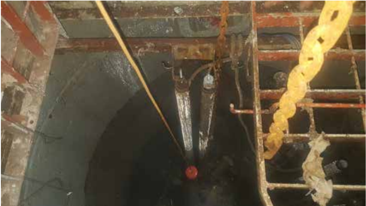
Figure 37 - Covenant Lift Station - Rail mounting brackets have been jacking up. They buckle when operators try to pull pump. Operators would rather "jog" the pumps over and over instead of risking losing the support bracing.
