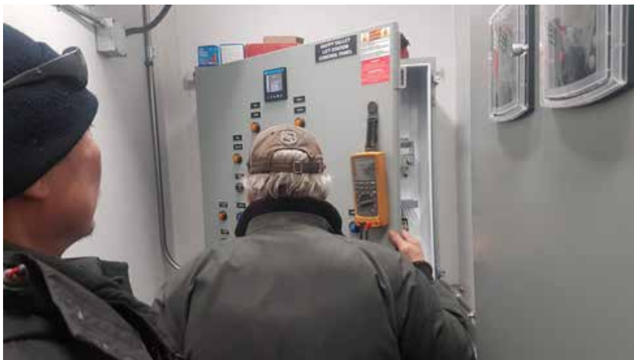
Figure 54 - Buck showing Dwayne how the lift station panel works.
