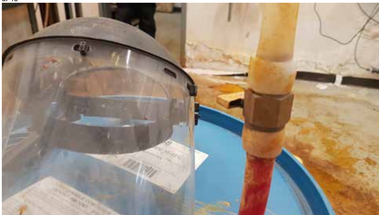
Figure 19 Neat FeCl transfer pump is broken. Crew used temporary valve which corroded away within 20 to 30 minutes.
