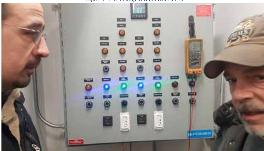
Figure 2 - Karl Hulse (Left) and Buck Amadon (Right) using Fluke meter to simulate transducer and show well control panel functionality.
