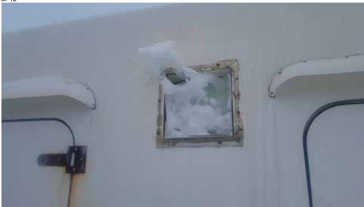
Figure 41 - Covenant Lift Station - Outside shot of "interior passive ventilation"
