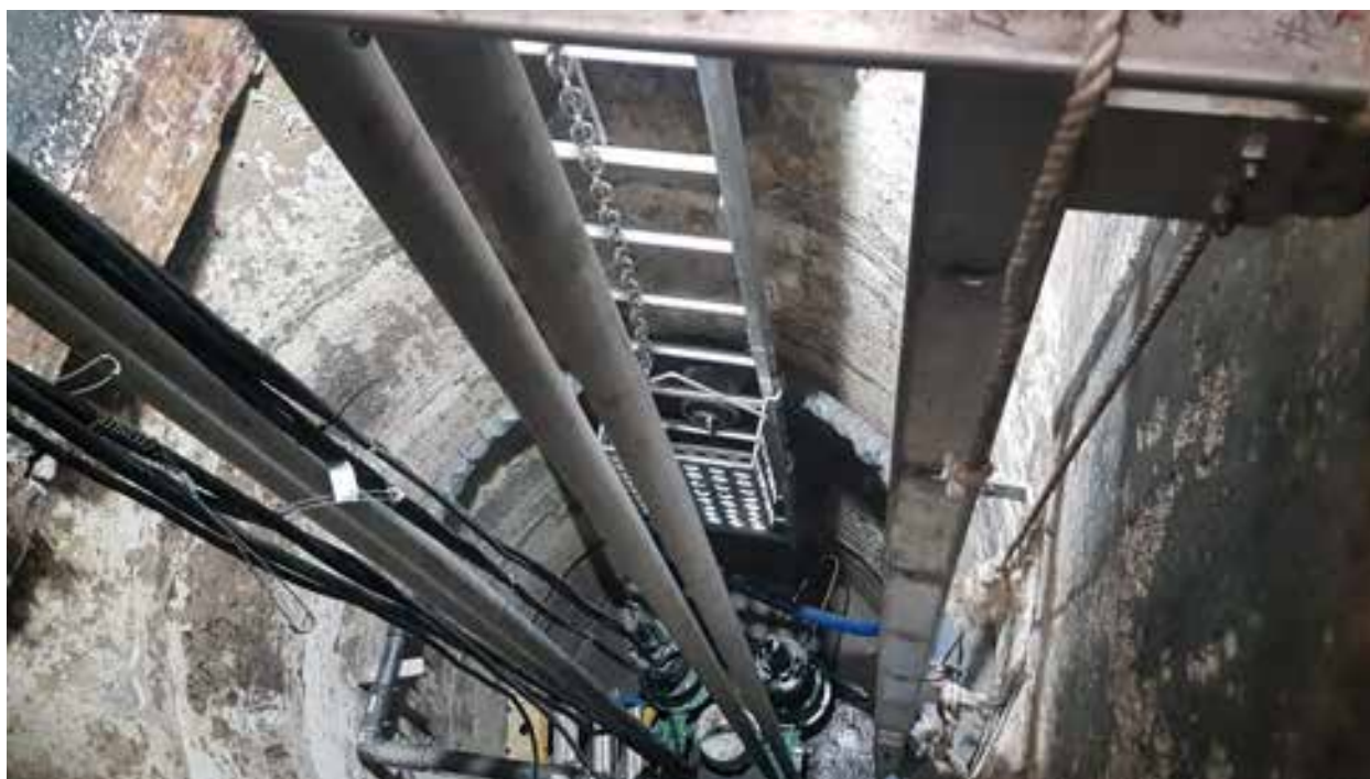
Figure 334 - HVLS Looking down well after all pump cables and power have been set. Temporary connection hose is routed around the ladder (grey)
