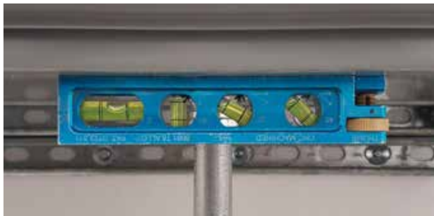
Figure 3- Well Pump Control Panel Level
