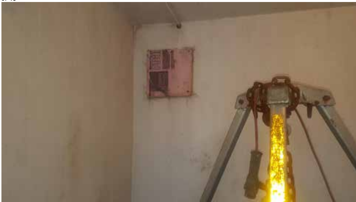
Figure 39 - Covenant Lift Station - Vent Package Removed. Boarded Up
