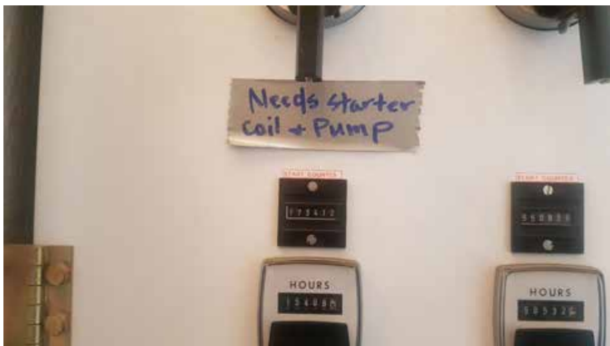
Figure 30 - Terminal Lift Station Control Panel - Recommended parts for functionality
