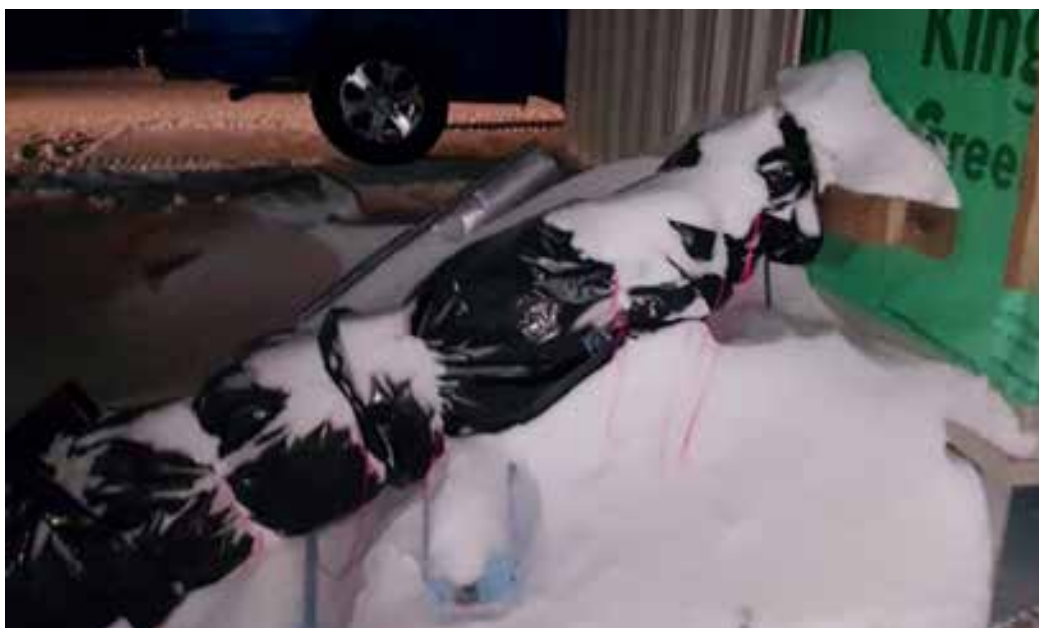
Figure 11 - Exterior connection of temporary bypass to building
