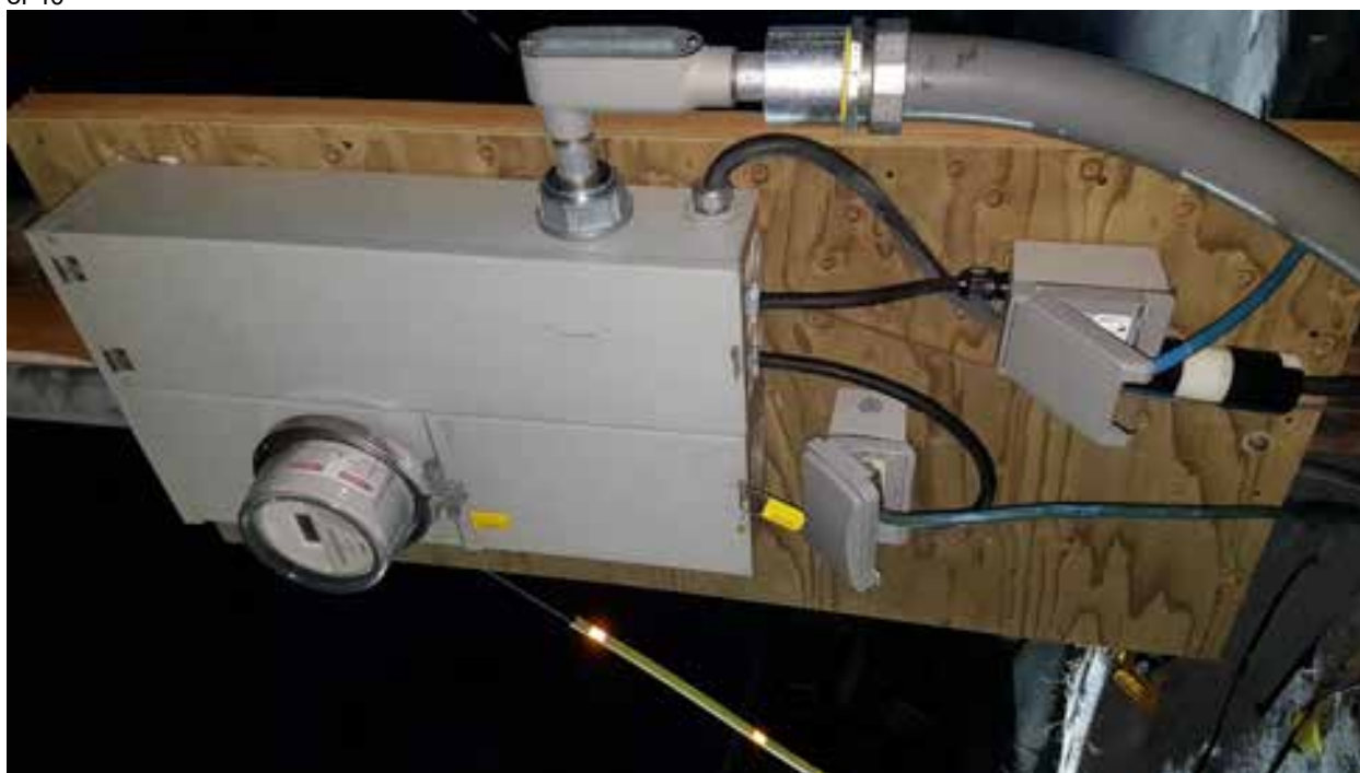
Figure 13 - 125 amp meter base needing replacement with 200 amp meter base
