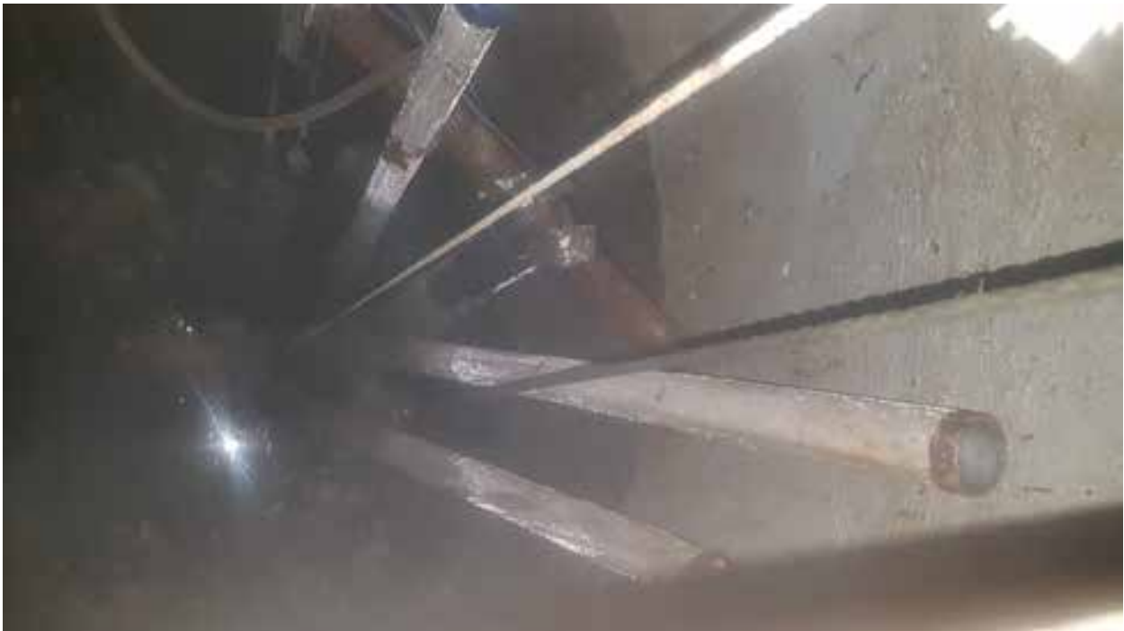
Figure 3830 - "Support" bar that operators must stand on to re-align pump rails when they dislodge, as well as re-wire a new pump when one fails. Bar is angled behind the set of functioning pump rails (left) to the concrete wetwell behind the shadow of the chain.
