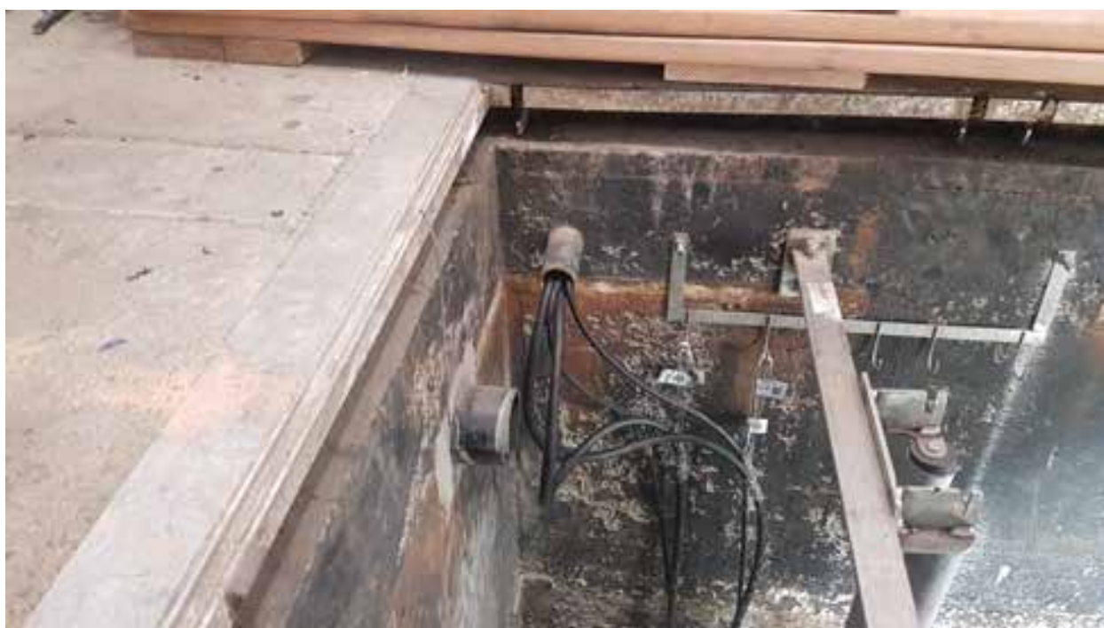
Figure 52 - HVLS with pump power cables running through conduit - suggest future orders for pump power cables to longer than necessary.
