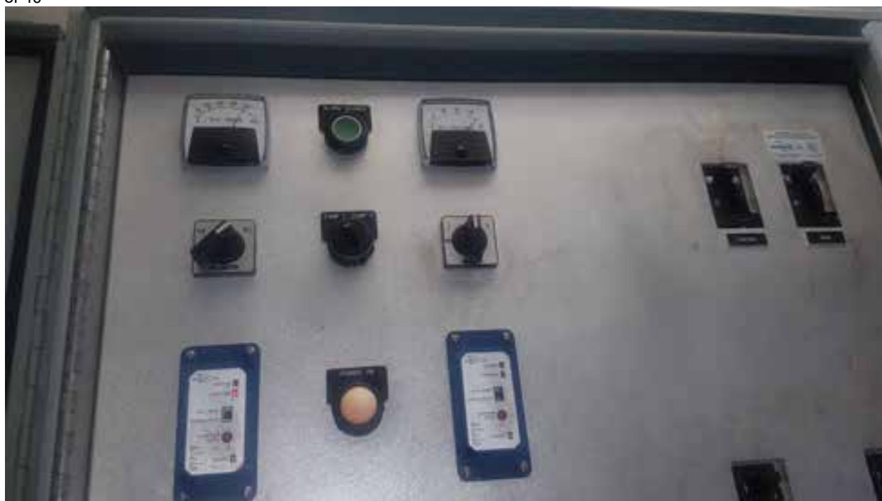
Figure 323 - covenant lift station - Pump control panel.
