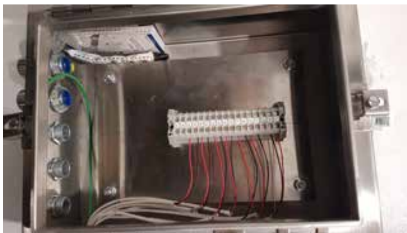
Figure 7 - "Sparkless" control panel box wiring
