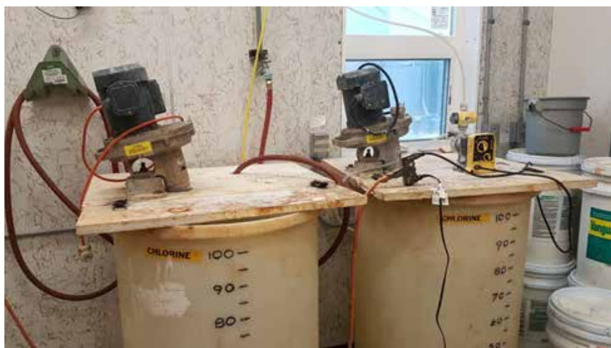
Figure 22 - Chlorine vats - Only one operational pump - Crew swaps pump between tanks as needed.
