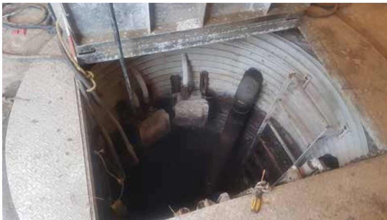
Figure 32 - Terminal Lift Station - Show of wet well. Functioning pump is on entrance side. Power junction boxes should be taken out of the wet well, and new ones placed above with conduit running down into wetwell.
