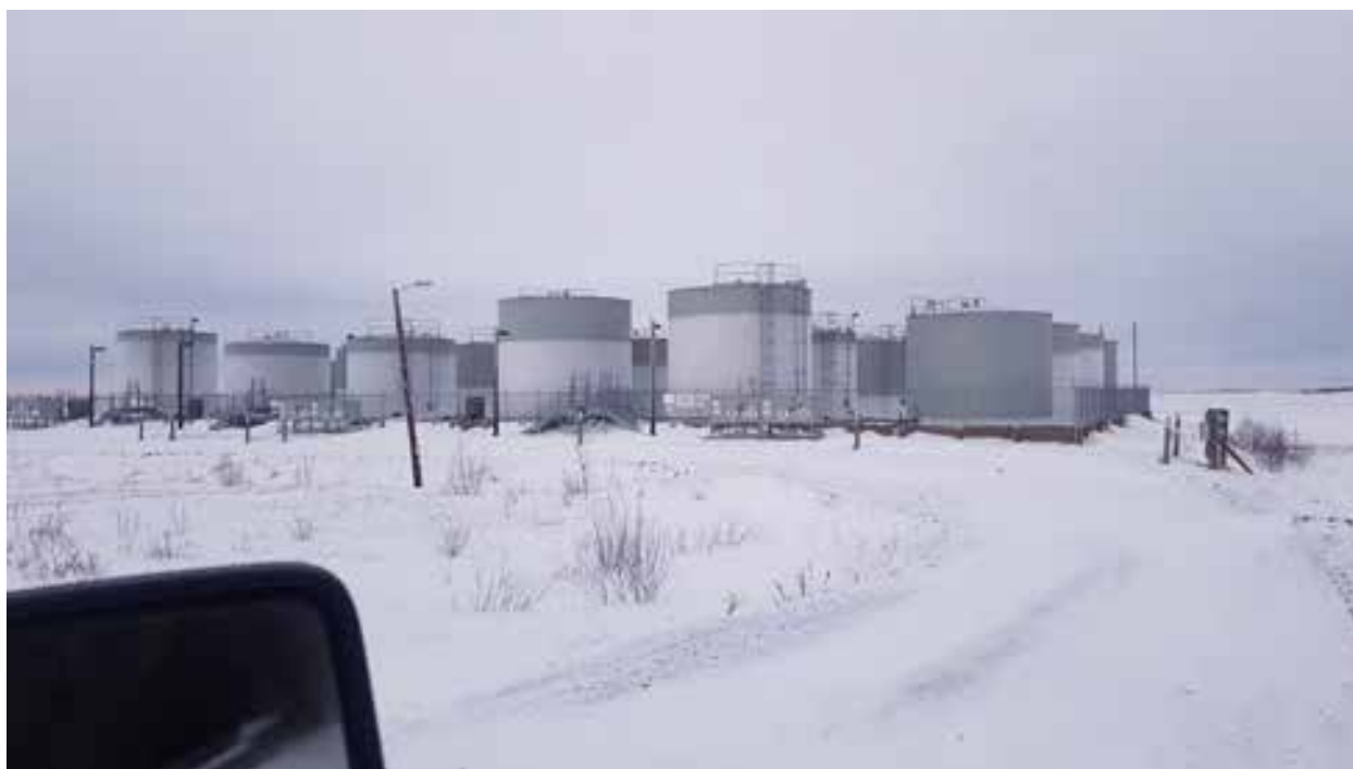
Figure 50 - City tank fuel farm, levels are easy to see because of frost.
