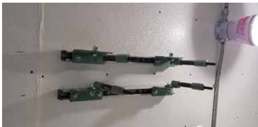
Figure 5 - Wet Well Heater Mounting Brackets
