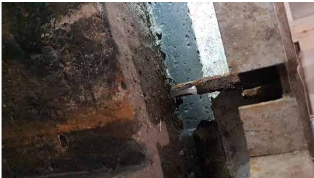
Figure 46 - HVLS Existing Wet Well hatch - interior shot showing hinge and how angle iron is set in concrete
