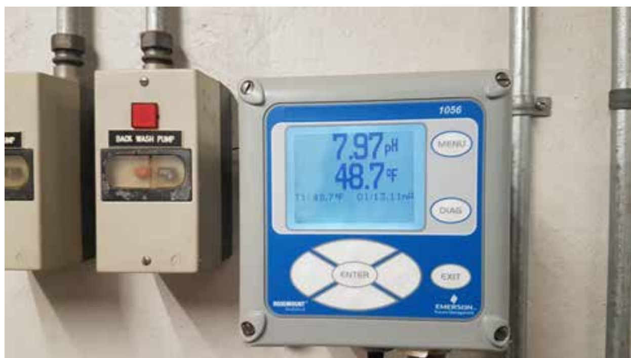
Figure 16 pH meter of treated water - Probe needs calibration – Sensor located on treated water to tank line
