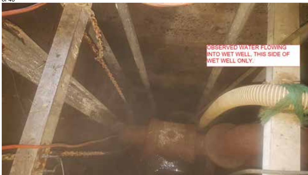
Figure 27 - FAA Lift station - Water seeping through wet-well, especially when utilidors are flooded
