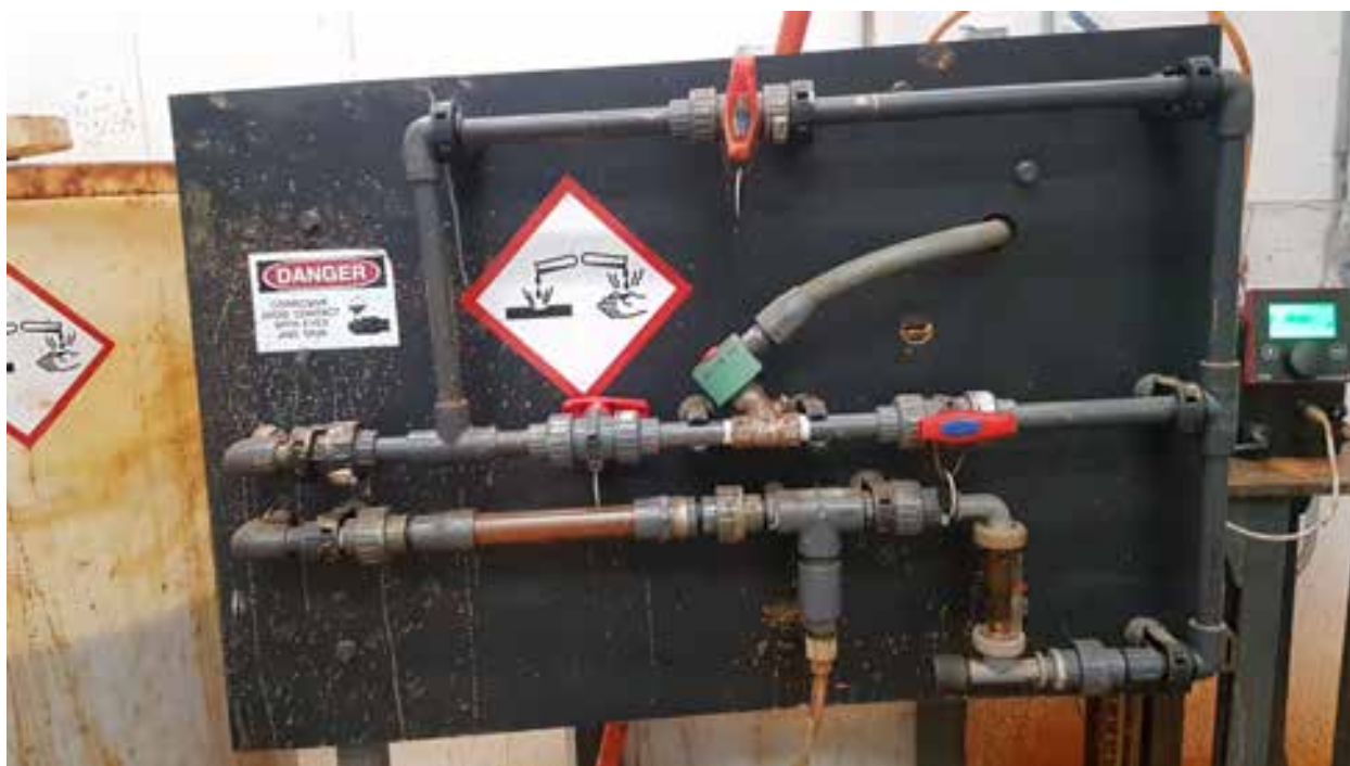
Figure 20 FeCl Neat Tank to Stock Solution tank mixing manifold. This needs some repairs.
