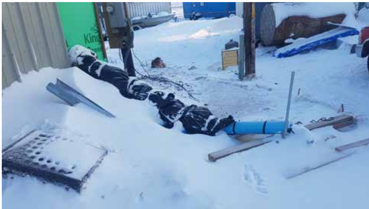
Figure 341 - HVLS Daytime shot of temp bypass.
