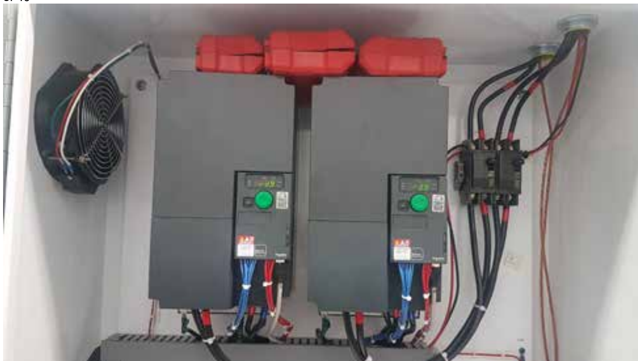
Figure 25 - Wiring in Pump Control Panel - single phase to three phase converters for VFDs
