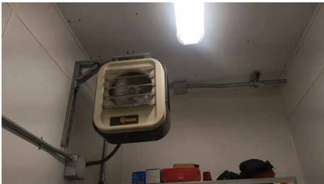
Figure 24 - New Heater in HVLC Control Room - Functioning
