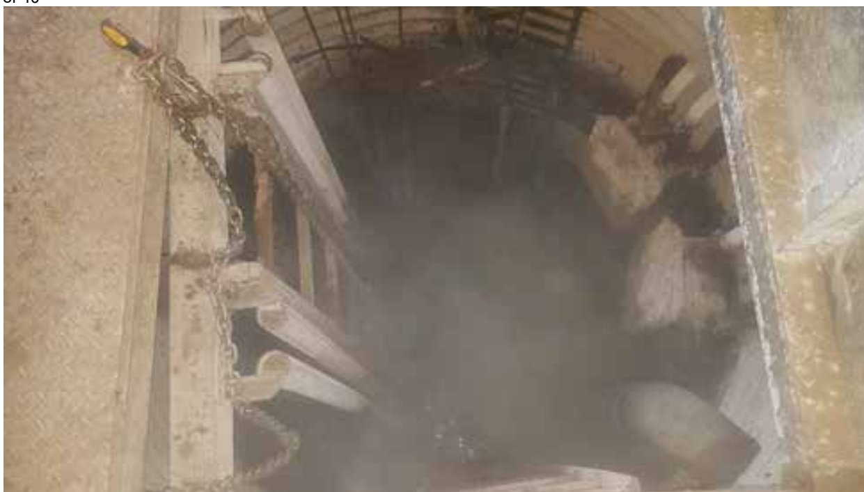
Figure 33 - Terminal Lift Station - Rails intact - side closes to picture is where pump was reportedly dropped and broke the bottom supports.
