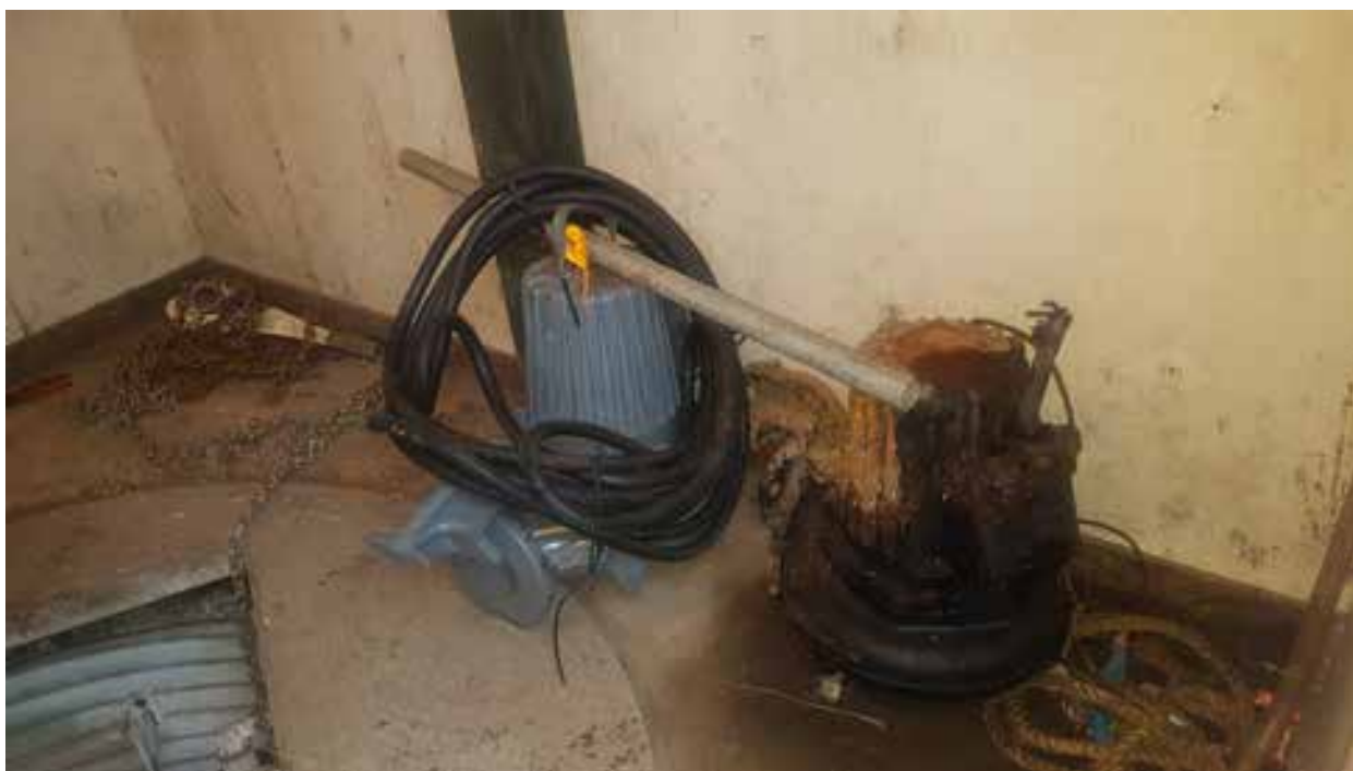
Figure 294 - Terminal Lift Station - Spare Pump - Could be installed if supports were fixed properly.
