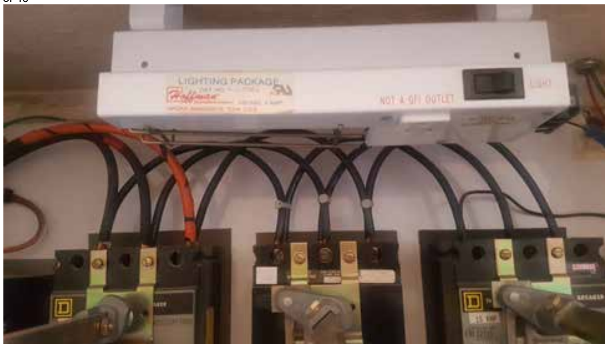
Figure 31 - Terminal Lift Station wiring - Interior looks good, only one picture to show general condition
