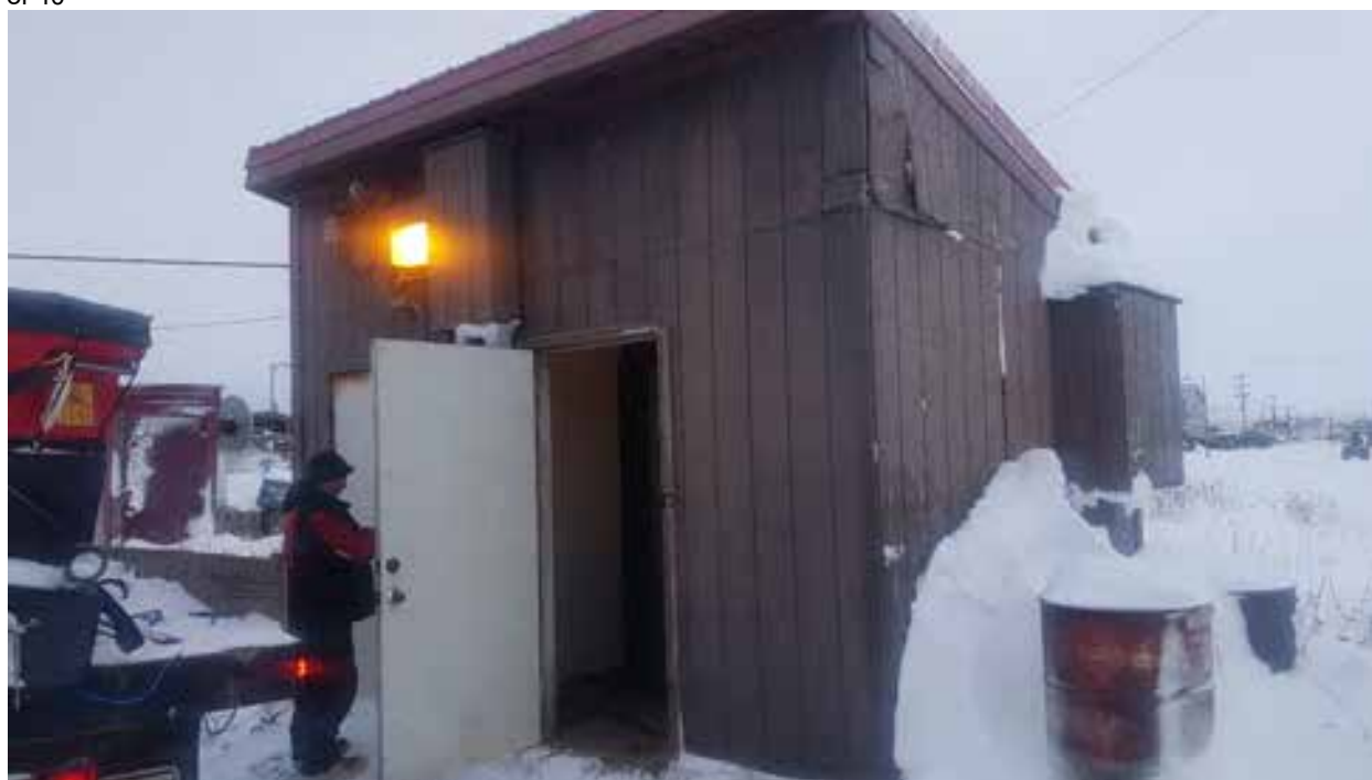
Figure 29 - Terminal Lift Station Exterior - Note Damage on Top Right Exterior
