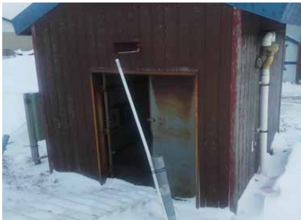
Figure 26 - FAA Lift station Exterior
