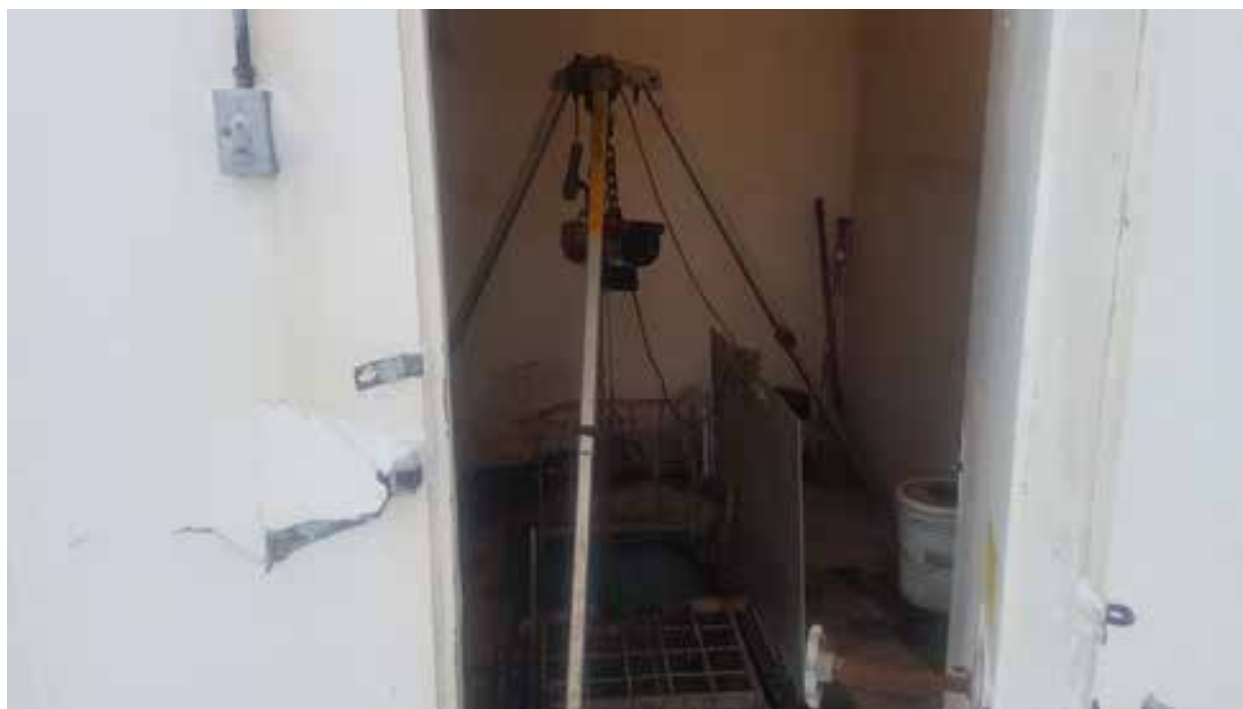
Figure 36 - Covenant Lift Station - Wet Well Room Interior
