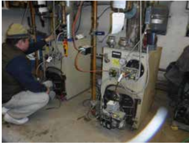
Figure 4: Boiler 1 (Left Side)
