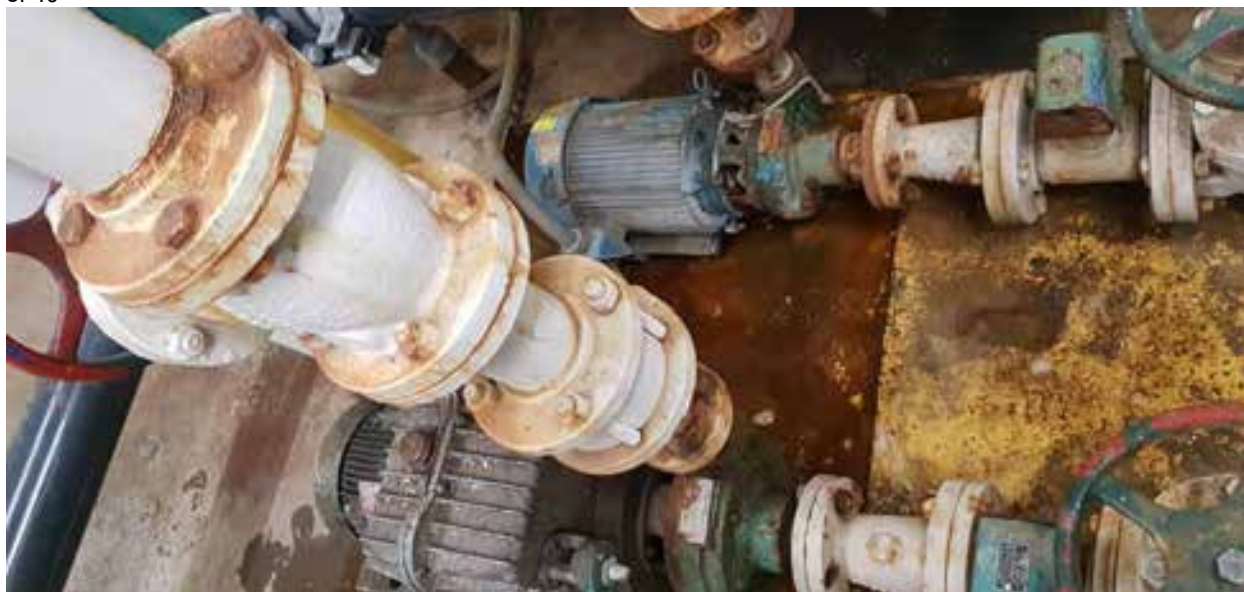
Figure 23 - Plant Booster Pumps - right pump working, left malfunctioning
