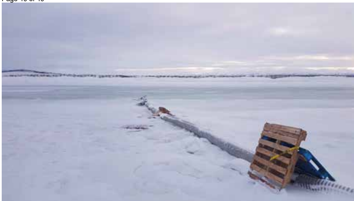
Figure 55 - Slough Bypass for freeze prevention of system.
