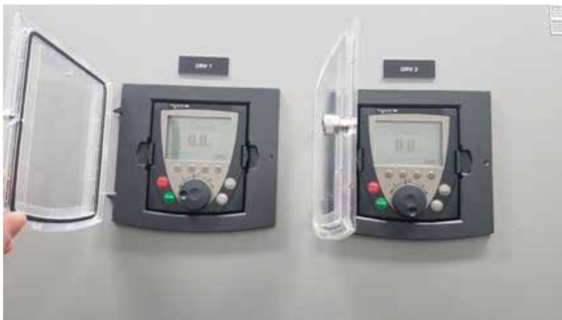
Figure 1 - HVLS Pump VFD Control Panels
