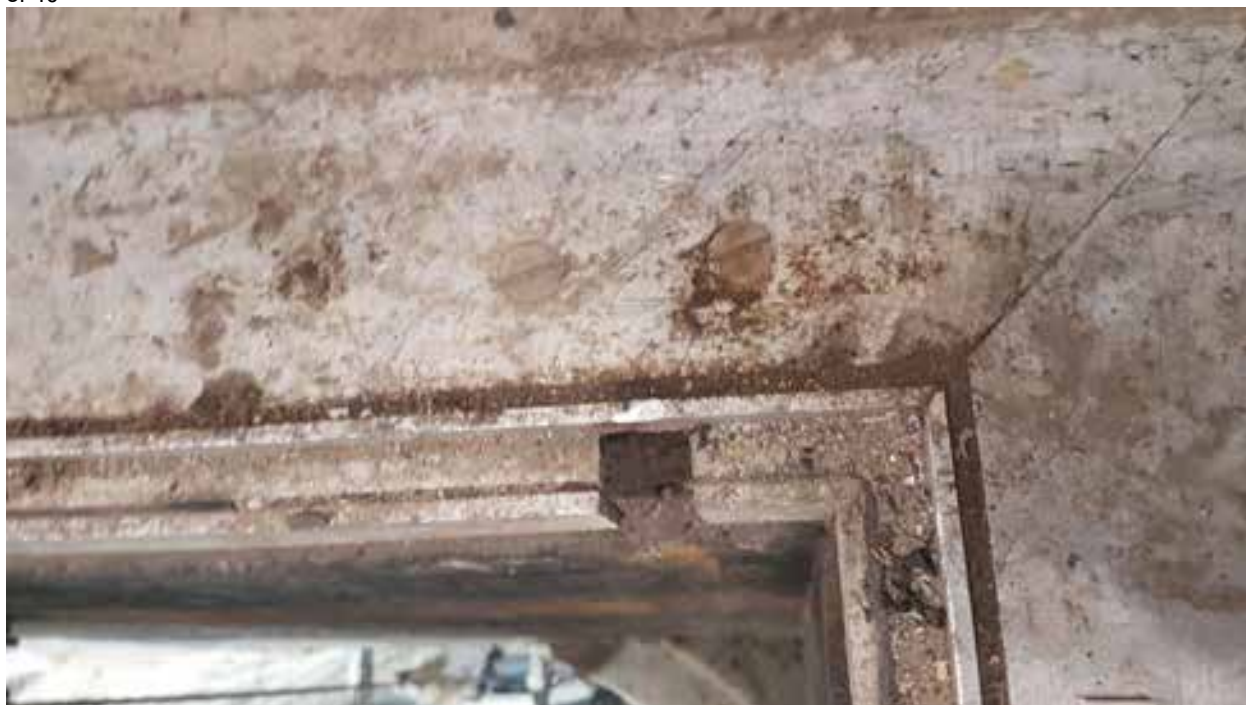
Figure 45 - HVLS wet well hatch existing - requires demolition prior to installation of new hatch
