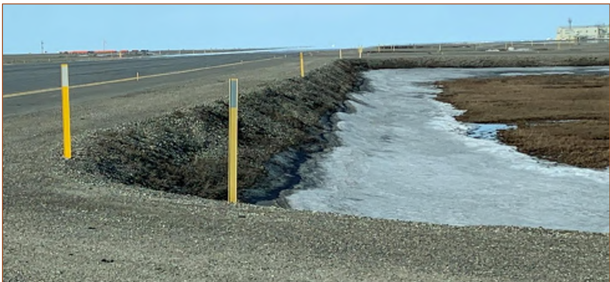
Figure 4-2: Steep Taxiway Shoulder Slopes and Erodible Materials
