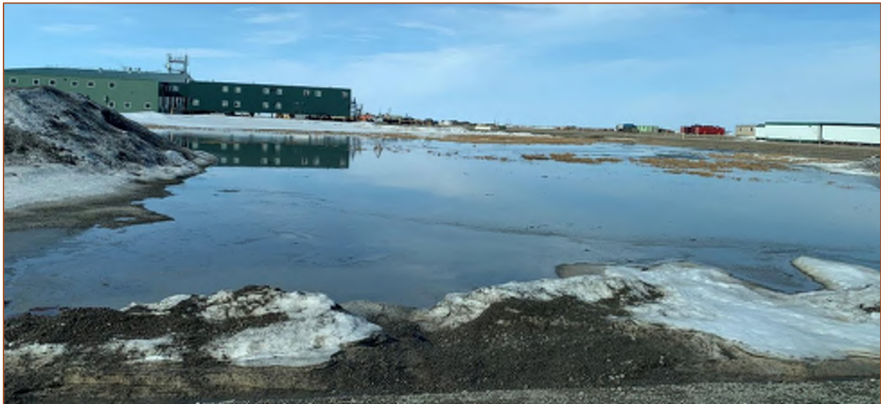
Figure 4-7: Ponding in Front of ARFF/SREB Parking Lot
