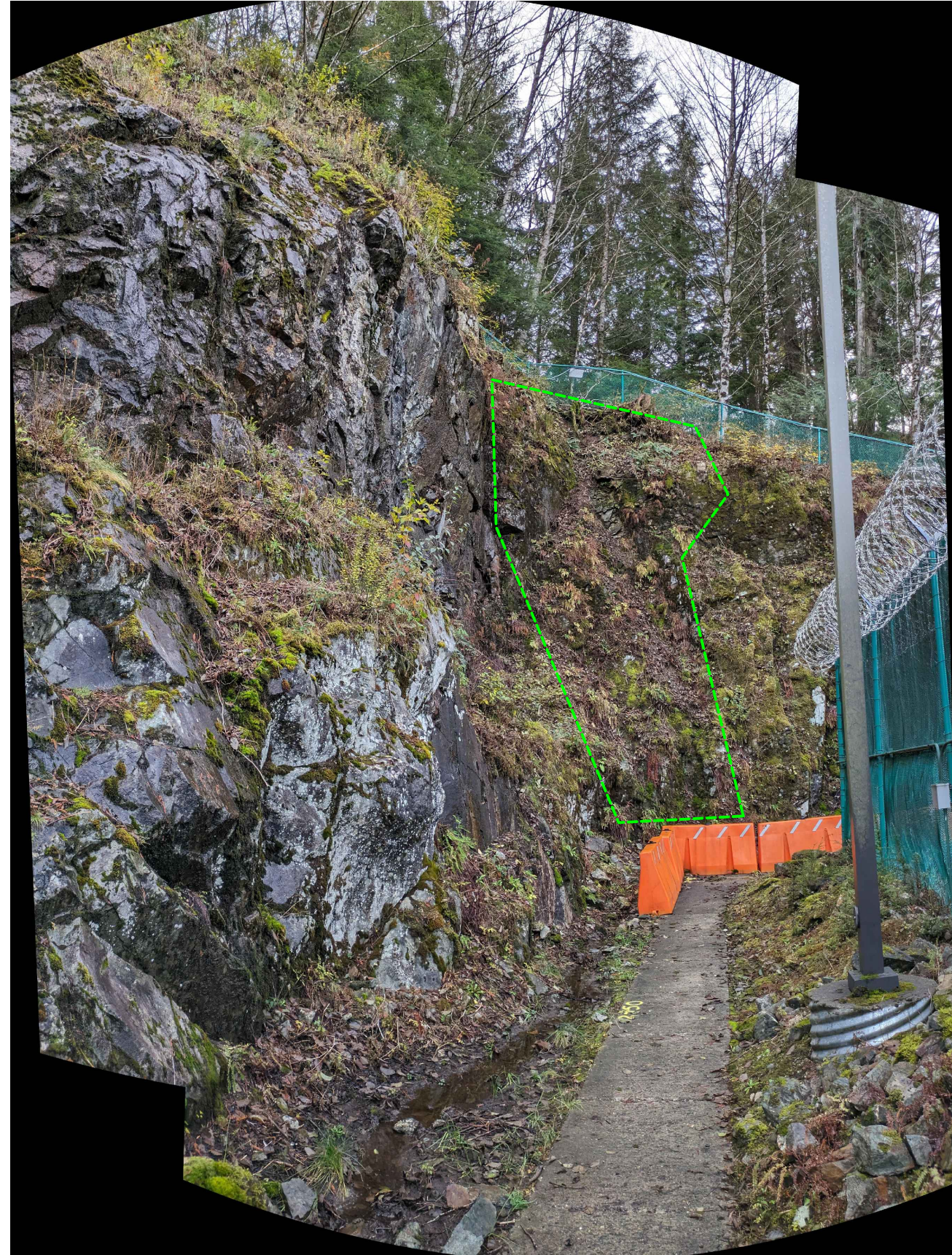
STATION 2+75 to 3+00 – HEAVY SCALING LOCATIONS
