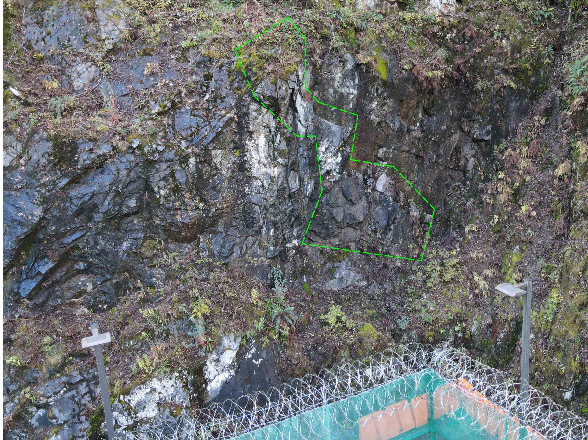
STA. 2+60 to STA. 2+70 – HEAVY SCALING LOCATIONS
