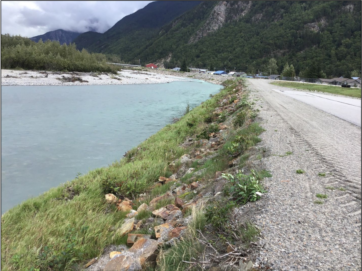
Figure 7. Portion of the Skagway River levee along the Skagway Airport looking northeast at Runway 20, in August 2024.
