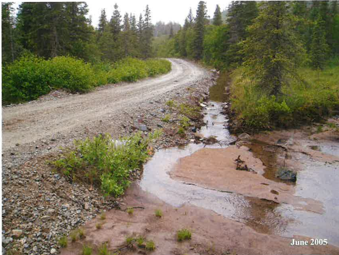
MP 9.2 - Looking northwest along the road. Two culverts allow for drainage in this area.
