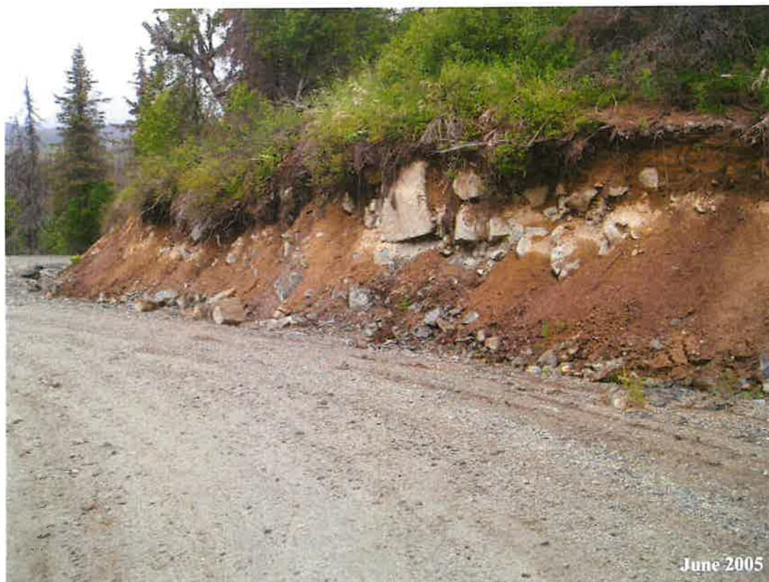
MP 9.4 - Top of the "S-curve". The embankment shown consists of organic and silt overburden, glacial till, and bedrock.
