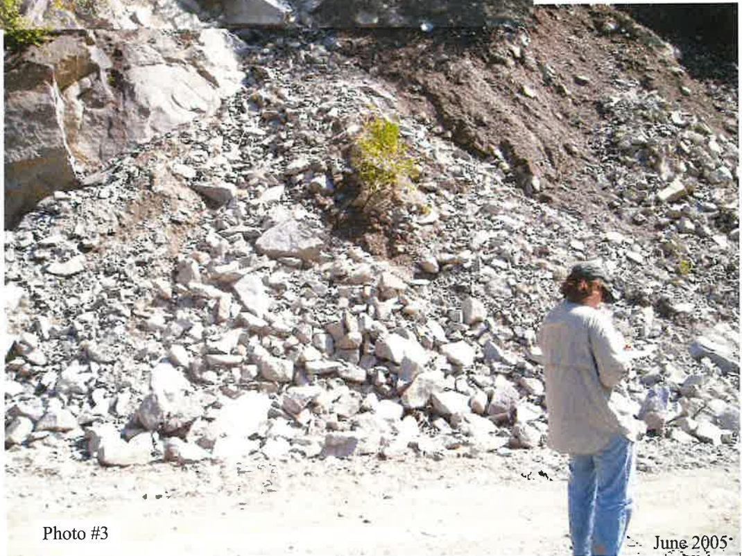
MP 1.0 - Looking up at the rock "chute" and the talus fan at the road. Rock fall area.
