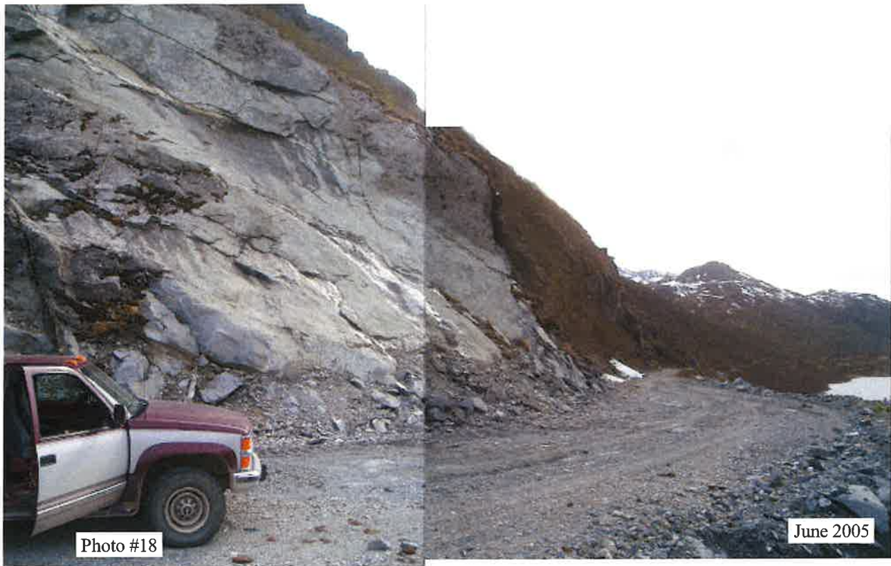
MP 2.2 - Slope failure surfaces/exfoliation type weathering along joints. North is to the right in the photo.
