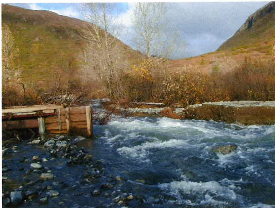
MP 7.6 - Embankment wash out at the bridge that crosses Timberline Creek.
