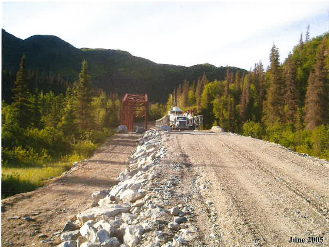
MP 11 - New bridge next to the old bridge at the Iliamna River. The bridge is about 2-3 ft higher than the old bridge.
