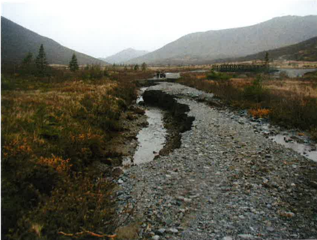
MP 3.6 - Looking at the road washed out at the bridge that crosses Chinkelyes Creek. The bridge is in the background of photo. Looking back toward Williamsport.
