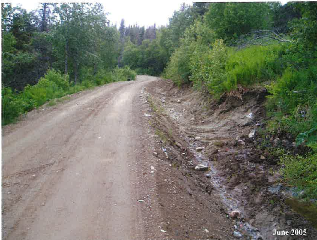
MP 11.4 - The maintenance contractor widened the ditch in this area for better drainage.
