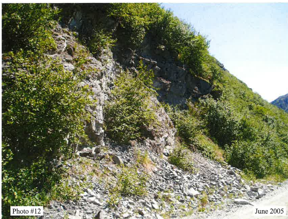
MP 1.35 - Relatively smaller cuts. Less rock fall problems. Rock structure is similar as MP 1.1.
