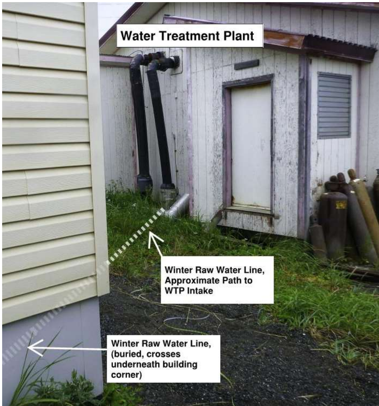
Figure 22: Winter raw water pipe routing at Water Treatment Plant.
