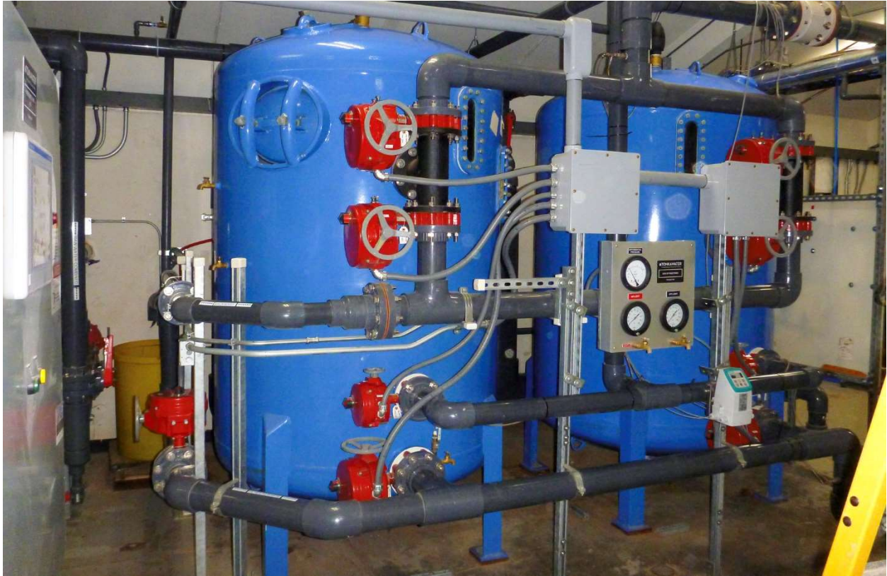
Figure 31: WTP mixed media filters (5 feet diameter by 8 feet tall. The WTP operator reported that these filters were installed as part of a 2018 project by Bristol construction. The new filters are larger than the old filters. Community officials believe the additional weight of the new filters is causing foundation settlement and structural issues at the WTP.
