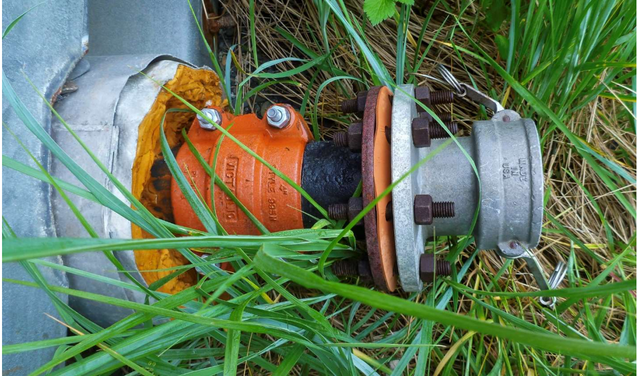
Figure 16: Raw water line connection point (photo 2 of 5).
