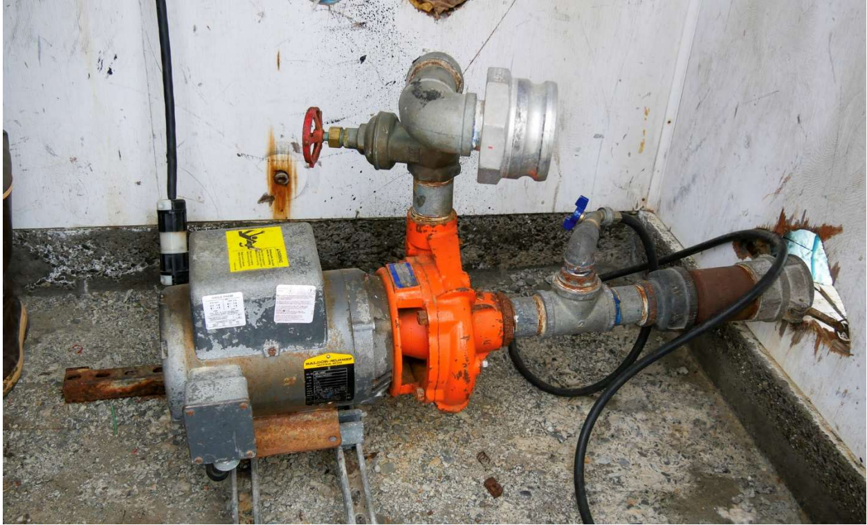
Figure 11: Winter water source 5 HP pump within the pump house (pump is removed during flooding).
