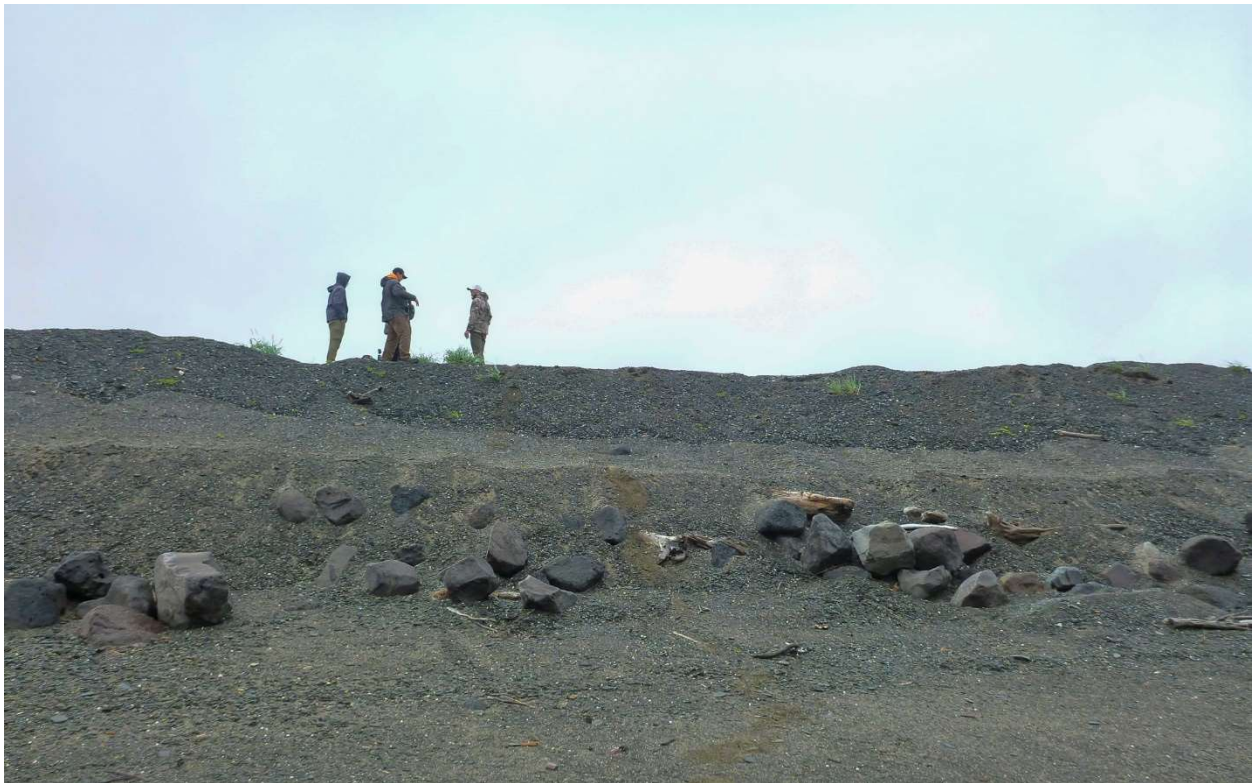
Figure 46: Collapsed rock protection and high water line visible along the berm (Looking from ocean shore inland).
