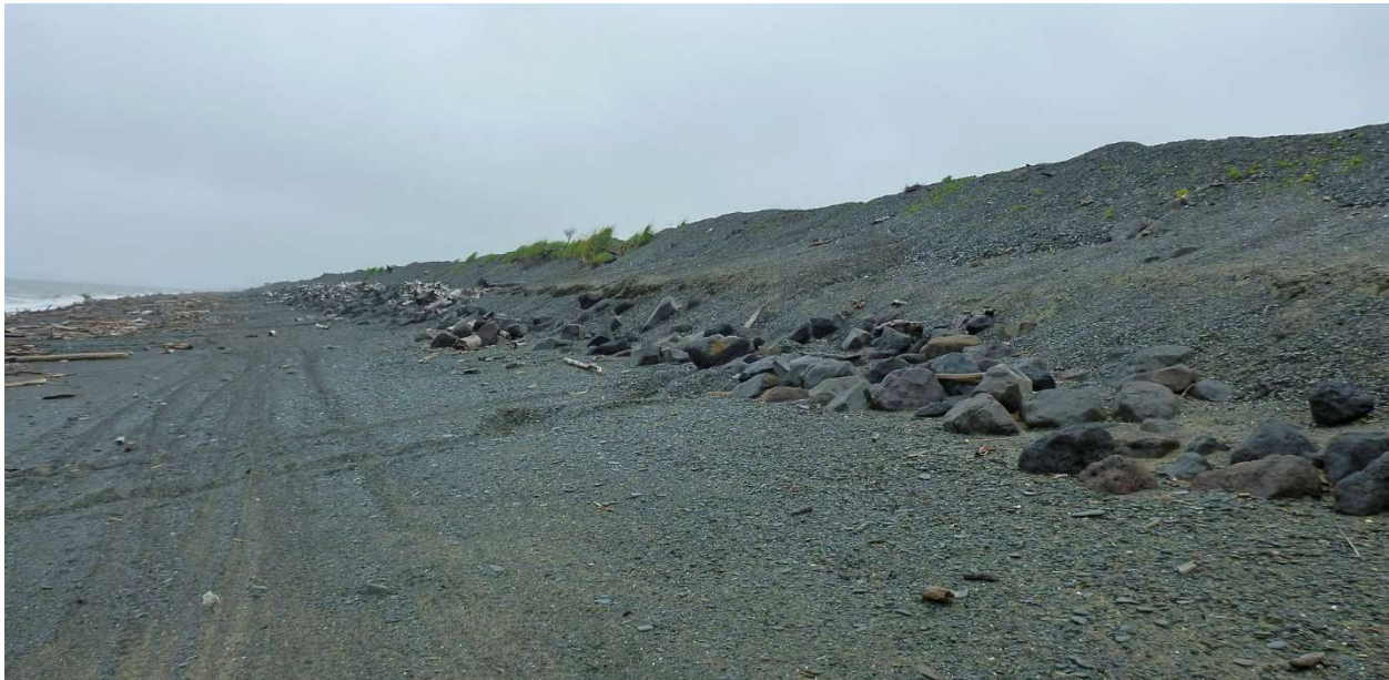
Figure 44: Collapsed rock protection placed along the berm. (Looking from the berm north toward Shaktoolik)
