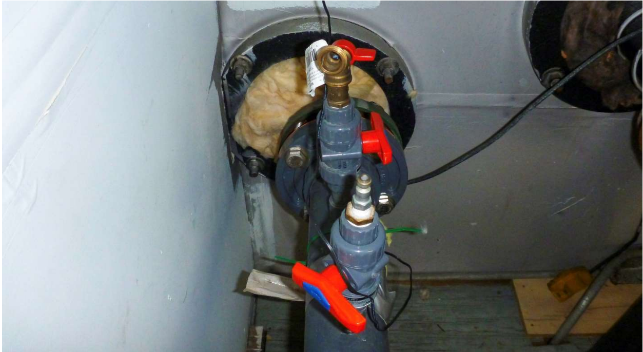
Figure 24: Winter raw water pipe as it penetrates inside the WTP. The small valves and attachments are used by operators to attempt to thaw ice in the pipe by alternately injecting warm water and compressed air.
