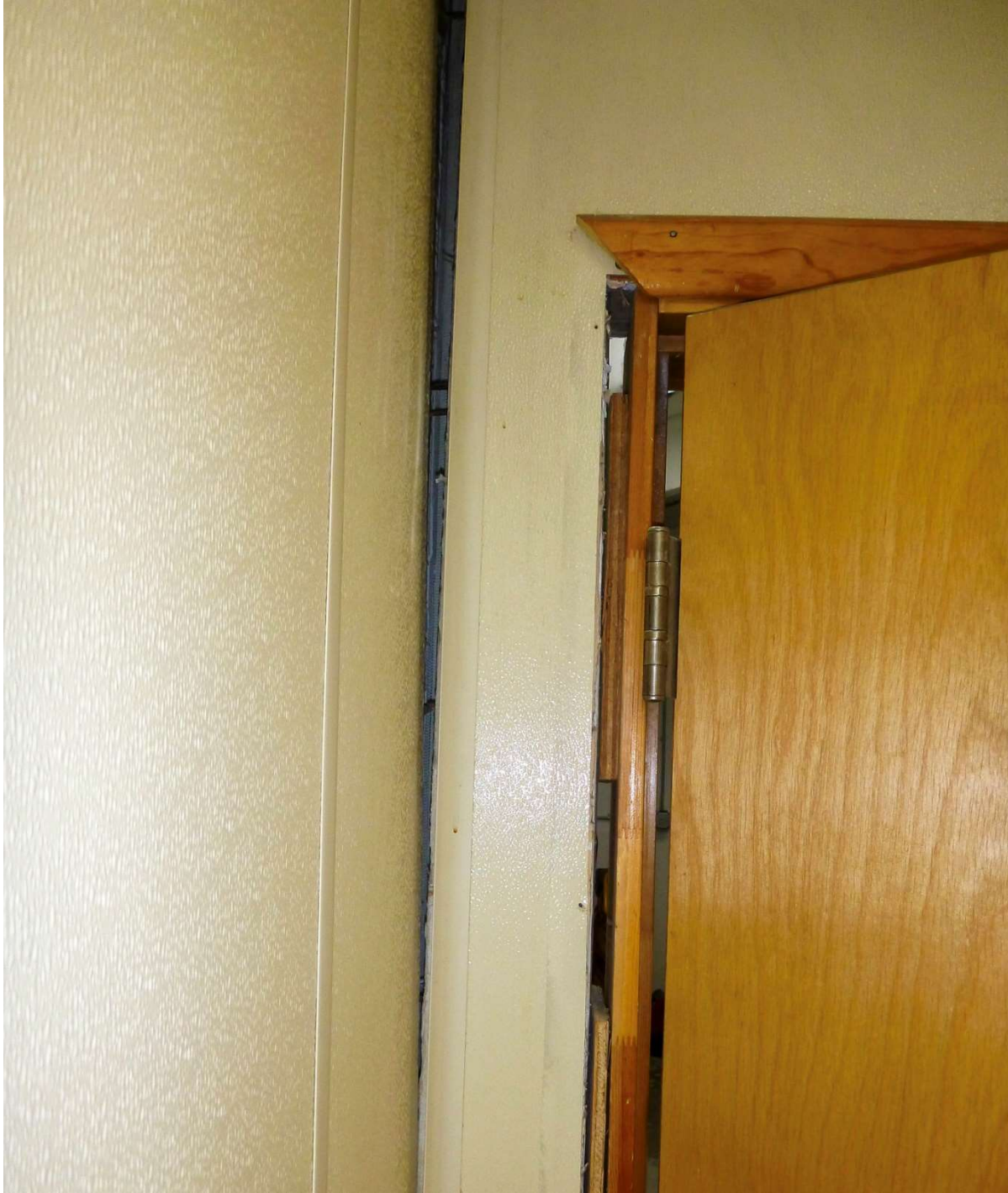
Figure 36: Cracks along exterior walls. WTP operation logs indicate the facility is unable to maintain room temperature during winter within the building. Community officials reported these cracks appeared after installation of the new mixed media filters (photo 4 of 5).
