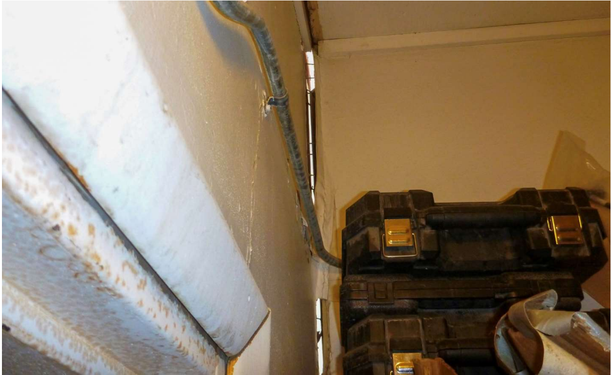
Figure 33: One of several locations where daylight is visible along exterior walls of the WTP . WTP operation logs indicated the facility is unable to maintain room temperature during winter within the building. Community officials reported these cracks appeared after installation of the new mixed media filters (Photo 1 of 5).
