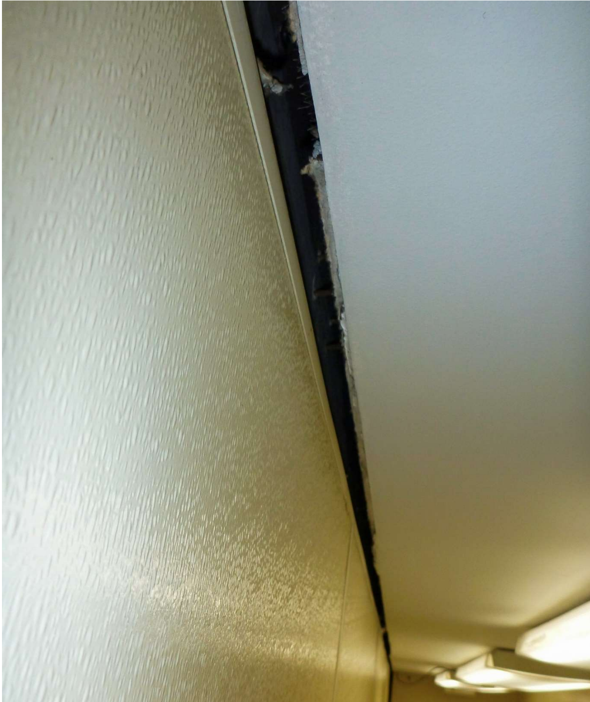
Figure 34: Cracks along exterior walls of the WTP. WTP operation logs indicate the facility is unable to maintain room temperature during winter within the building. Community officials reported these cracks appeared after installation of the new mixed media filters (photo 2 of 5).
