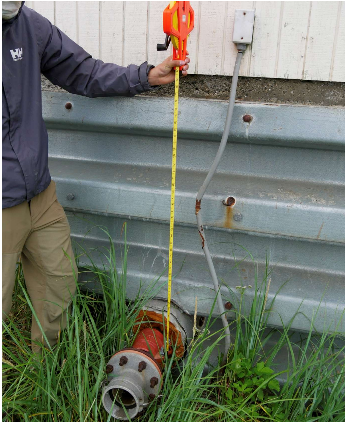
Figure 15: The raw water line connection point (at the pump house) that connects to the WTP via 600 feet of buried arctic pipe. The 600 foot long arctic pipe runs at approximately a 1% grade to gravity drain back to the river. The connection point features a cam-lock hose connection fitting, but no valve. The connection is regularly inundated at high tide such that seawater surcharges into the pipe and freezes within the pipe. The heat trace previously run through the arctic pipe is no longer functional. Frozen seawater inside this pipe is the primary concern with the existing winter water source. The frozen seawater is impossible to prevent without a valve, is challenging to thaw, and frequently delays wintertime pumping operations (Raw water line connection point photo 1 of 5).
