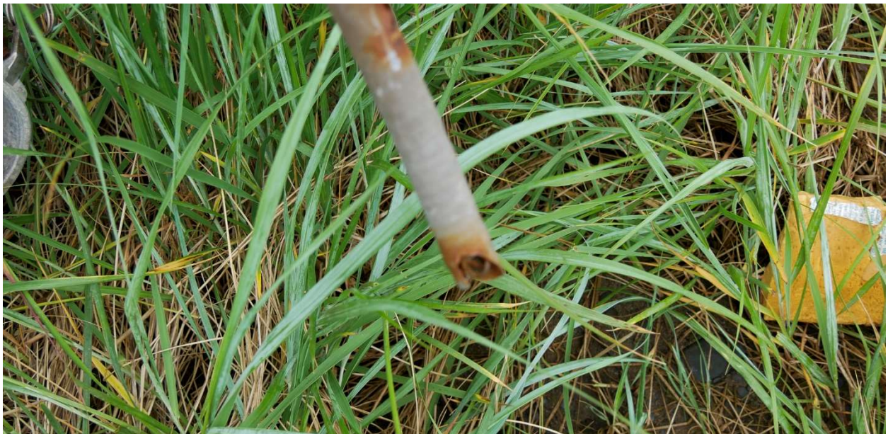
Figure 19: Corroded and disconnected heat trace wire at the raw water line connection point (photo 5 of 5).
