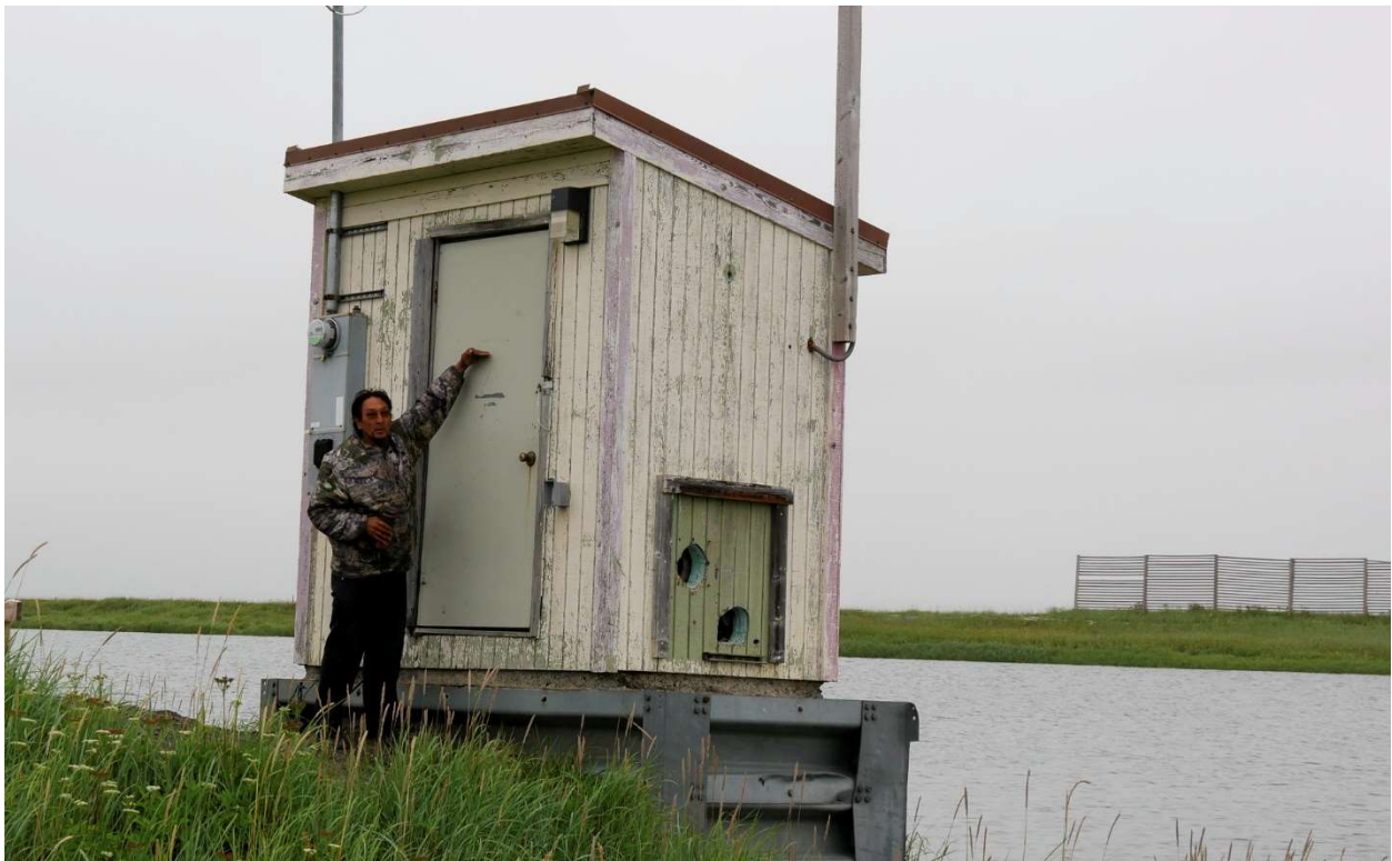
Figure 8: WTP Operator Mr. Nakarak indicating the estimated high water line during fall storm surge flooding. Note the location of the electrical box. No remote service disconnect switch is available to de-energize the pump house during extreme flooding.
