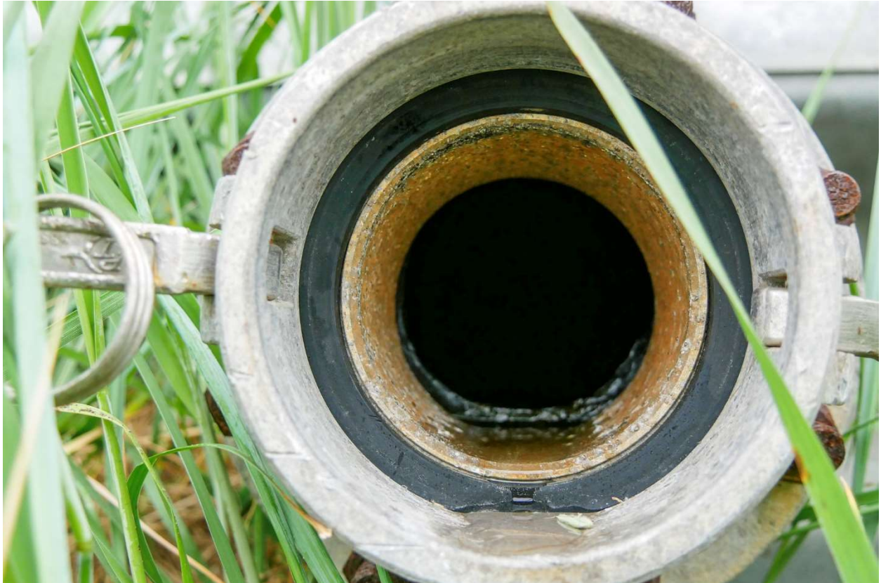
Figure 18: Raw water line connection point, with residual water from high tide visible (photo 4 of 5).
