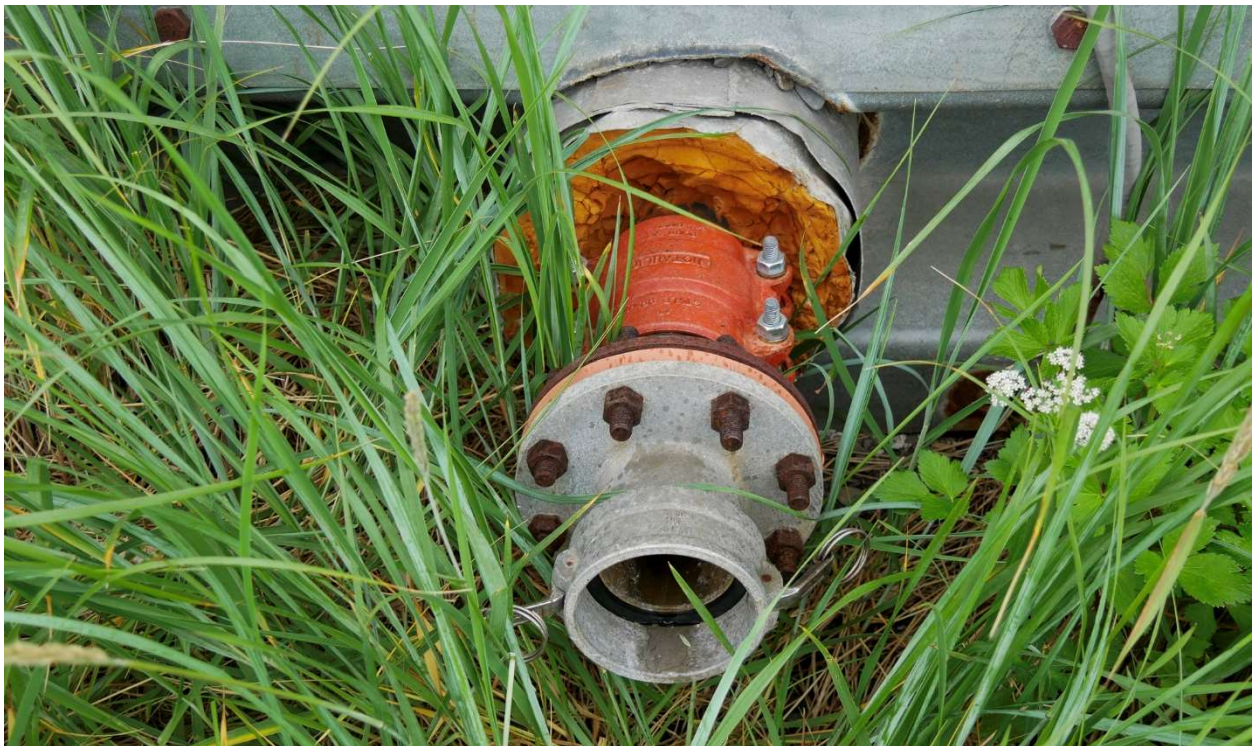
Figure 17: Raw water line connection point (photo 3 of 5).
