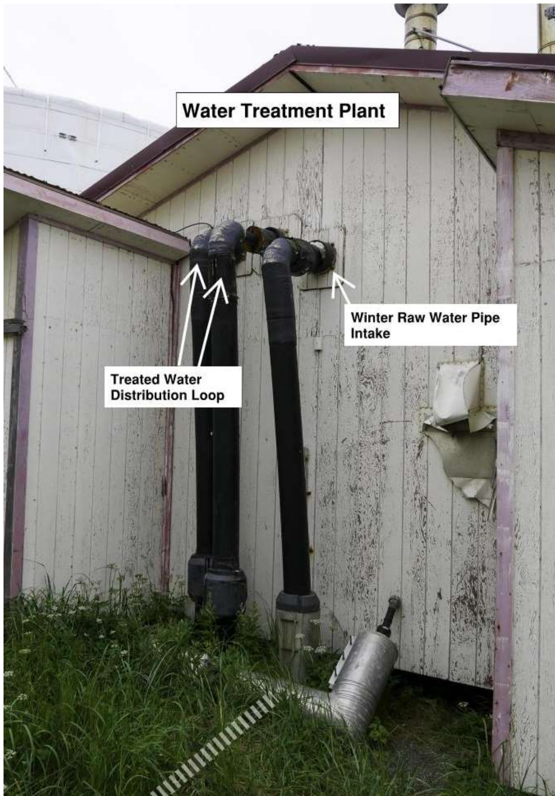
Figure 23: Winter raw water pipe routing into Water Treatment Plant. Note, differential settlement has caused the insulation jacket on the winter raw water pipe to separate where it penetrates the building.
