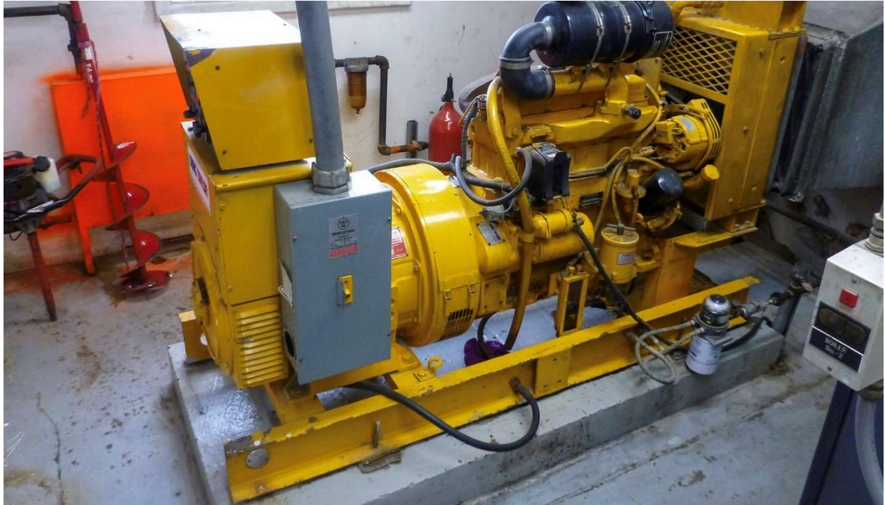
Figure 29: WTP backup generator.
