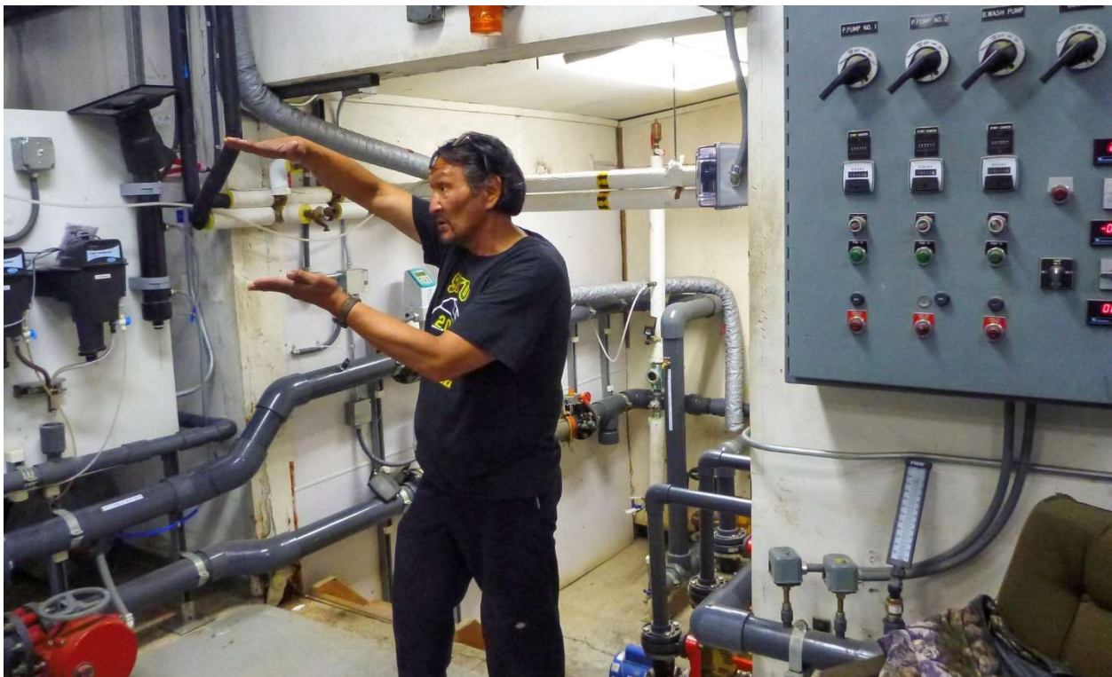
Figure 28: Mr. Nakarak describing WTP operations.
