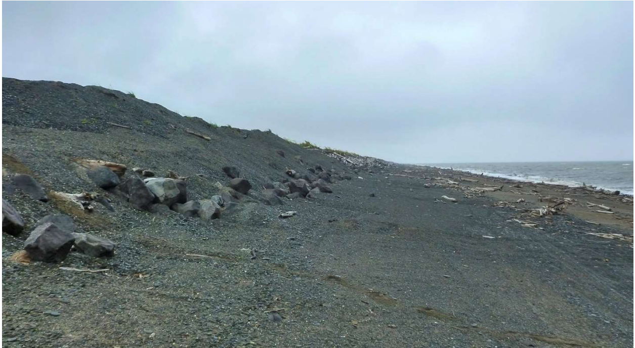
Figure 45: Collapsed rock protection placed along the berm. (Looking from the berm south away from Shaktoolik).
