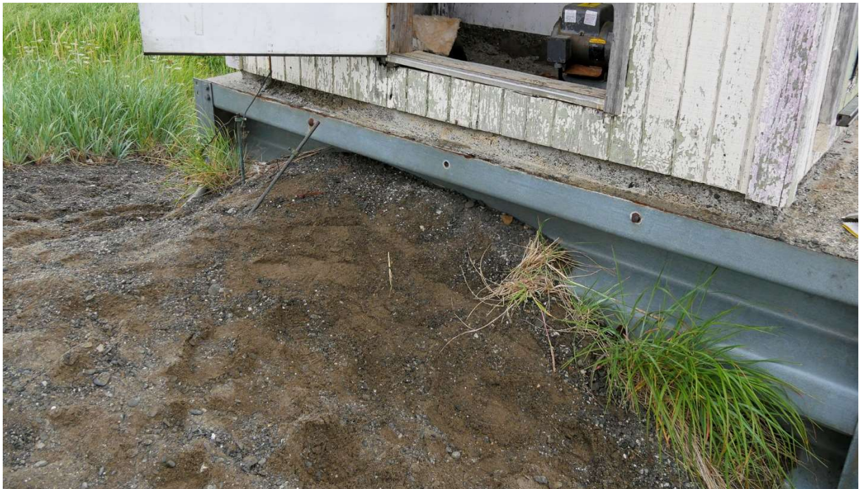
Figure 14: Mild erosion around the foundation of the winter water source pump house.
