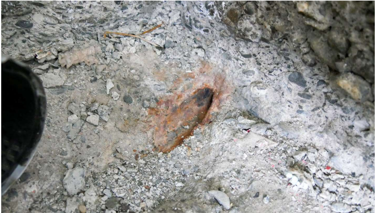
Figure 13: Floor drain hole within the winter water source pump house. Mr. Nakarak indicated that the drain hole occasionally freezes, impeding drainage after flooding. Note the concrete degradation of the floor.
