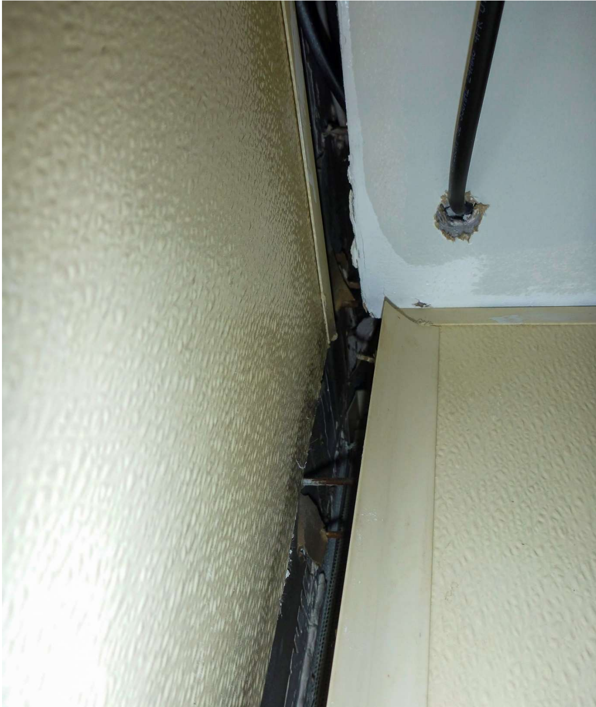
Figure 35: Cracks along exterior walls. WTP operation logs indicate the facility is unable to maintain room temperature during winter within the building. Community officials reported these cracks appeared after installation of the new mixed media filters (photo 3 of 5).
