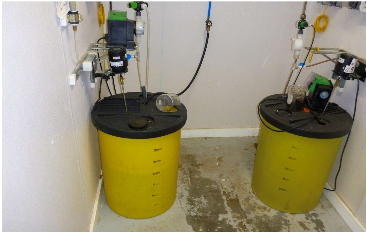
Figure 30: WTP Polymer and potassium permanganate feed systems.
