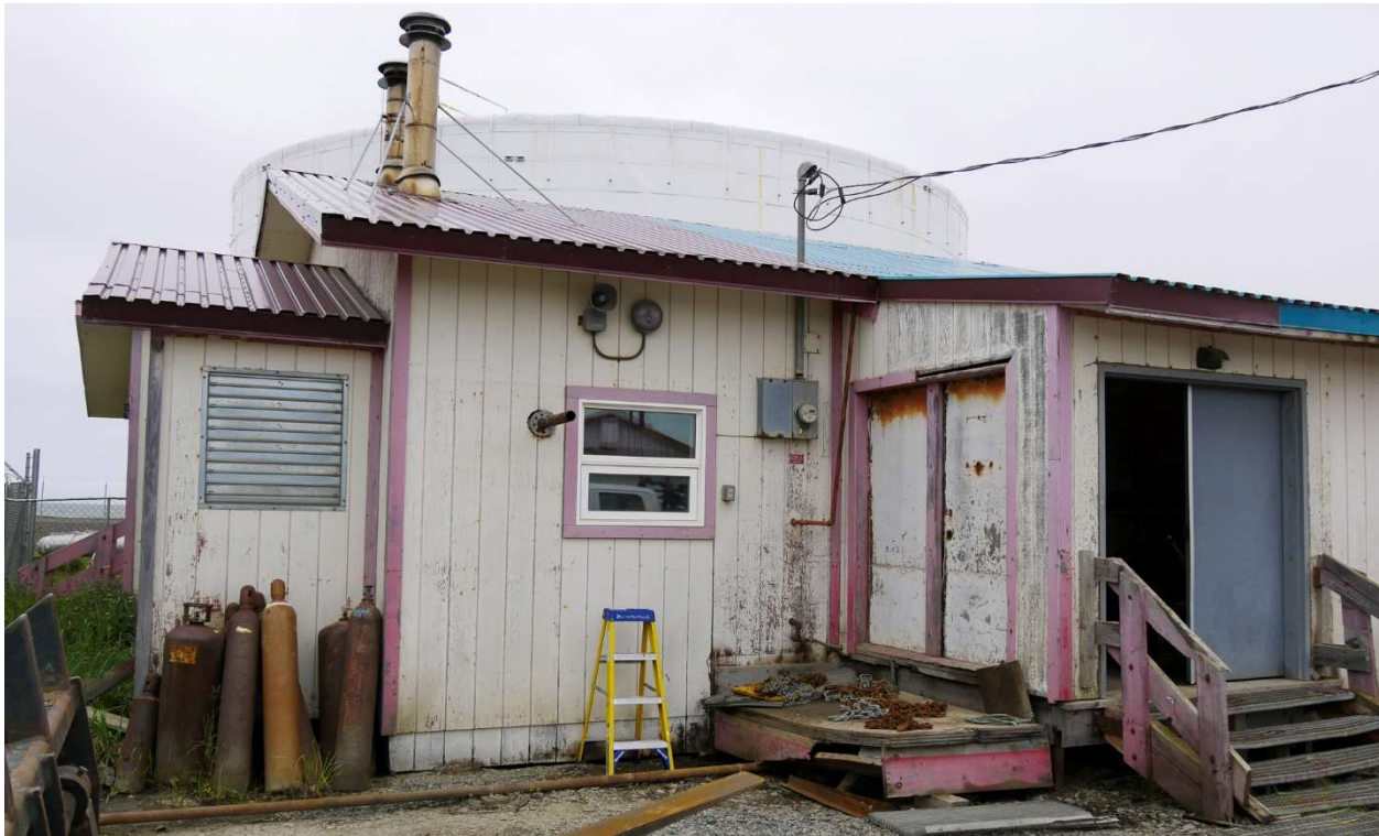
Figure 27: WTP (foreground) with 848,000 gallon water storage tank (background)
