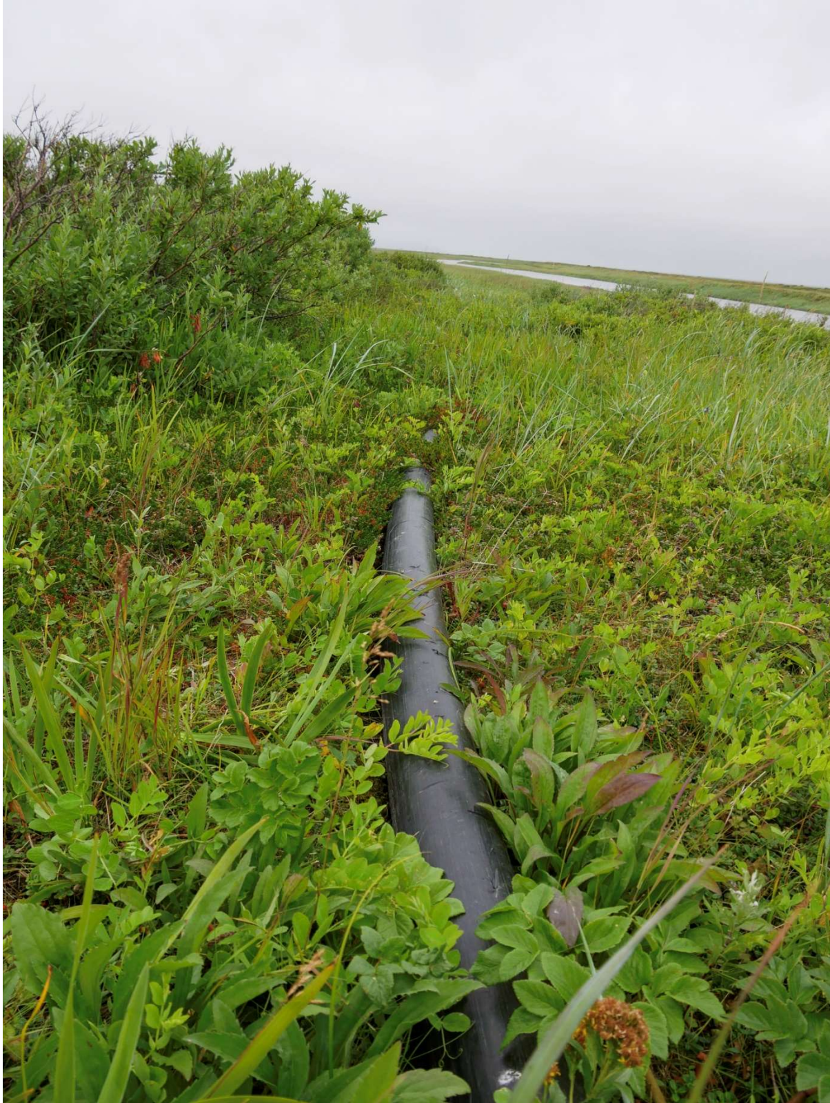
Figure 42: HDPE summer raw water supply line running across the surface of the tundra back to town. The line is approximately 6500 feet long, and is not insulated nor heat taped. The line is purged with air at the end of the year to prevent freezing.
