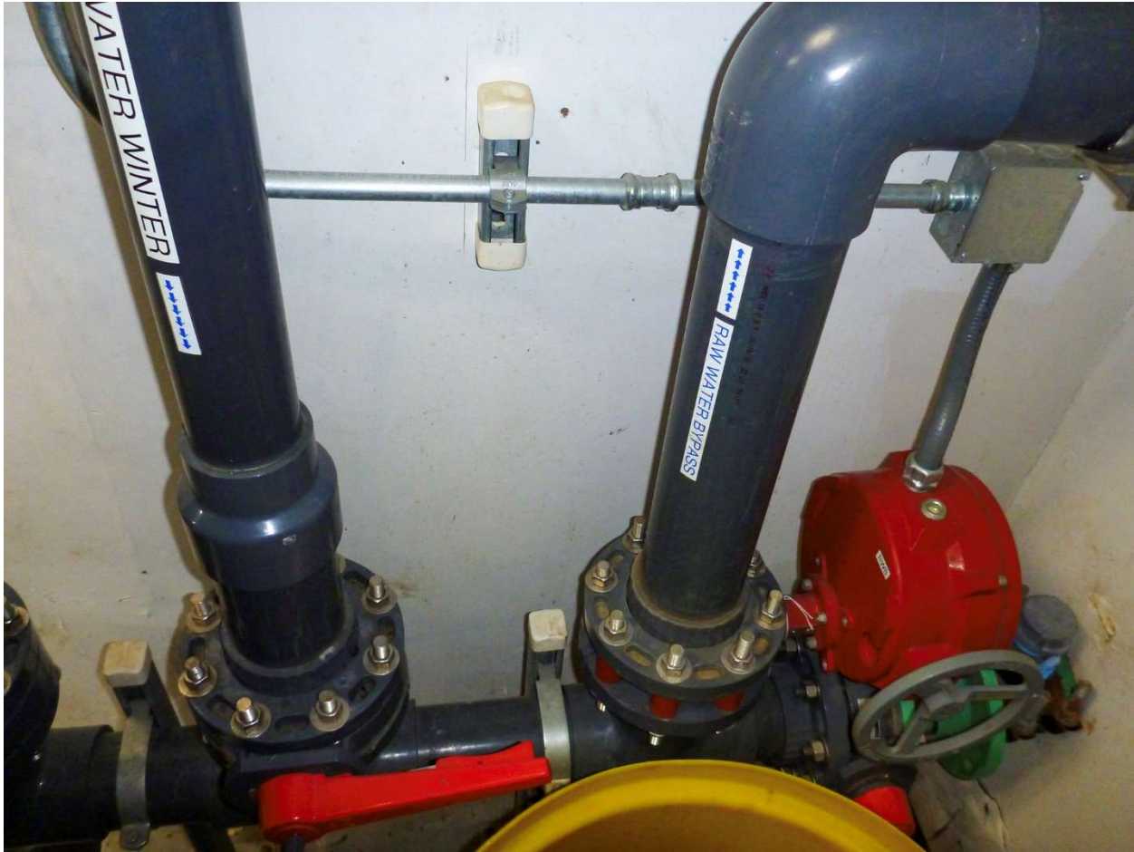
Figure 26: Raw water bypass valve system. Water is automatically wasted above a set point of 500 microsiemens per centimeter.
