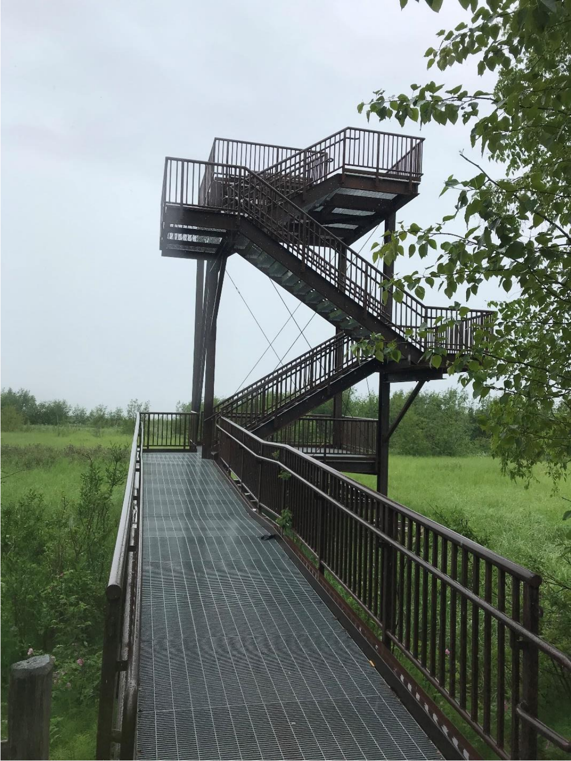
2023 – tower leaning, NW piling lifting & SE piling compressed/sinking
