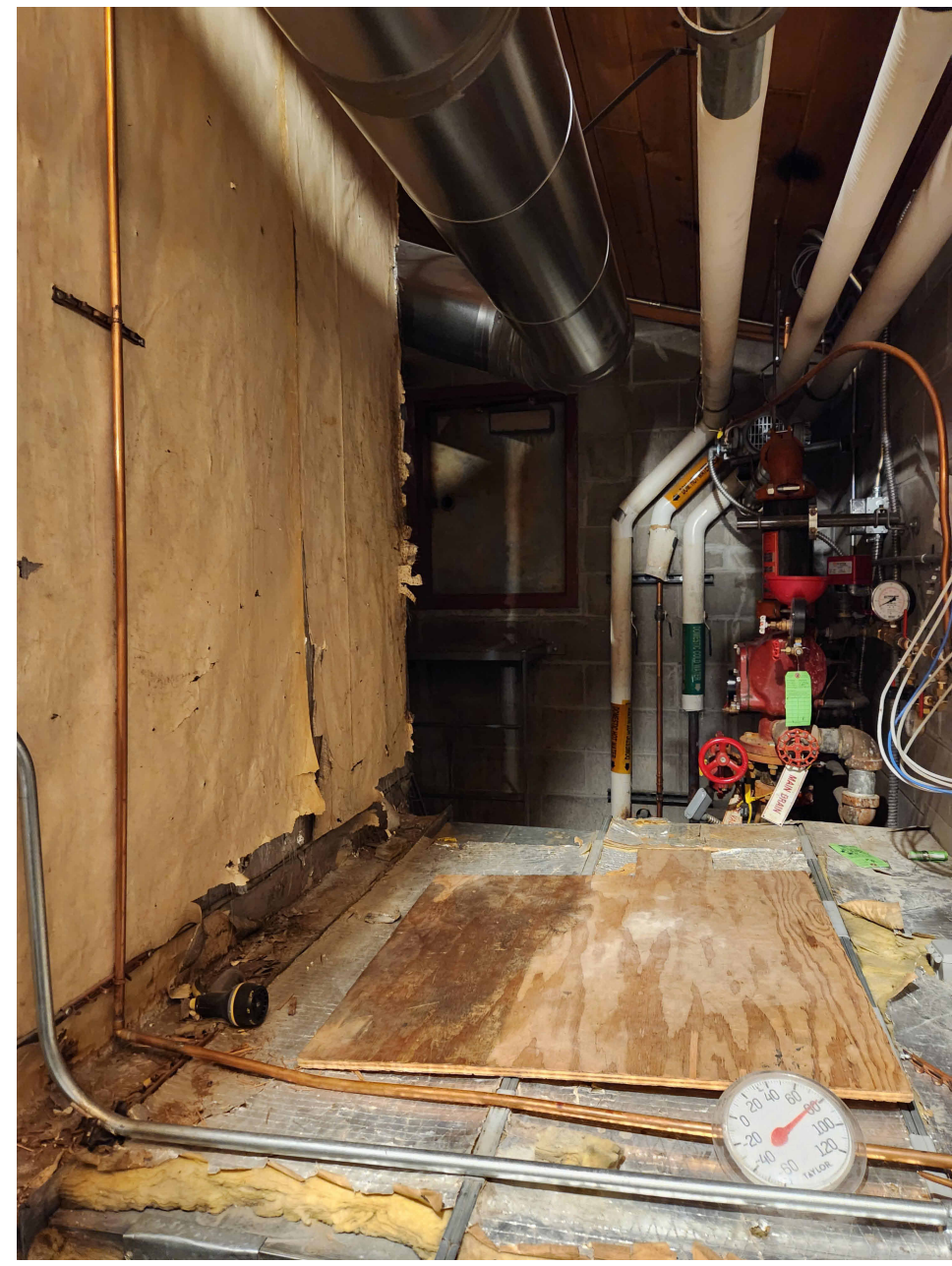
3 FAN ROOM ACCESS OVER DUCTWORK
