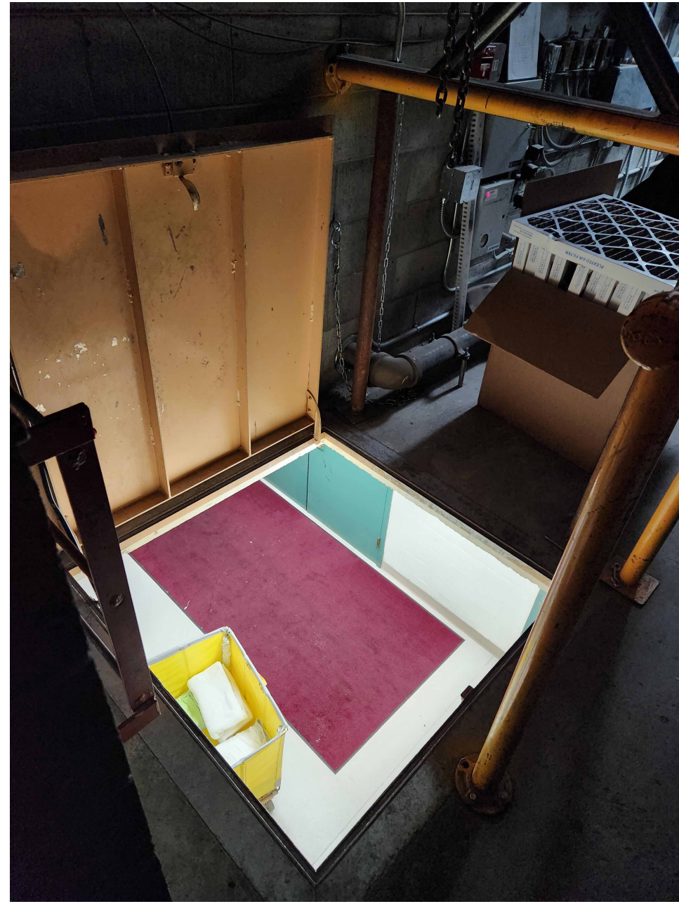
1 FAN ROOM ACCESS HATCH AND HOIST
