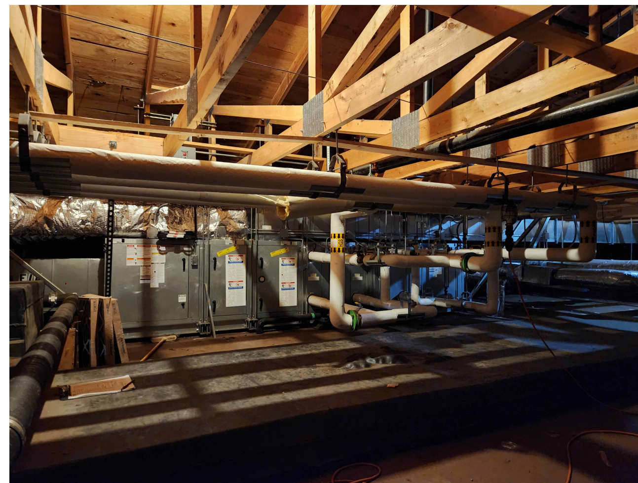
7 ATTIC - AHU AND HYDRONIC LINES
