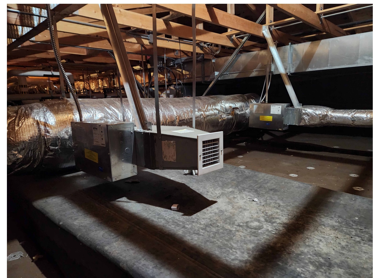
10 ATTIC - HVAC SUPPLY TO ATTIC SPACE
