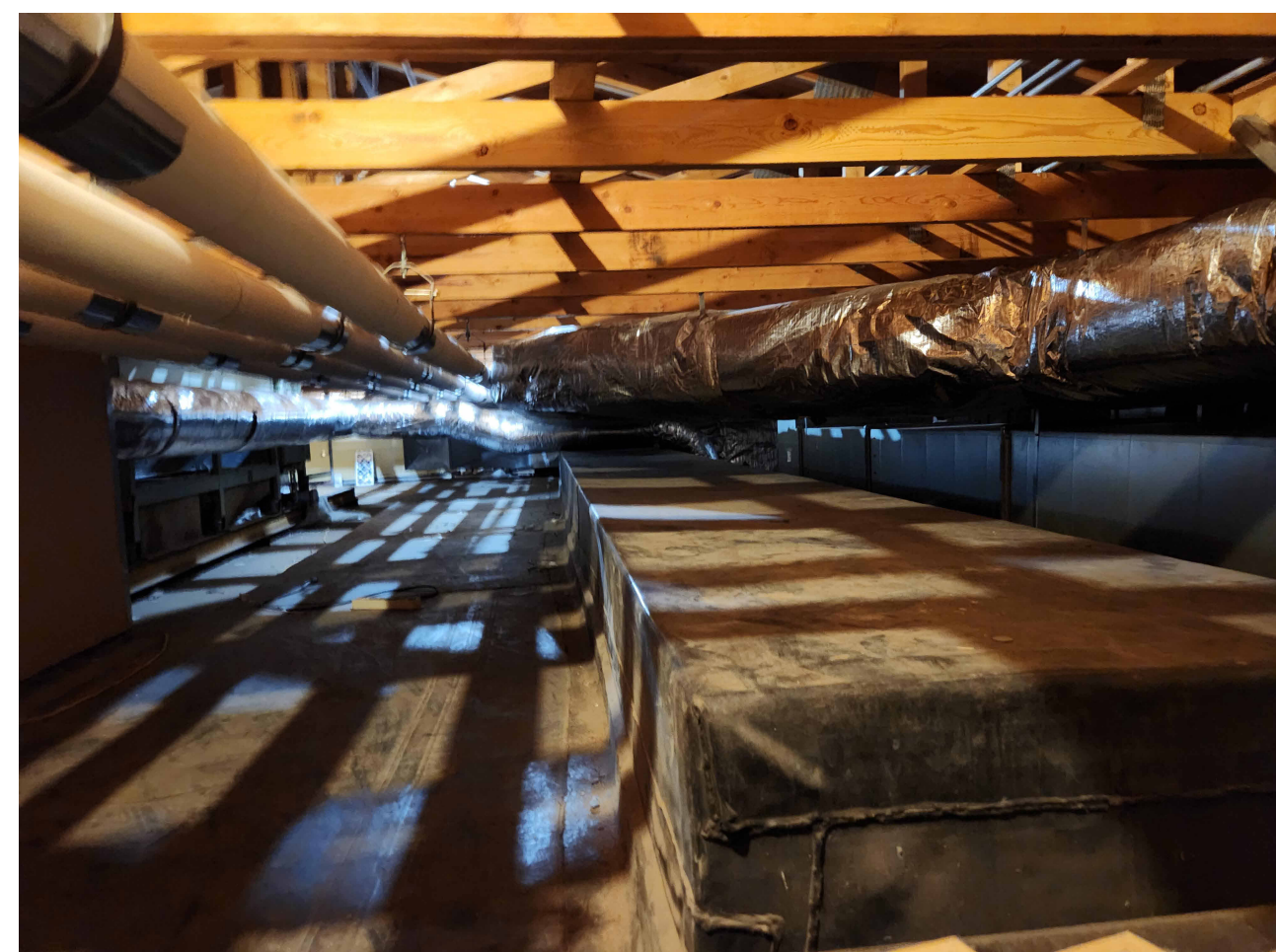
12 ATTIC - HVAC BUMP AT MIDDLE OF ROOM
