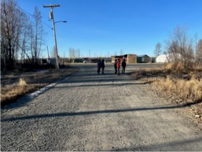
Entrance road where flooding occurs.
