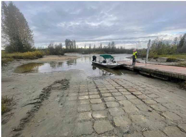
Sediment filled boat launch basin, ramp, and dock.
