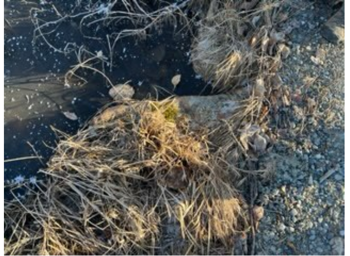
Crushed entry road culvert.
