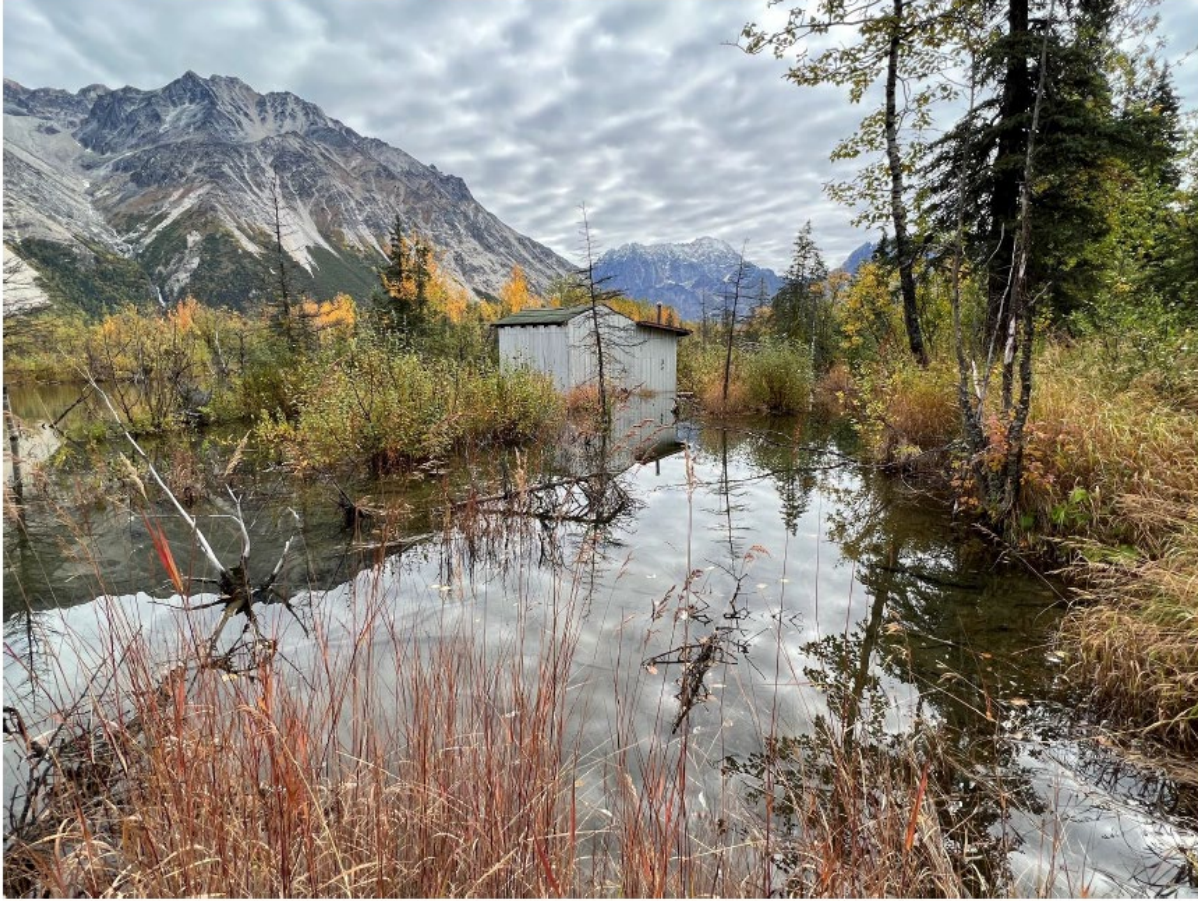
Existing Camp, wood cabin with metal siding under water
