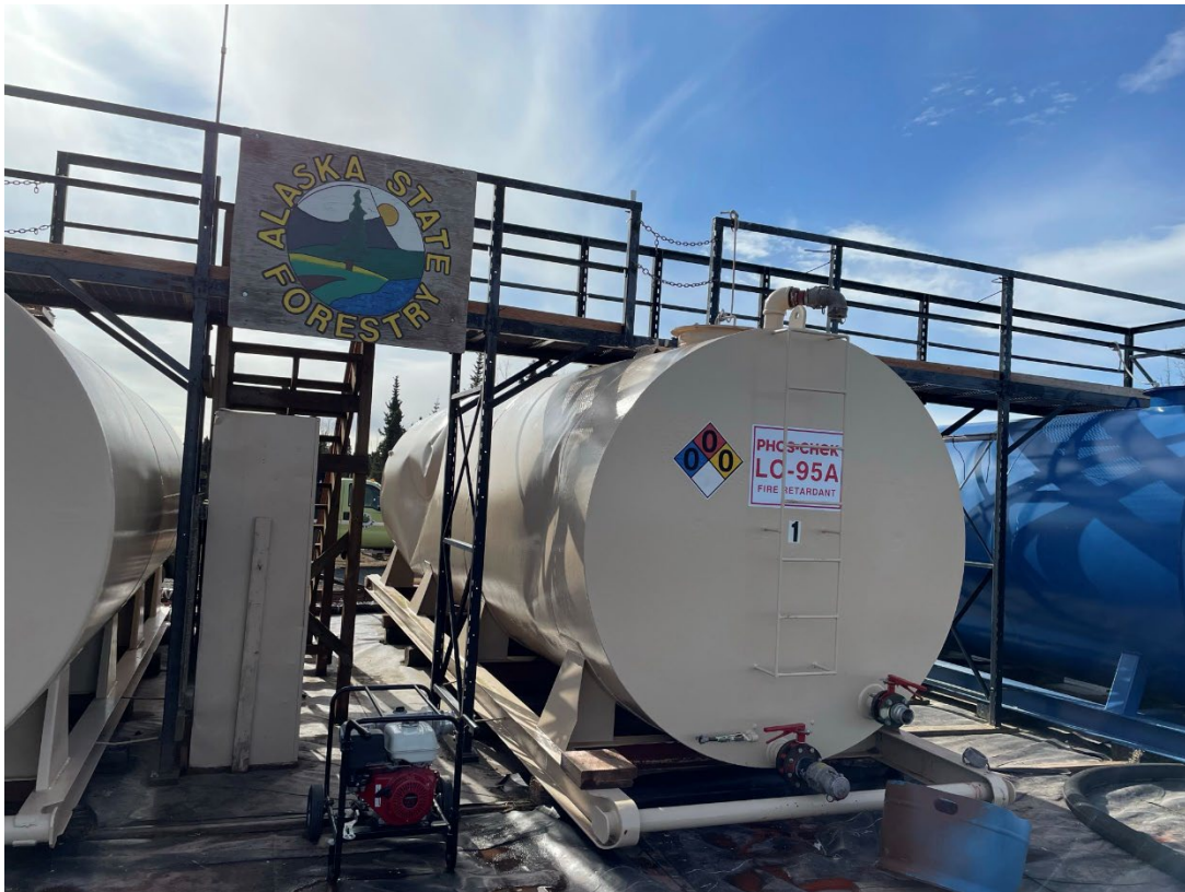
Above: Tank in Kenai that currently requires refurbishment.
