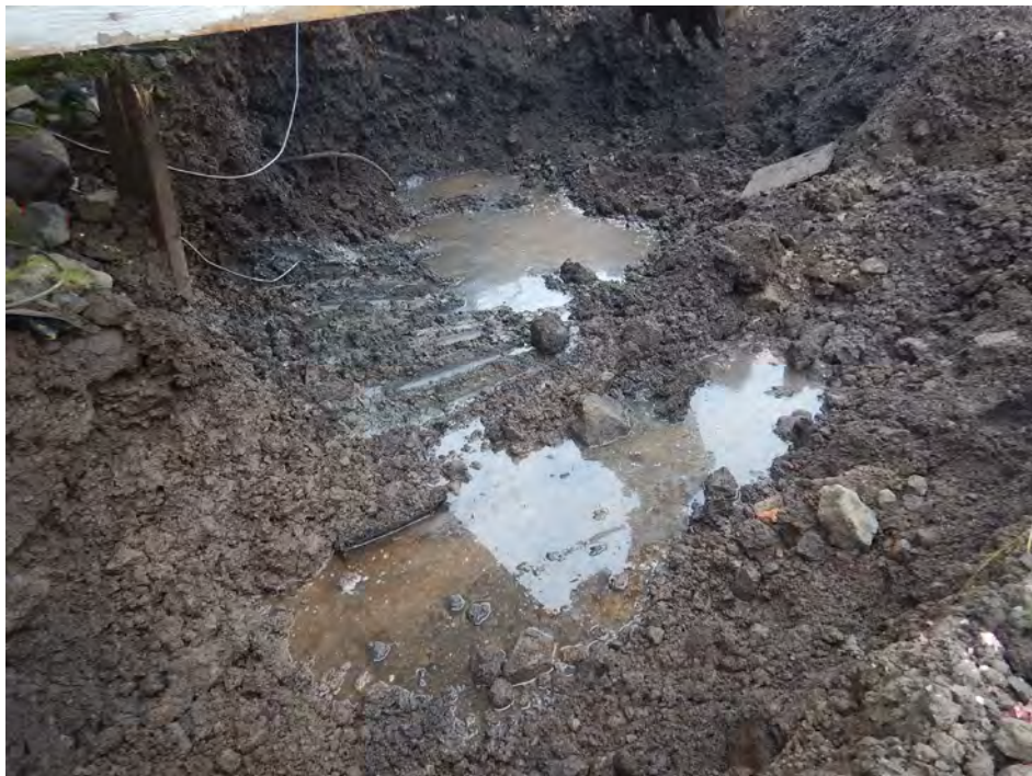
Photograph 6: Water in excavation with POL sheen, view east.
