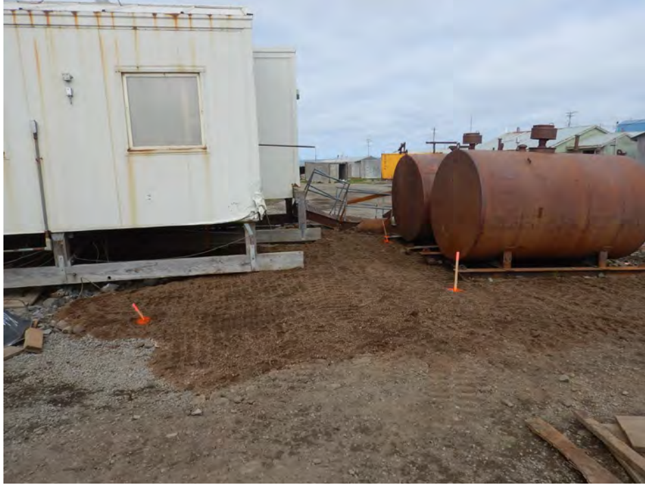
Photograph 13: Recontoured backfilled excavation, tanks moved southwest approximately 10 feet away from road, view northeast.
