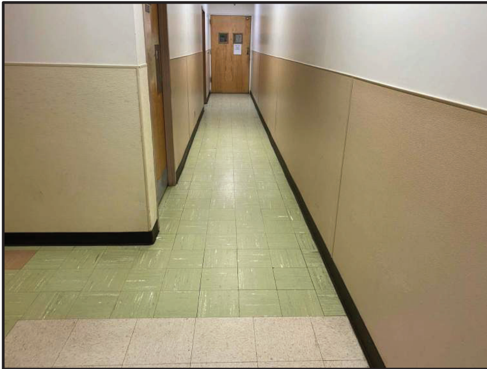
Photo 1: Green 9"x 9" tiles in the employee corridor. Both the tiles and black mastic beneath the tiles are ACM (>1% asbestos). These tiles extend into McKinley hallway and the solariums off that hallway.
