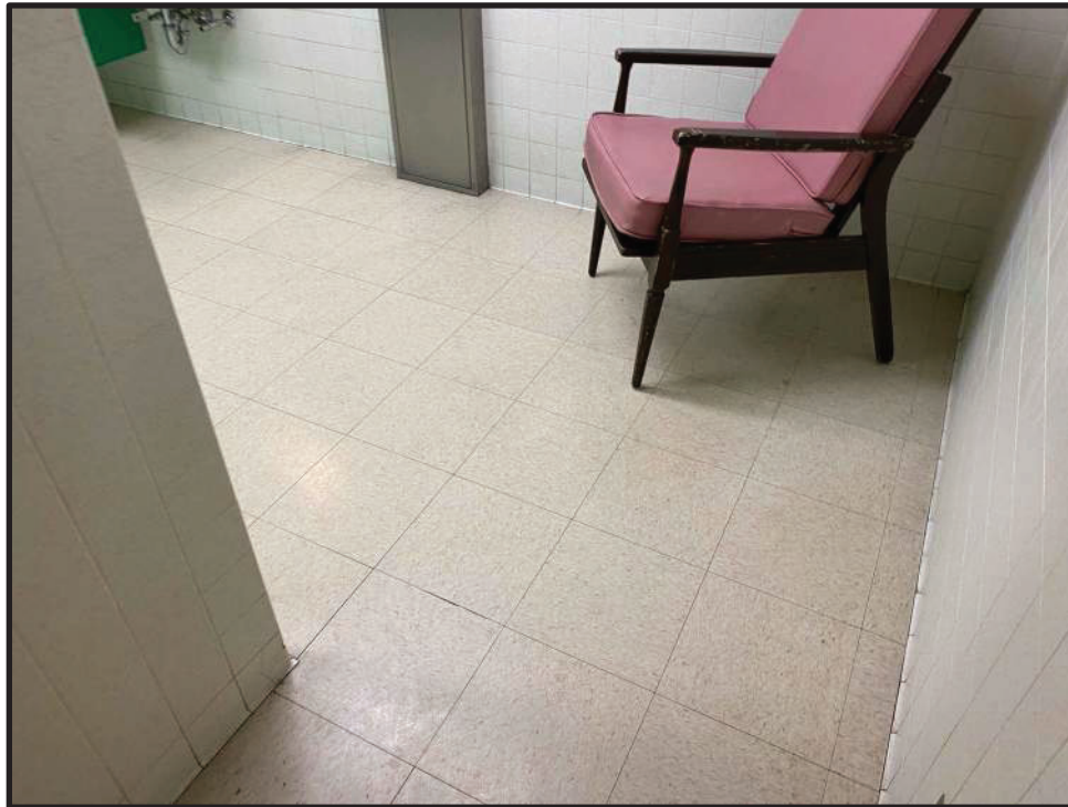
Photo 3: 12x12 vinyl tiles in the men's locker room. Black mastic contained levels of asbestos below 1% and flooring system is recommended to be abated and disposed of as ACM.
