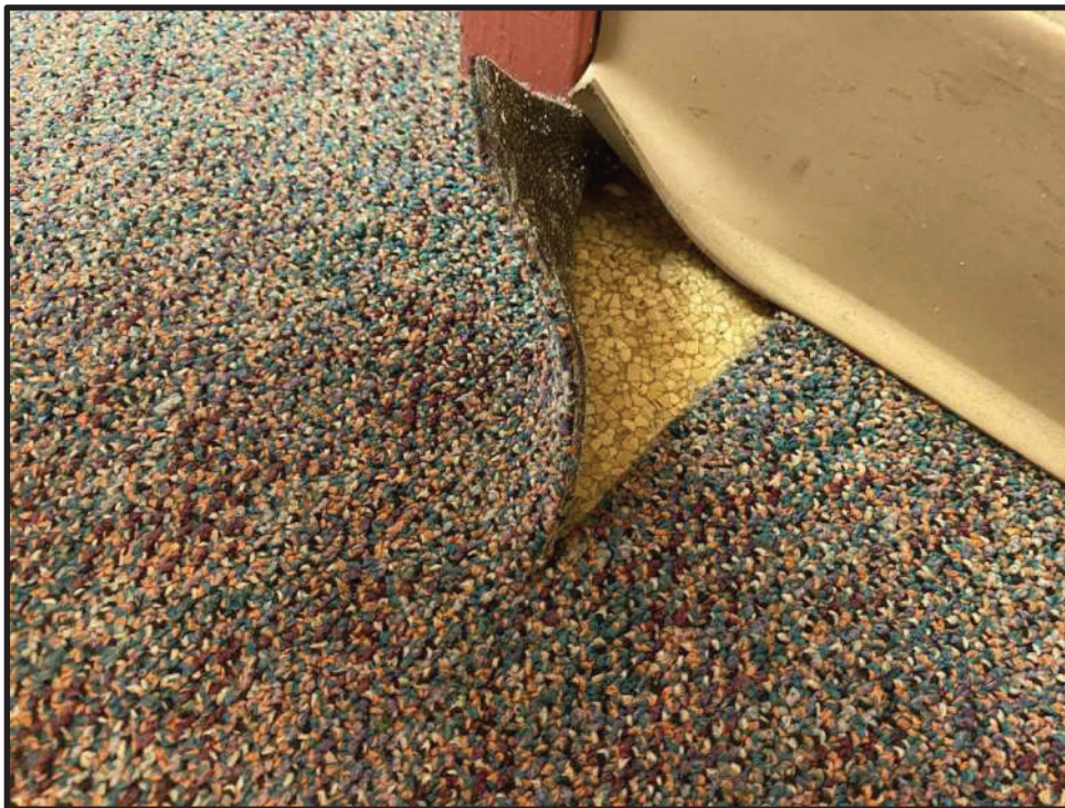
Photo 6: Location of Sample 21. Example of a differing color and style vinyl under self-stick carpeting. Entire floor system is recommended to be abated and disposed of as ACM.
