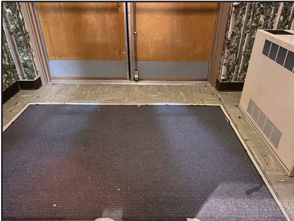
Photo 2: Multi-colored tiles sampled in the entryway at the end of McKinley Hall had asbestos in black mastic below 1% and flooring system is recommended to be abated and disposed of as ACM.
