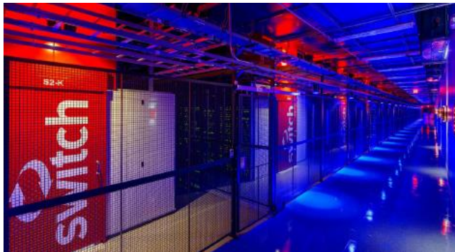
Switch, Inc., IFM
