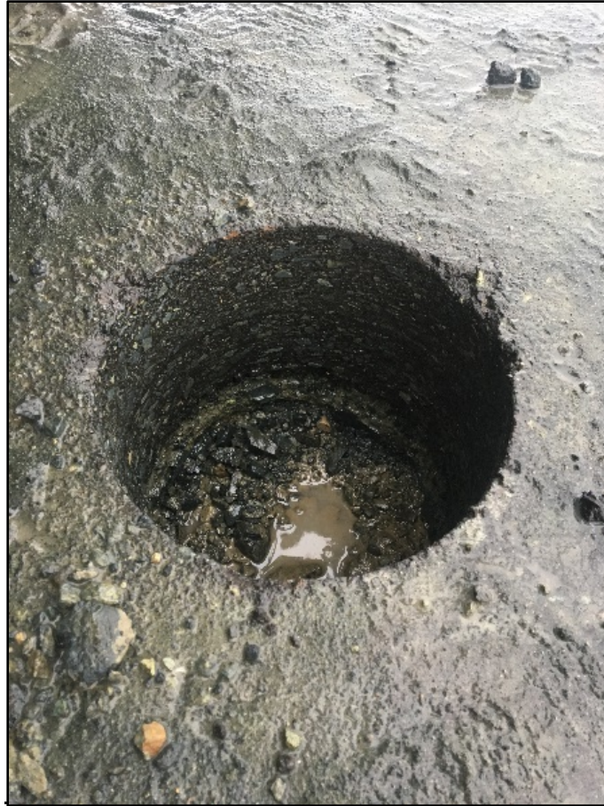
Photo 8: TH19-2104 after coring 8" of asphalt and driving the first SPT 8-32" through the base. Base consists of poorly-graded sub-angular gravels (GP).
