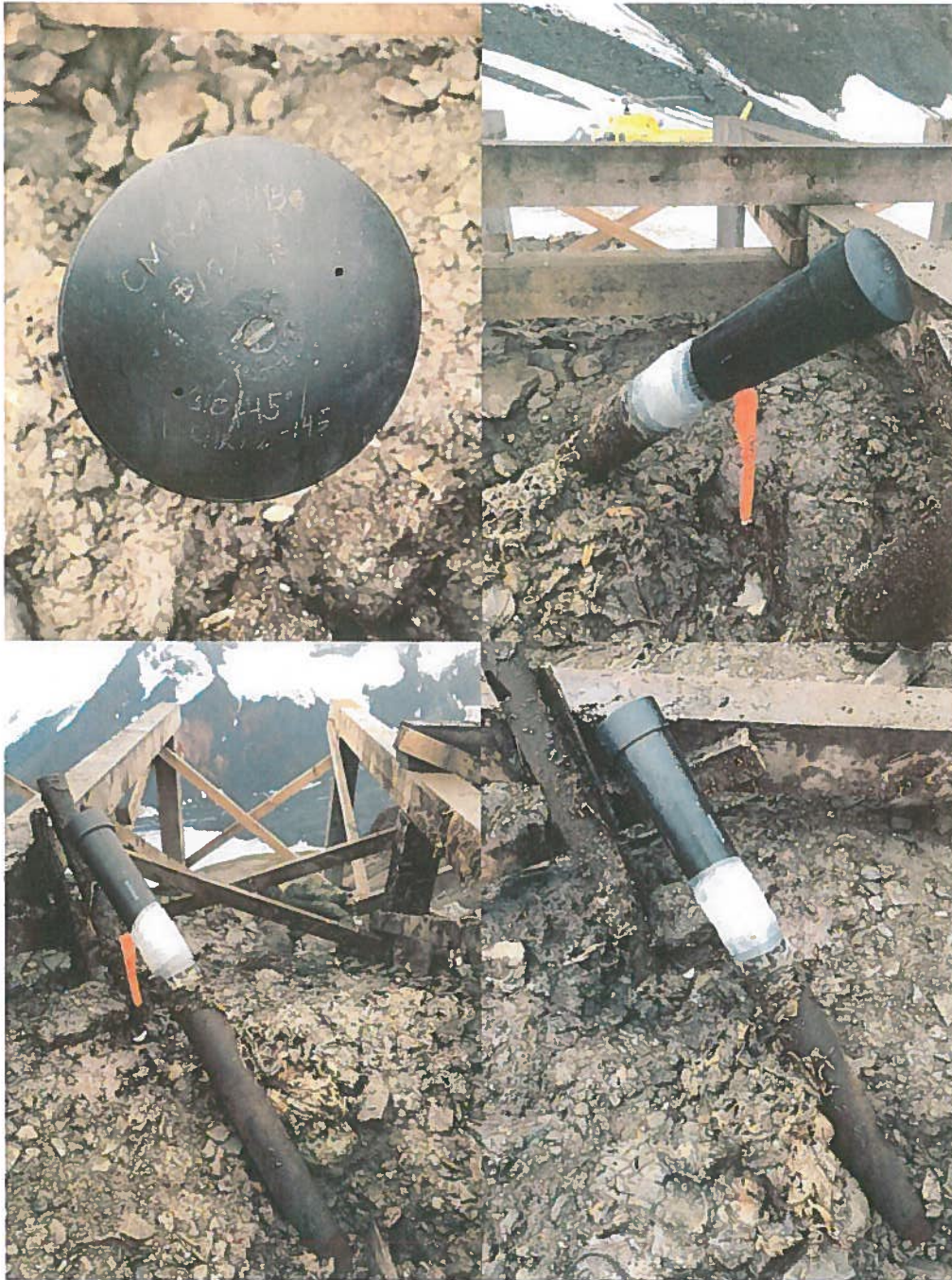
Photo 4: Paradise City Pad diamond drill hole CMR22-145 is capped. Mixed slotted and unslotted PVC was installed to support potential future geophysical surveys.
