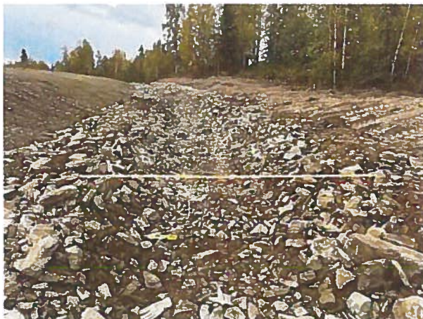
Photo 17: 20220916 upper portion of channel
