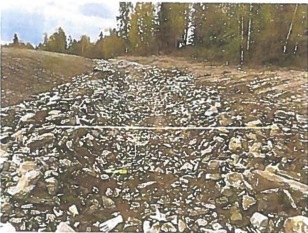
Photo 17: 20220916 upper portion of channel
