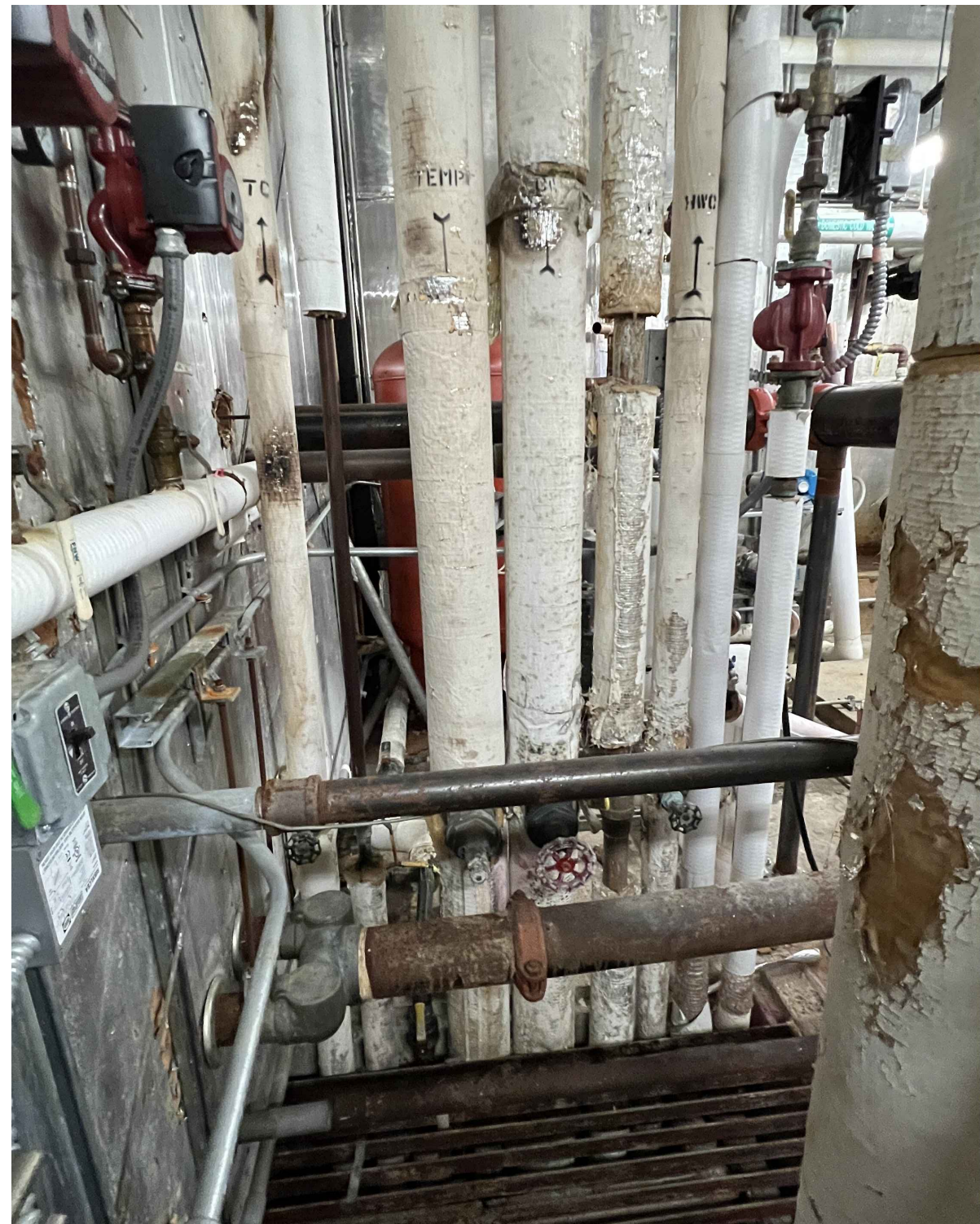
A EXHIBIT PHOTO - MECH. ROOM
