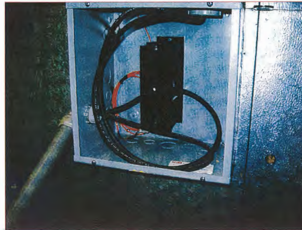
3 E19A NTS ENCLOSURE PHOTOGRAPH
