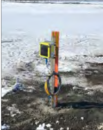
Photograph 28. Example of installed thermistor well, DTC, and datalogger.
