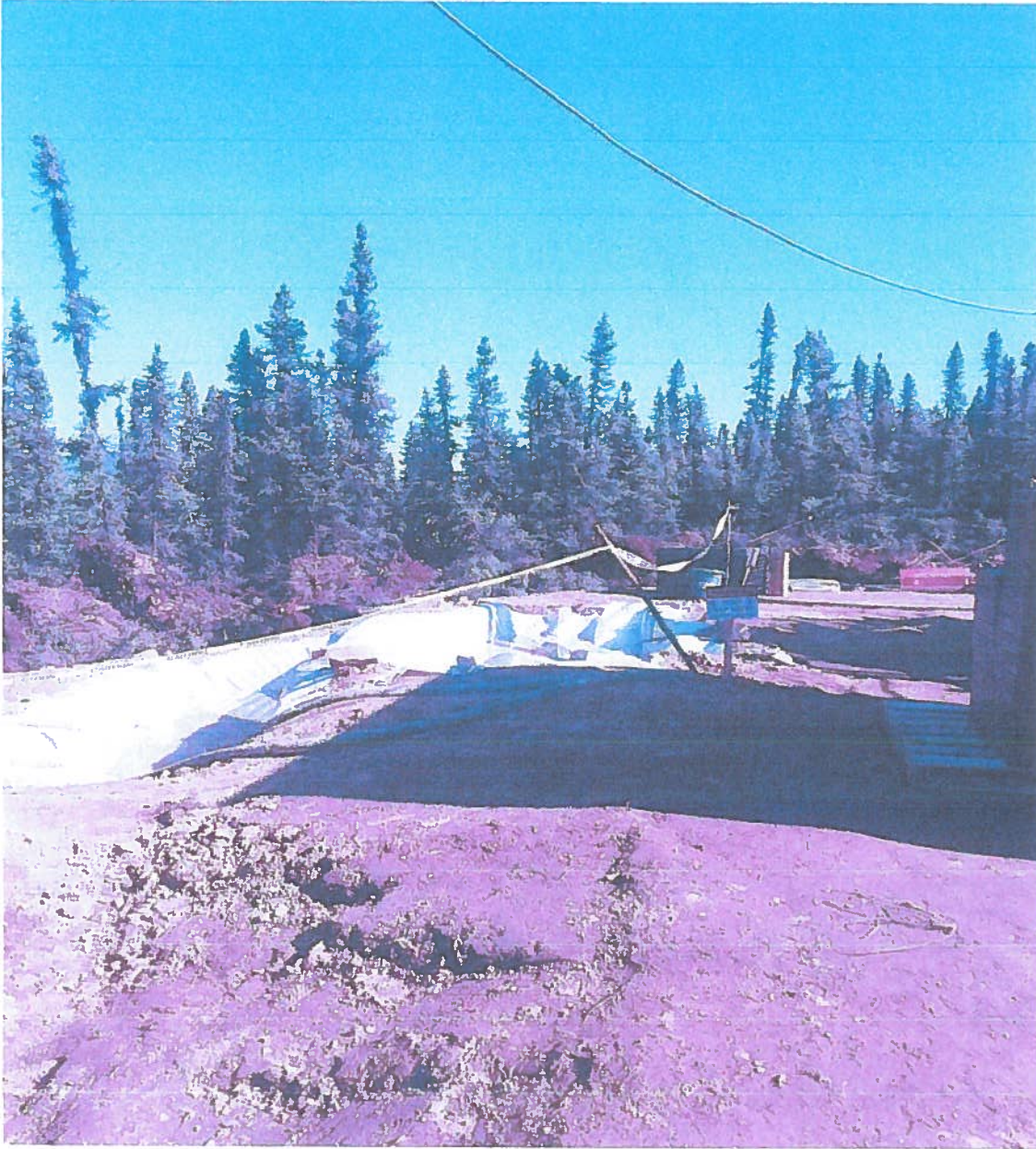
Photo showing the completed sump at Drill pad #1 from the 2020 Amanita drill program.
