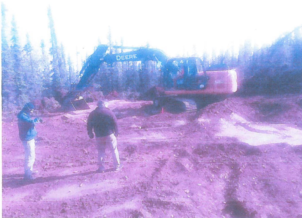
Photo showing drill pad construction from the 2020 exploration drill program on the Amanita claim block. This is representative of the type of pad construction to be utilized for the 2021-2025 Plan of Operations.
