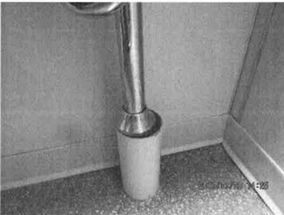
Figure 12 Penetration misalignment under sink in Crew Head
