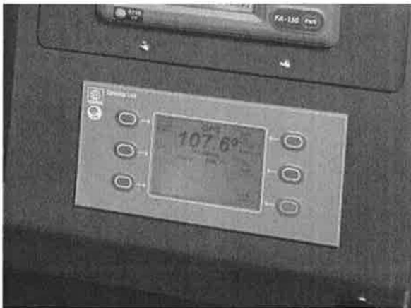
Figure 51 Gyro Compass control in Pilothouse
