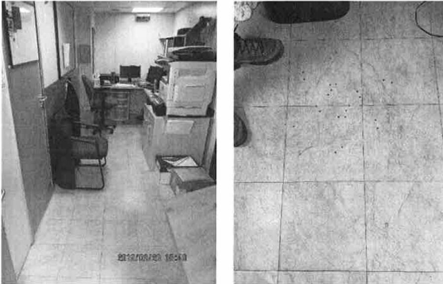
Figure 25 Passenger Service Office (left) with holes in deck covering (right)
