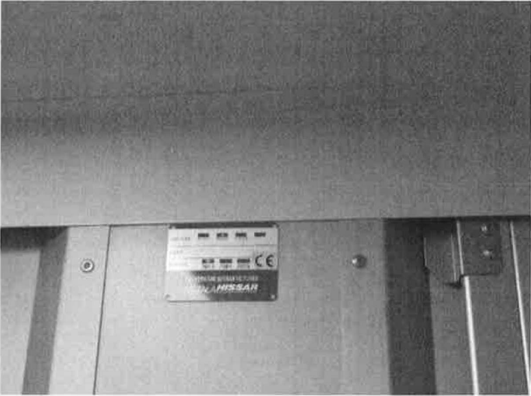
Figure 45 Minor spots in overhead of Passenger Elevator
