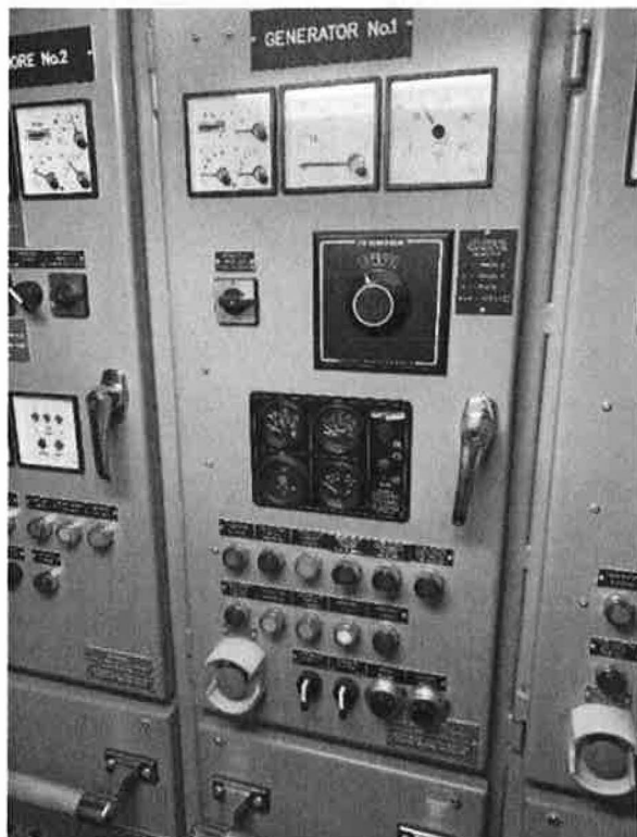
Figure 35 Generator 1 Switchboard in the starboard Switchboard Room
