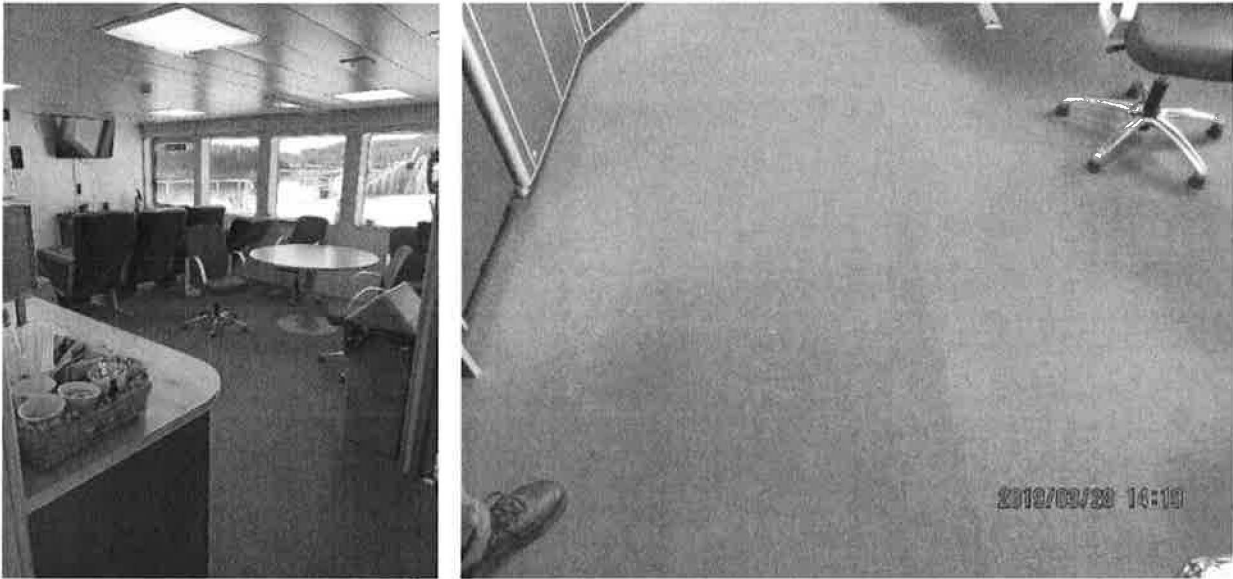
Figure 9 Crew Day Room (left) with minor stains and deformation on carpet (right)
