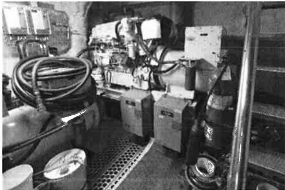
Figure 23 Generator 4 in Port Engine Room
