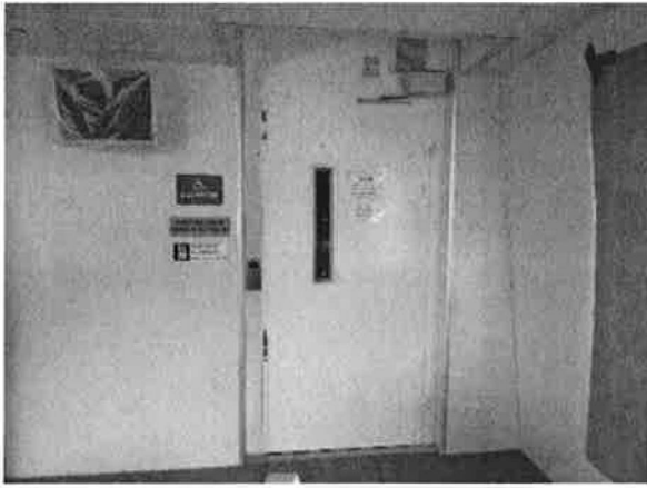
Figure 27 Passenger elevator on Passenger Deck
