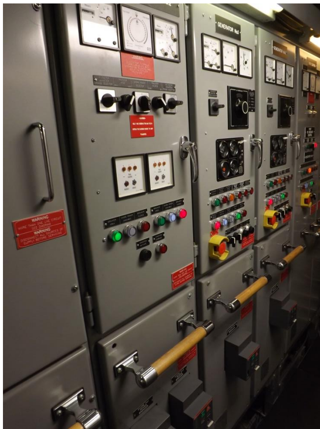
FVF Fairweather Starboard Switchboard Room Panels
