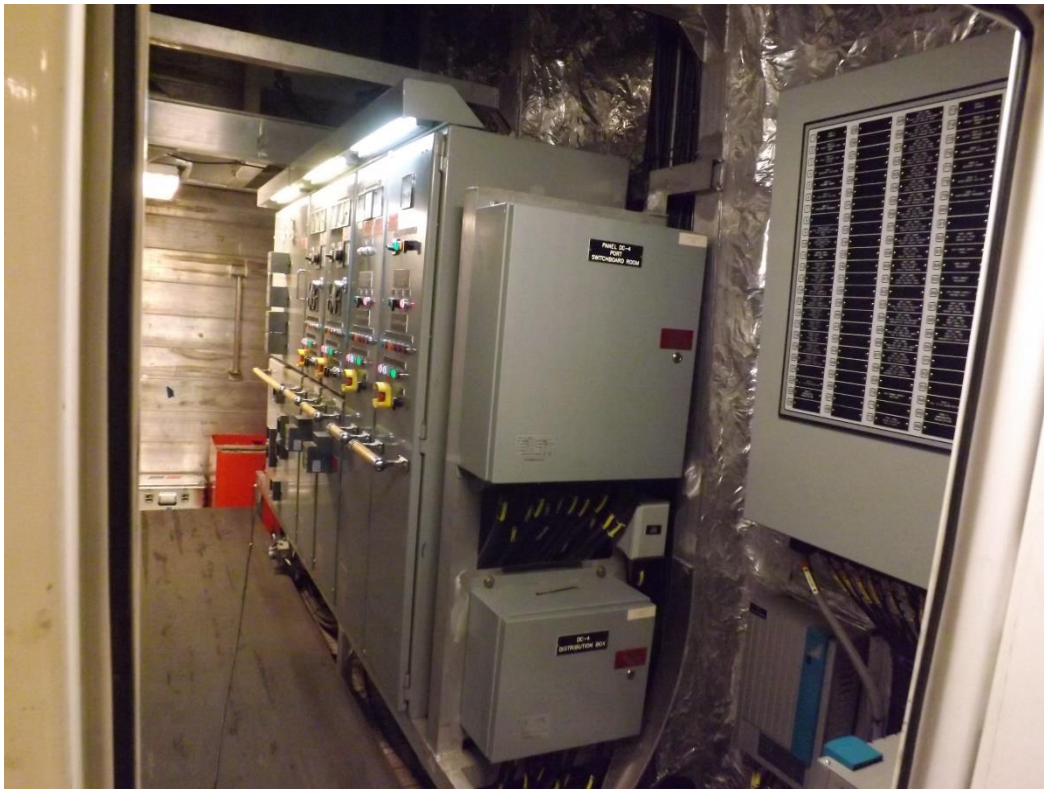
FVF Chenega Port Switchboard Room
