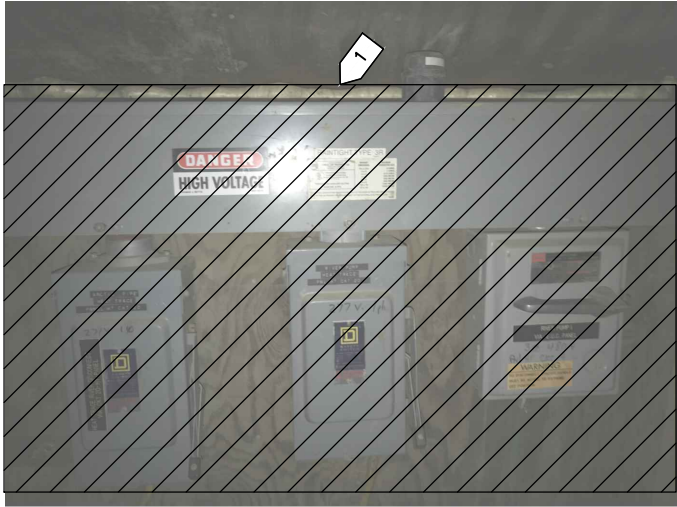
EXISTING RAW WATER PUMP HOUSE ELECTRICAL PANELS
