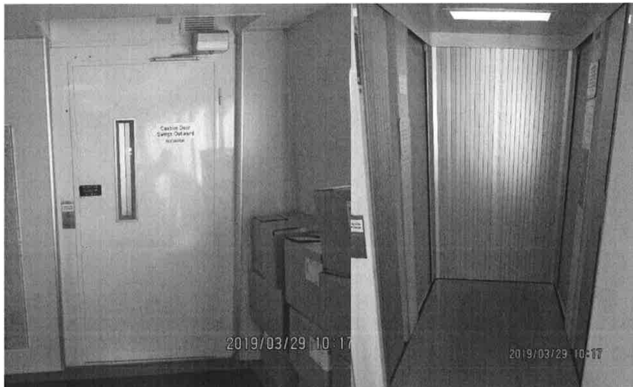
Figure 44 Passenger elevator on Passenger Deck
