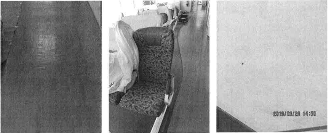
Figure 15 Bubbling in faux wood flooring (left), replacement seats (middle), and minor dents in bulkhead (right) in Forward Observation Lounge
