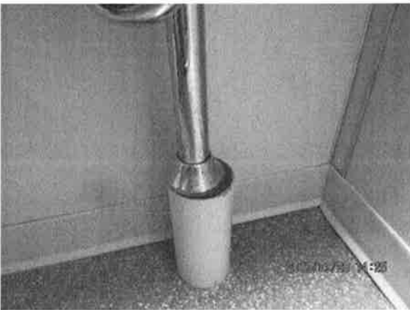
Figure 12 Penetration misalignment under sink in Crew Head
