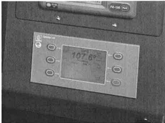
Figure 51 Gyro Compass control in Pilothouse
