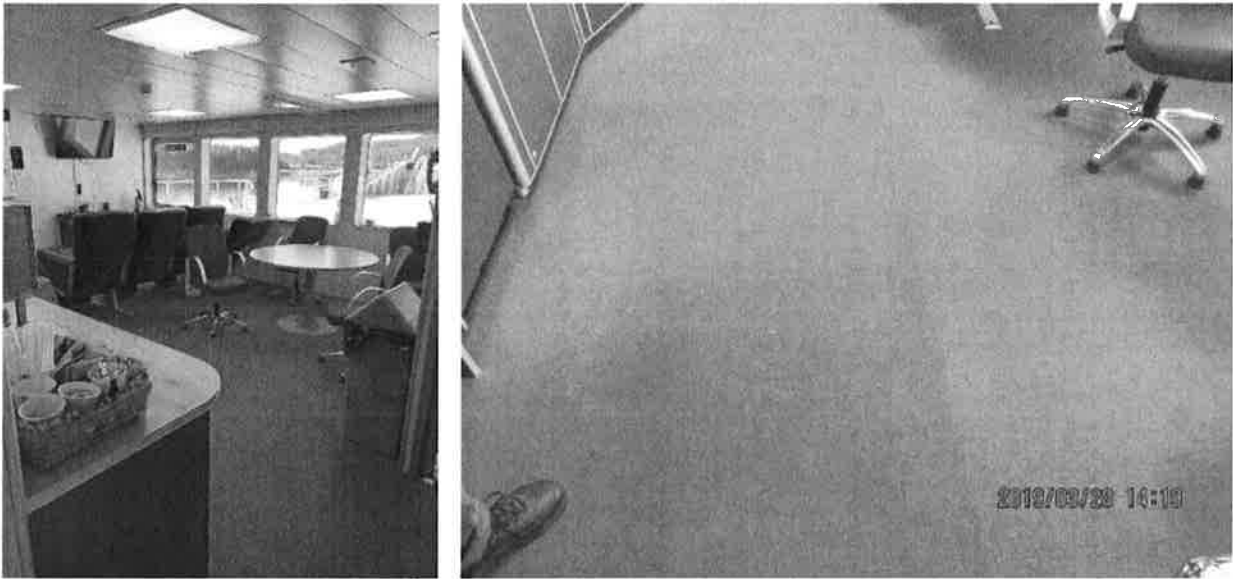
Figure 9 Crew Day Room (left) with minor stains and deformation on carpet (right)
