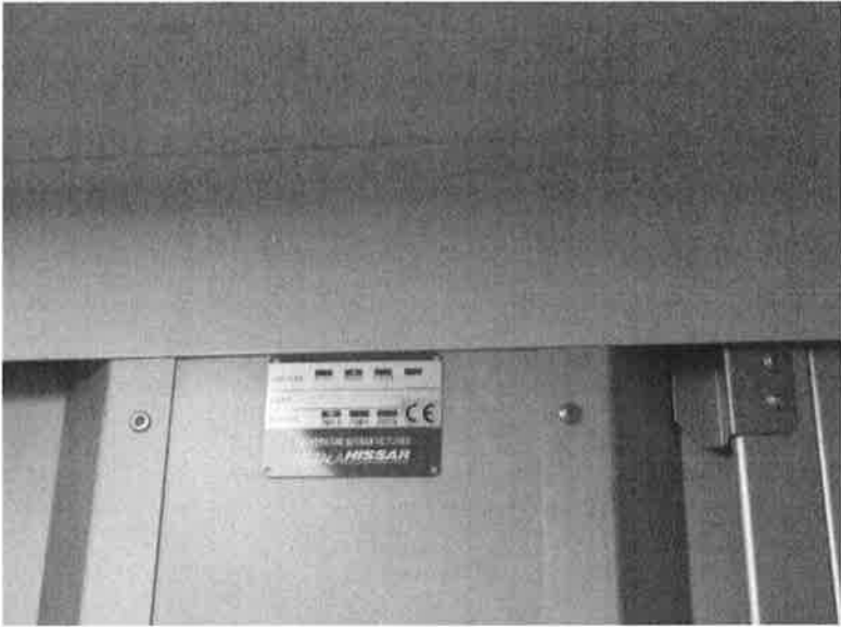
Figure 45 Minor spots in overhead of Passenger Elevator
