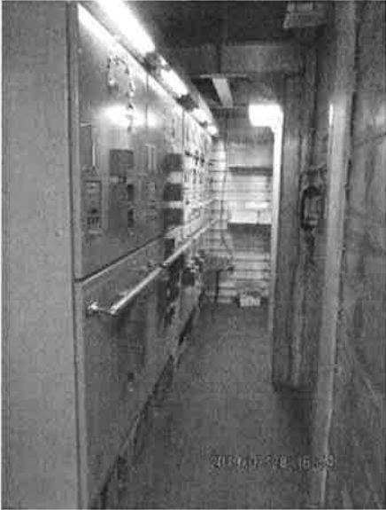
Figure 33 Starboard Switch Room on Vehicle Deck
