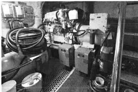
Figure 23 Generator 4 in Port Engine Room
