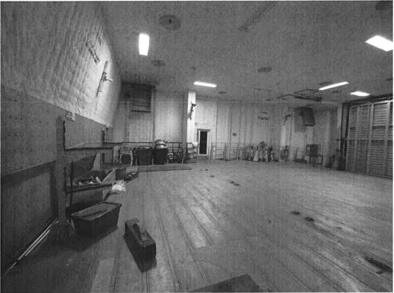
Figure 1 Vehicle deck view looking forward towards side door; insulation visible at sides and overhead
