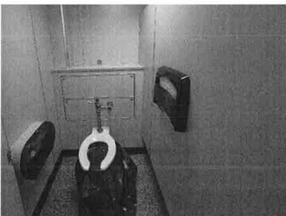
Figure 14 Appliance discoloration in Passenger Head on Passenger Deck
