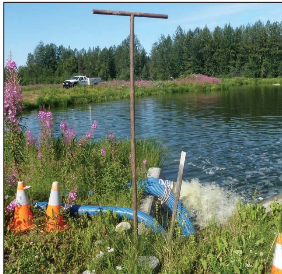
Figure 2-6: Gasoline-Powered Pumps Used to Assist with Aeration During Summer 2016
