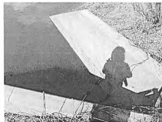
Cell 1 and 2 overflow pipe
