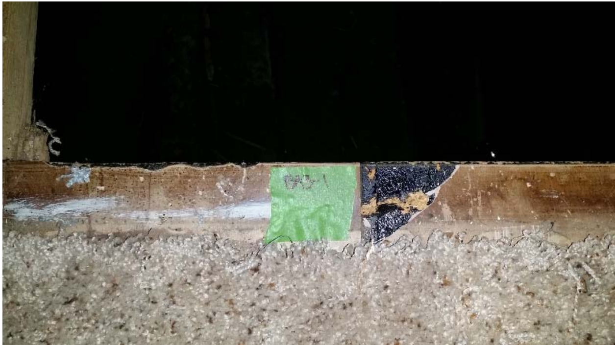
Photo 7: The dark brown vinyl flooring under the carpet in Bedroom 3 contained 3% Chrysotile asbestos.
