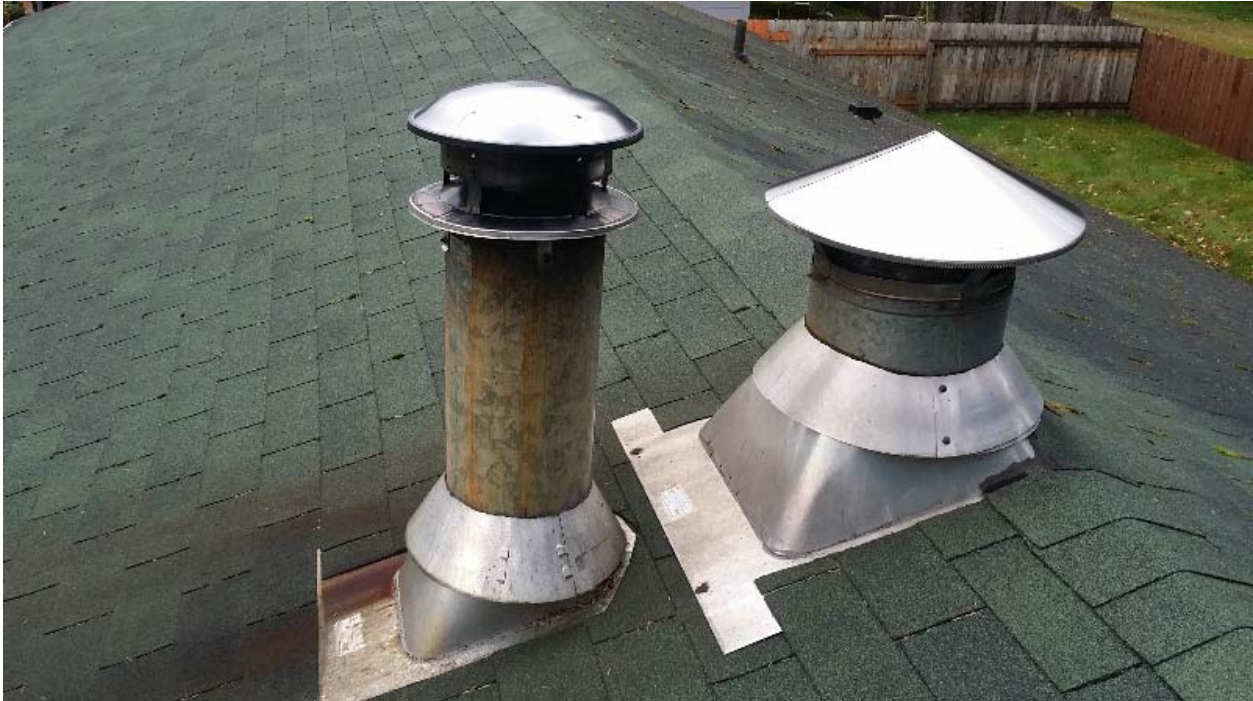
Photo 4: Both chimney pipes had plaques identifying them as asbestos-containing pipes and are considered Non-Friable Category II ACM.
