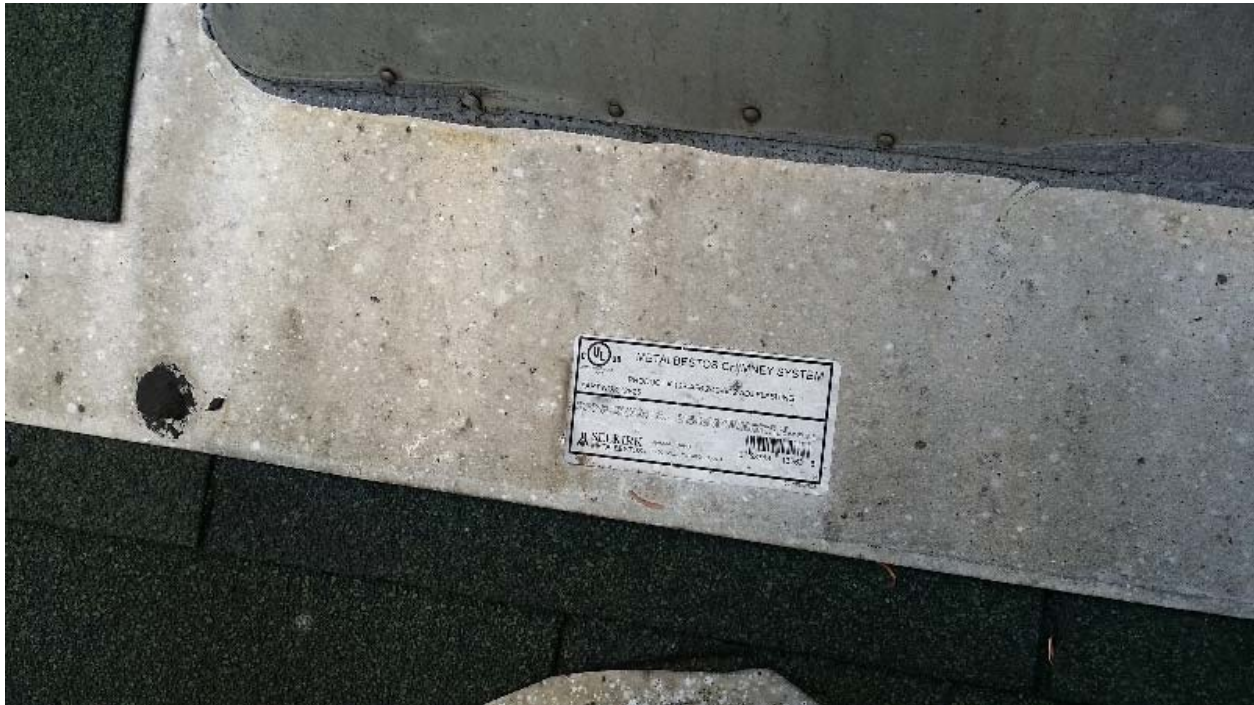
Photo 5: NORTECH did not collect a sample of the chimney pipe segments as both chimneys contain labels indicating they contain asbestos.
