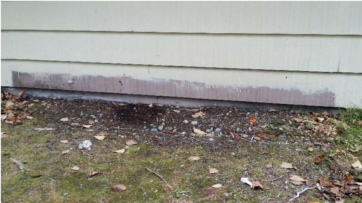
Photo 3: The area of purple-brown paint with a lead concentration of 1.6 is located near the sliding back door.
