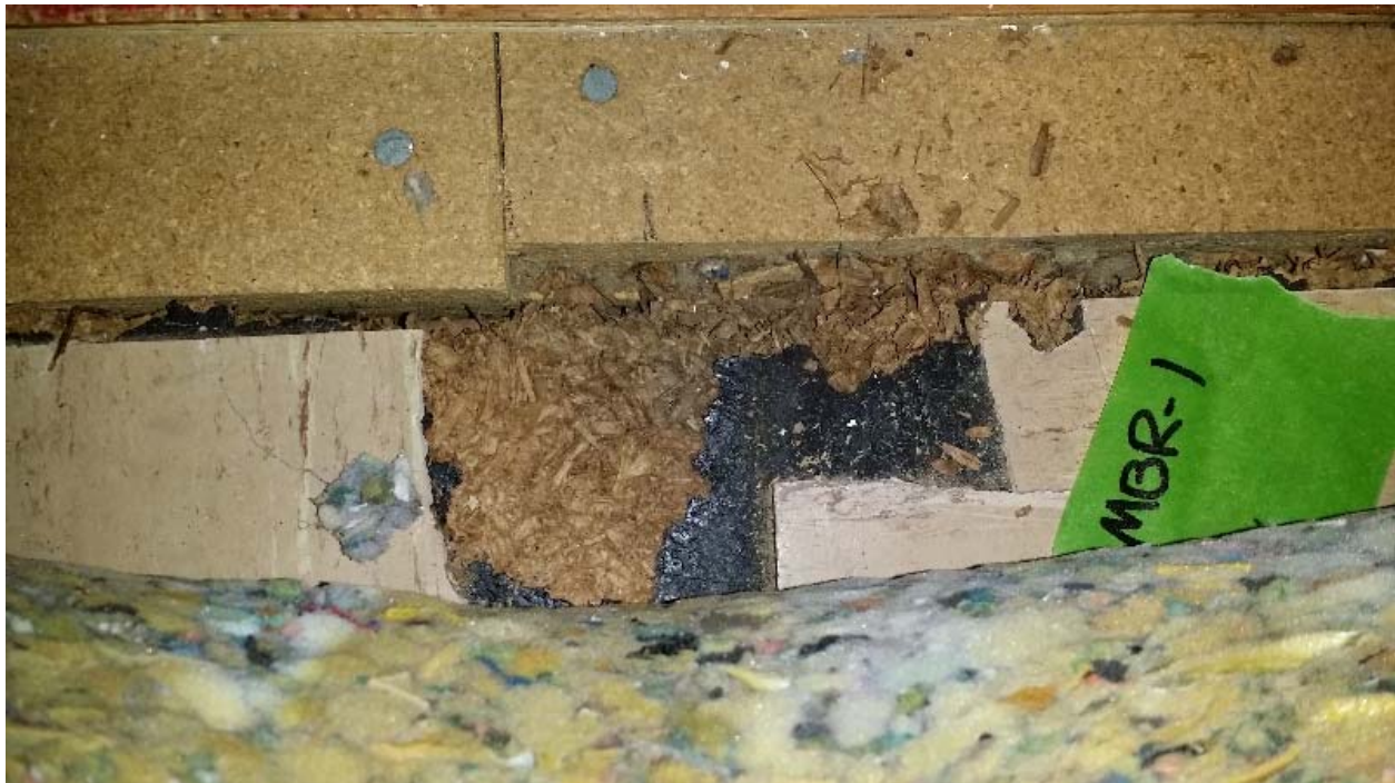
Photo 6: The light brown vinyl flooring under the carpet in the Master Bedroom contained 4% Chrysotile asbestos.
