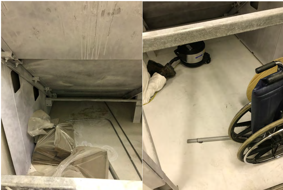
Photos 54 and 55: TG/E – Floor in the FRRR before cleaning (left) and clean FRRR floor after HEPA vacuuming (right).
