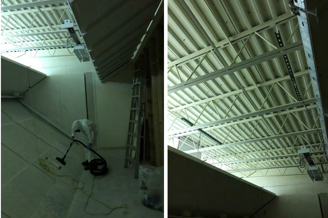
Photos 52 and 53: TG/E – Fully suited worker cleaning in the FRRR (left) and view of overhead rafters in the FRRR (right).
