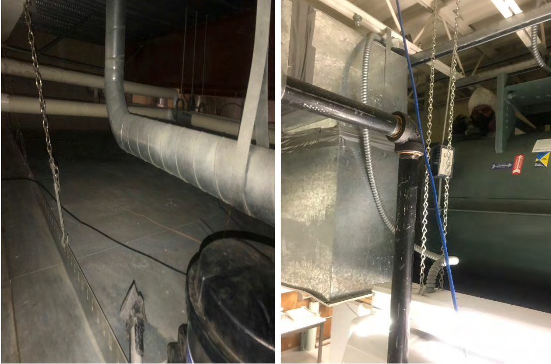
Photos 37 and 38: SR – Attic/duct area before cleaning (left) and worker in full PPE cleaning the attic area (right).
