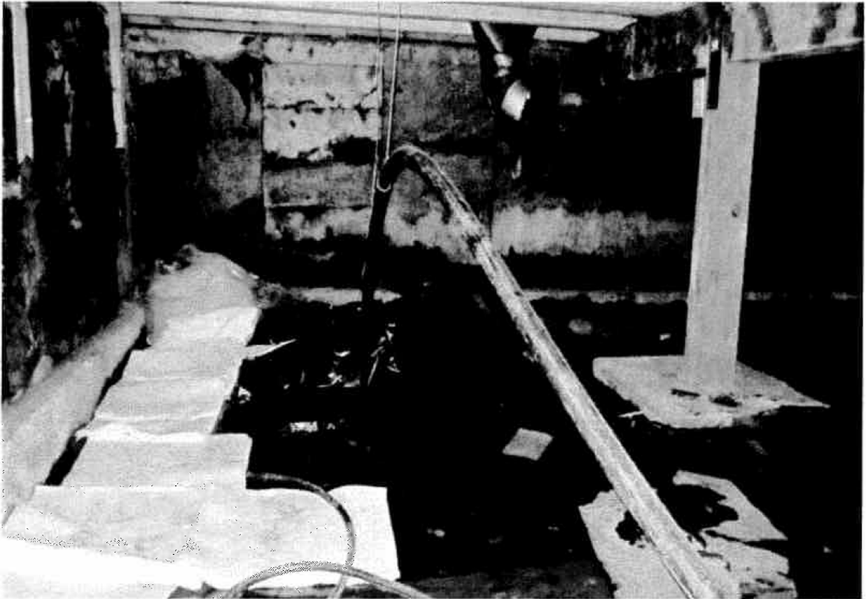
Figure 3: Crawlspace near the sump at the time of fuel release. Photo copied from “RE: Fuel Oil Spill Assessment and Remedial Work Plan Report Letter,” dated February 22, 2012, prepared by Nortech Inc.
